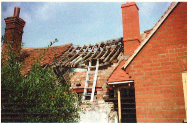
Plate 29: Exposed roof structure of back room, with New extension to the south (C A Cheal)
