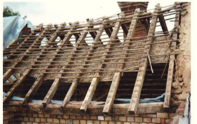
Plate 30: Detail of east side of exposed roof structure over front room (C A Cheal)
