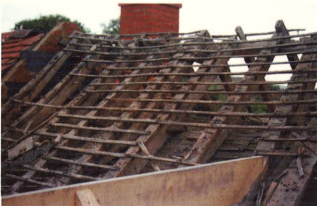
Plate 31: Detail of east side of exposed roof structure Over back room (C A Cheal)
