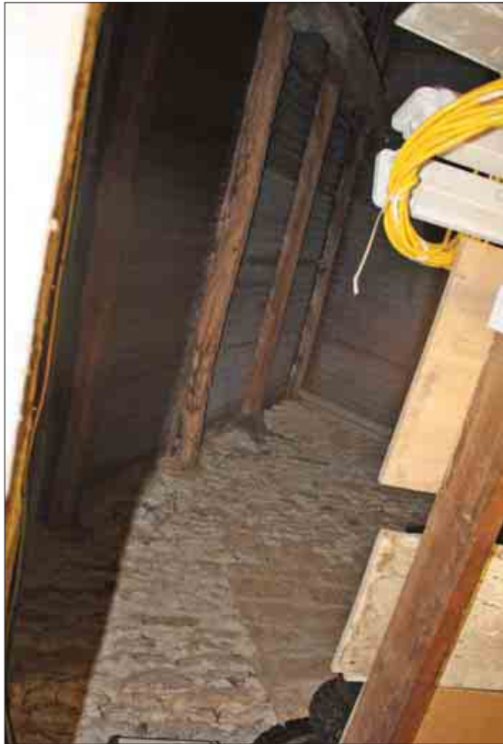
Plate 72: Blocked opening on southern wall at first floor level as viewed from G2, Building 1
