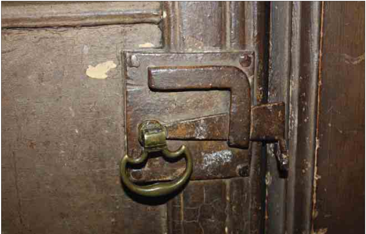
Plate 45: Detail of late 18th/early 19th century spring latch on door from F5b to attic
