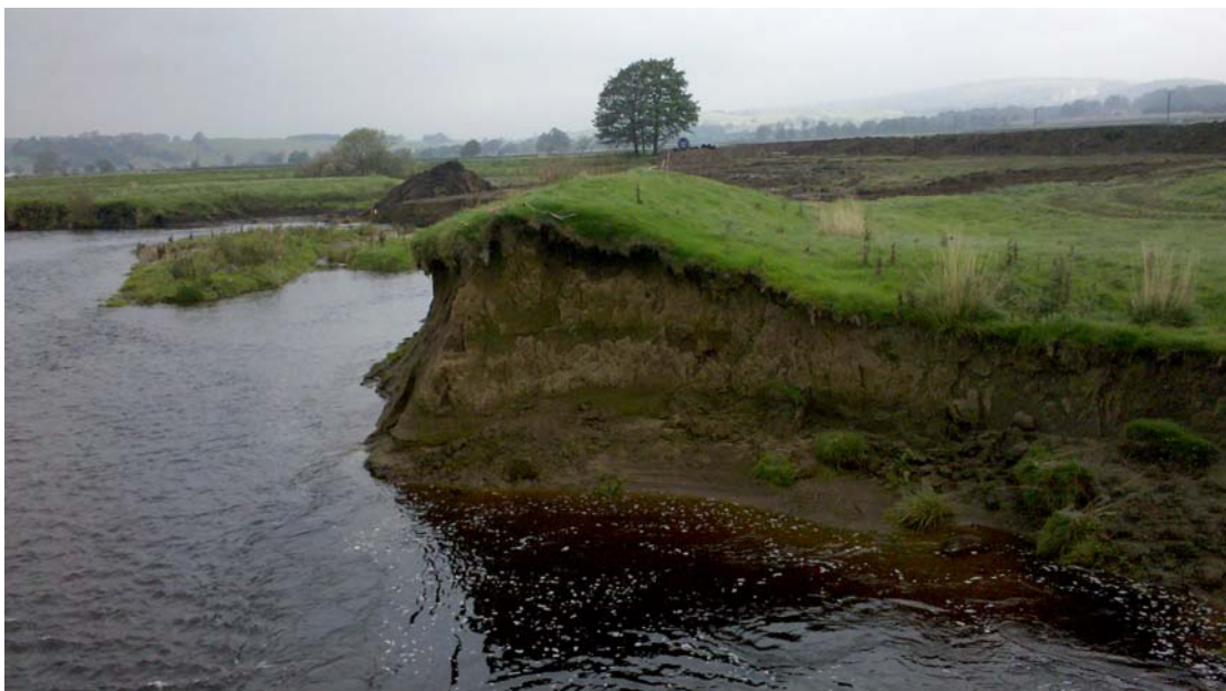
Plate 2: The result of severe riverine erosion, which has truncated a portion of embankment 101=105 , looking north
