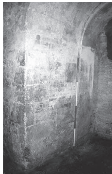
Plate 2.16 Vault 6, details of the stone quoins of the archway to the tower
