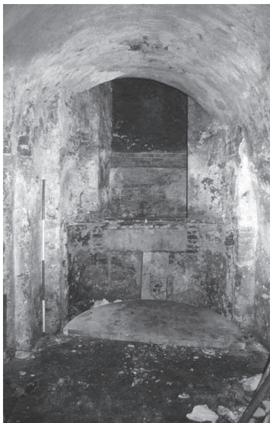
Plate 2.10 Vault 3 looking E, showing slightly skewed window recess with private tomb 3500 beneath. The semi-circular lid of the tomb is lying on the floor
