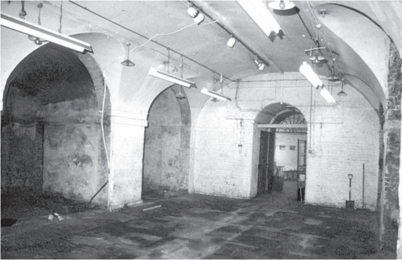
Plate 2.1 Main central vault looking S. The doorway leads through to the E-W vault and the main stairs.
