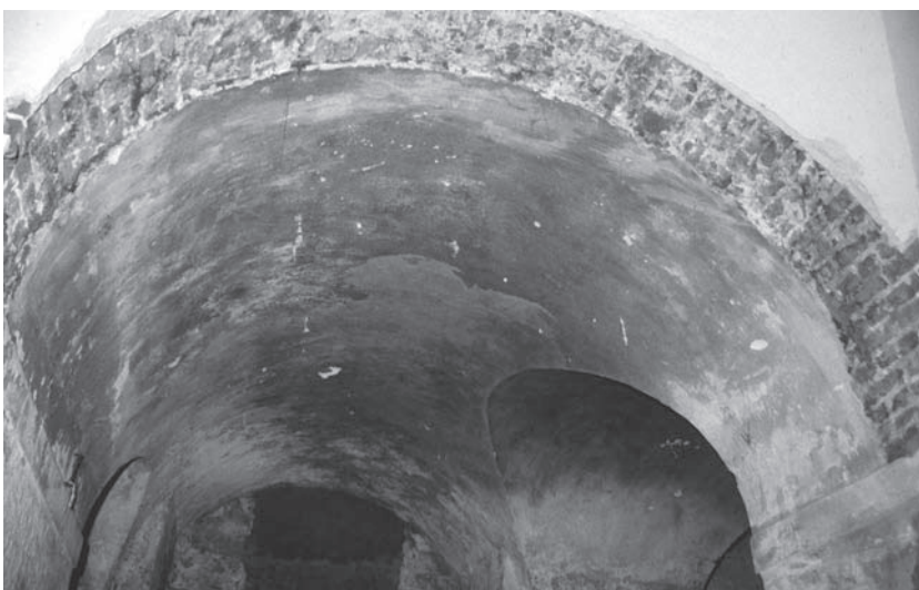
Plate 2.13 Vault 5 showing exposed brickwork where the 19th-century sealing wall has been removed
