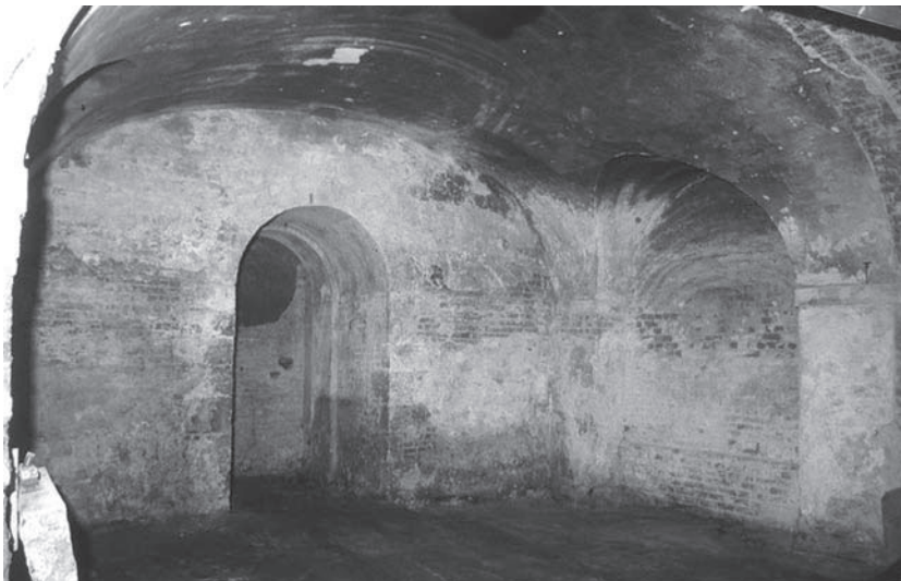
Plate 2.15 Vault 6 looking W. The block doorway to the base of the tower is clear
