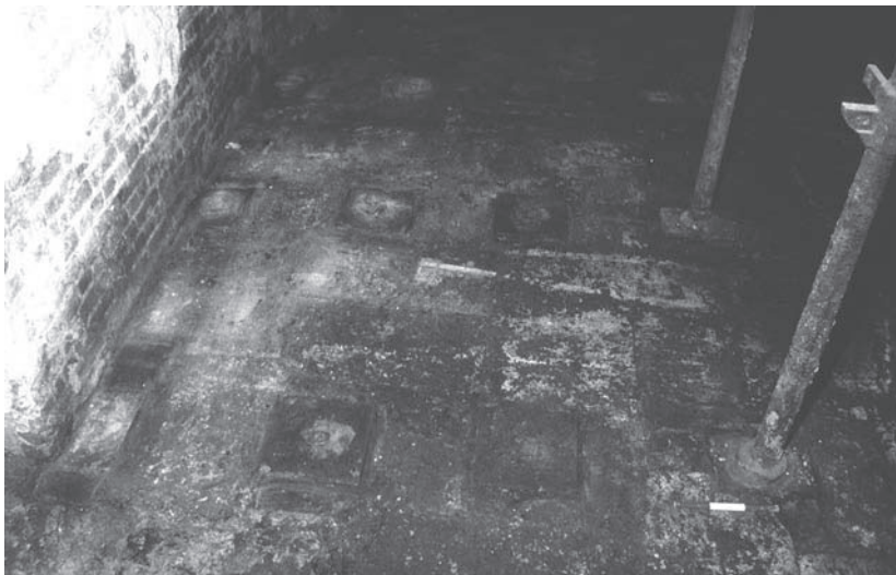
Plate 2.6 Stone post bases and extant cast iron posts for shelving in Vault 1
