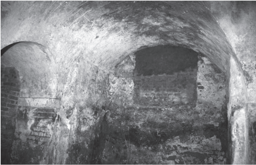
Plate 2.14 Vault 5 looking W, showing square end of vault and blocked window. To the left is the block archway to Vault 4. To the right the fillet or buttress in front of the arch spring can be seen clearly
