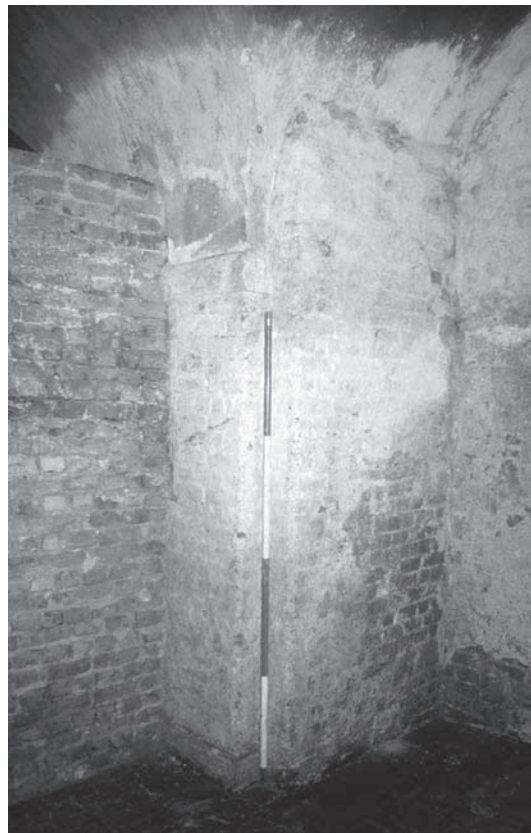
Plate 2.8 Vault 2 looking N, showing to the left the brick blocking of the opening through to Vault 1
