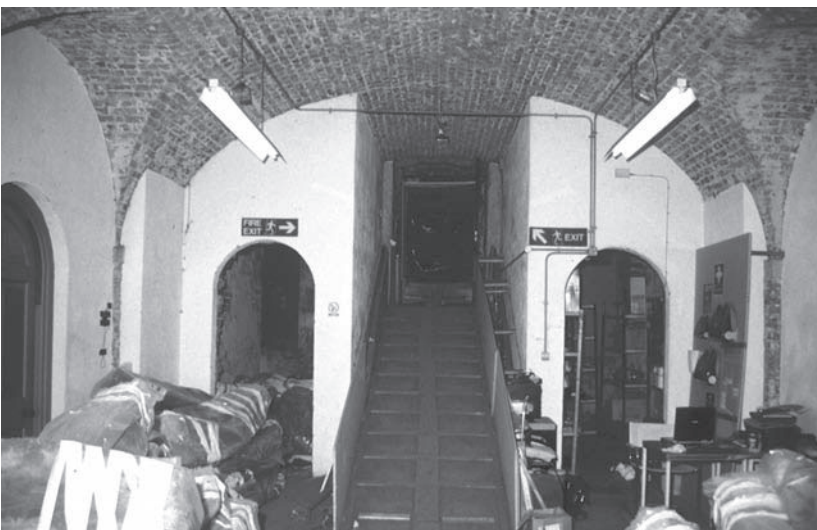
Plate 2.3 Central vault, N end, showing inserted modern stairs with Vault 7 to the left. To either side of the main vault, the fillets or buttresses in front of the main arch springs can be seen clearly.
