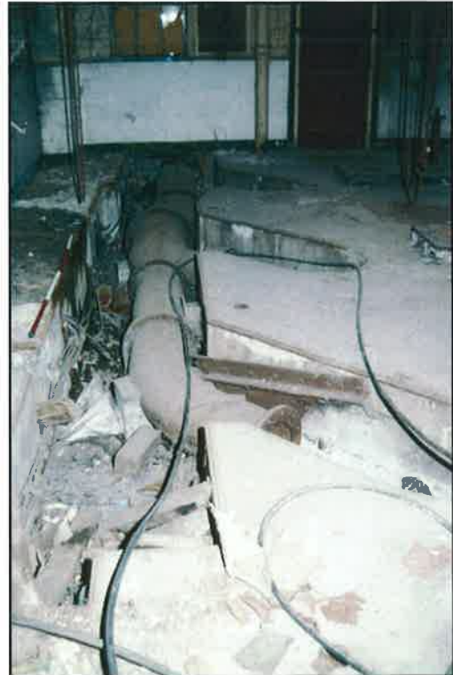
Plate 37: Internal east view of iron pipes within Drainage Pumping Station no. 2
