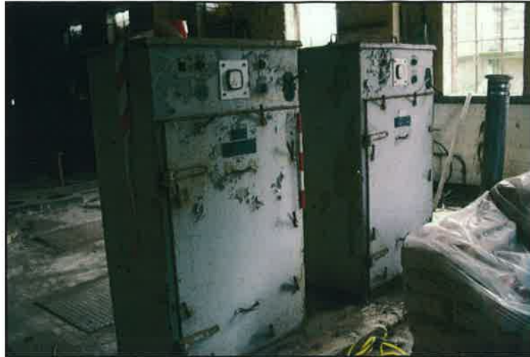
Plate 38: Internal east view of controls boxes within Drainage Pumping Station no. 2
