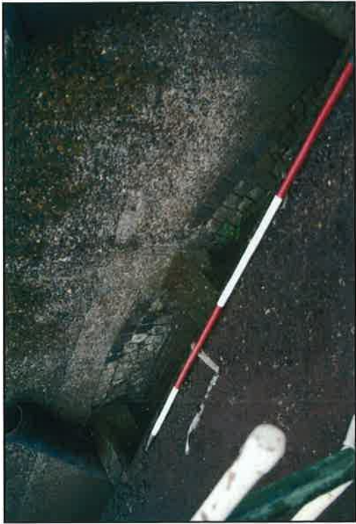
Plate 18: North-east view of blocked precipitation lane arch at east termination of re-aeration lanes
