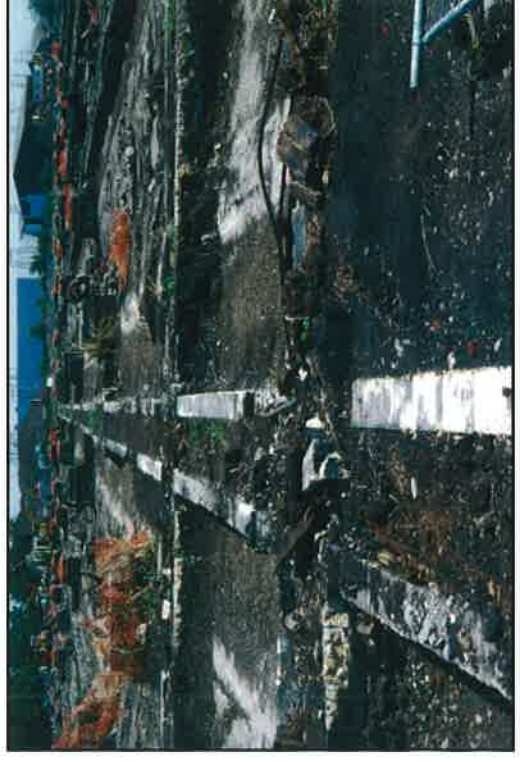
Plate 16: East view depicting brick troughs above precipitation lanes (taken during demolition works)
