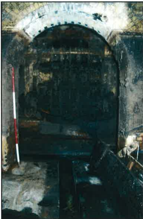
Plate 11: Penstock at south-west termination of precipitation lane
