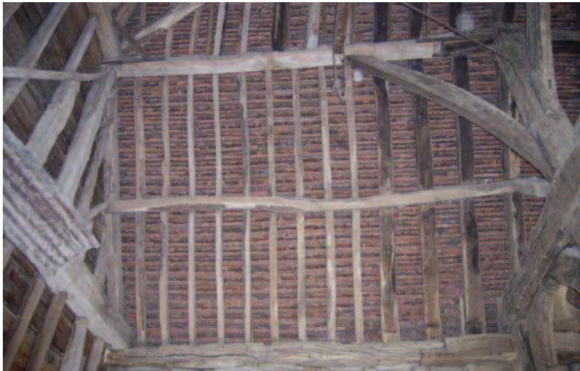
Plate 14: Roof at W end. Rafters to left secondary. Primary smoke blackened rafters to right
