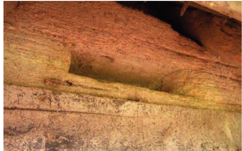
Plate 21: Chase mortise in face of wall plate, under eaves, from former projecting oriel
