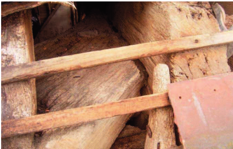
Plate 22: Curved corner brace and end of tie beam at E end of barn
