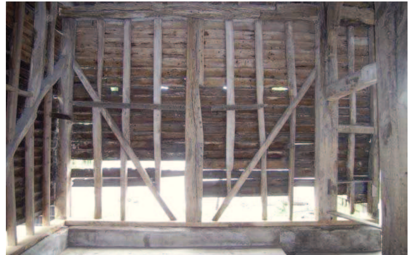
Plate 13: Secondary framing and possibly reused tie at W end of N wall
