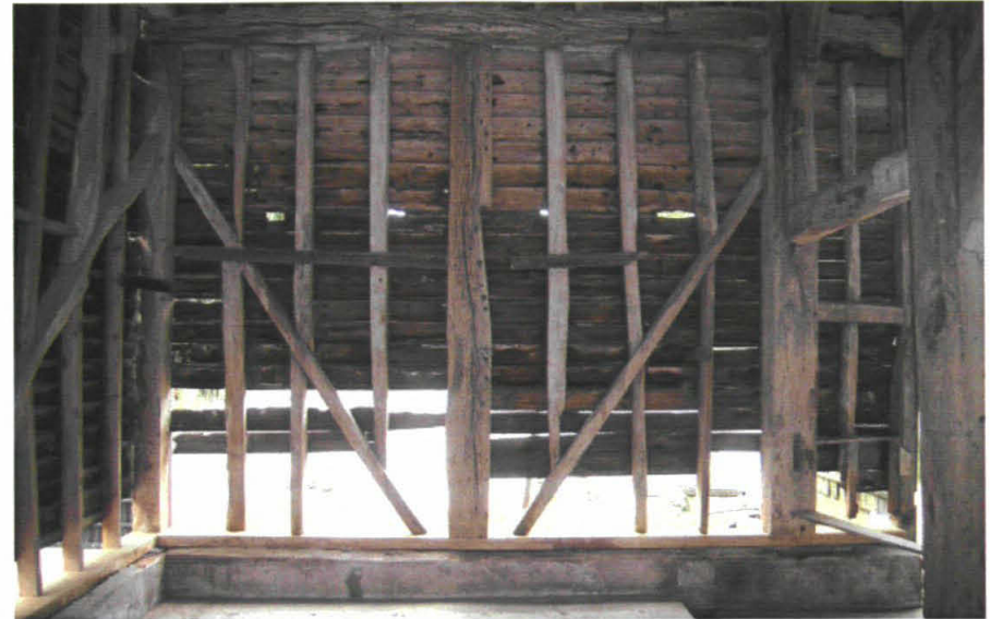
Plate 13: Secondary framing and possibly reused tie at W end of N wall
