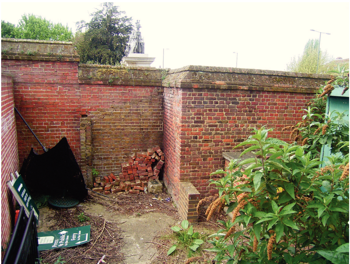
Plate 11: South-western elevation of wall beside trophy gate showing evidence of former structures
