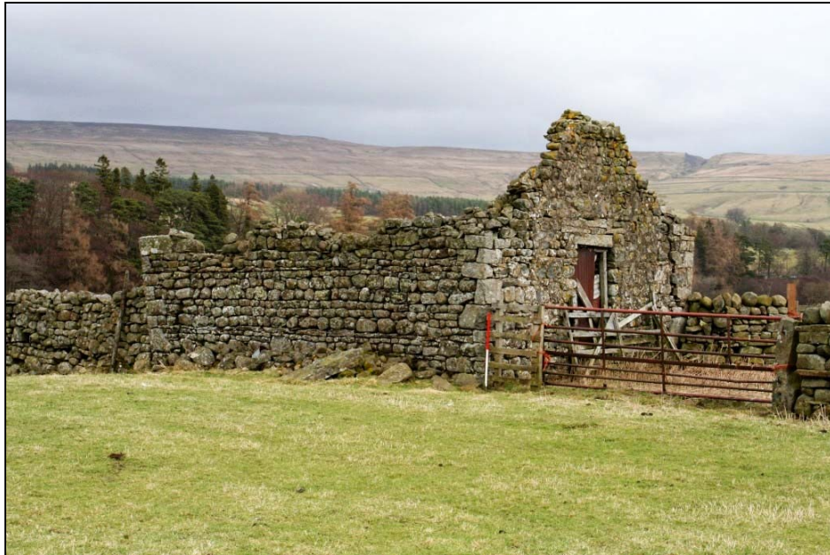
Plate 24: An example of the typical state of survival of field barns in Holwick (1033)
