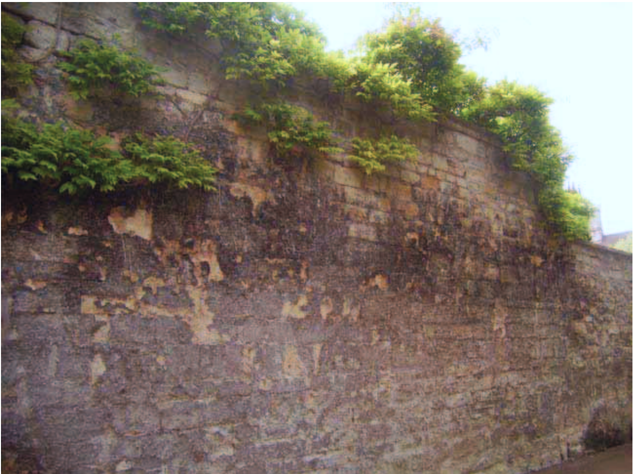
Plate 6: President's Lodgings Wall, Magdalen College: Coursing on north face, looking south west
