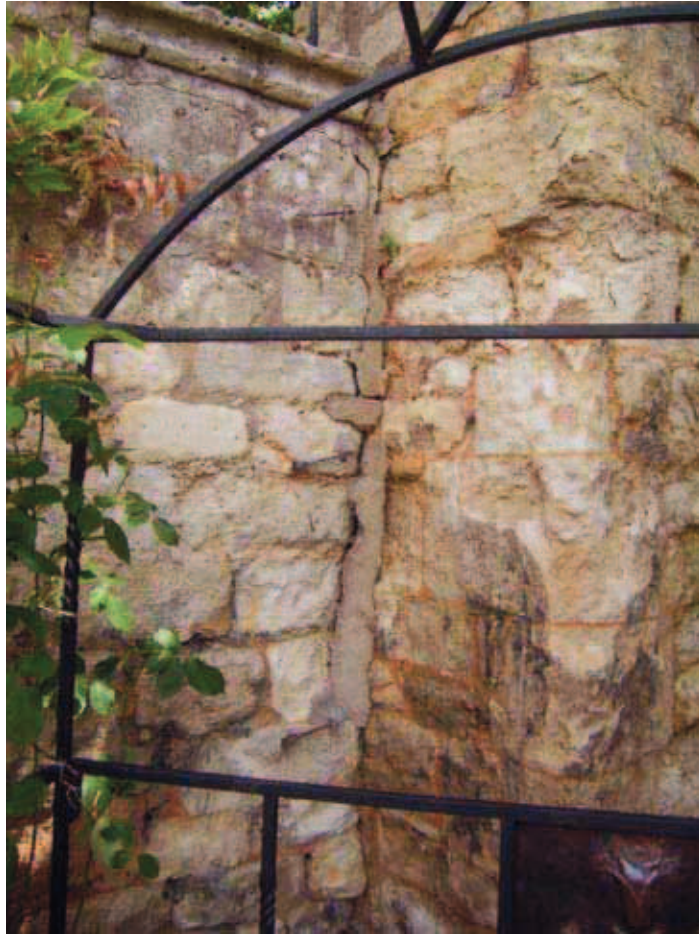
Plate 7: President's Lodgings Wall, Magdalen College: Cement repairs on south face, looking north east
