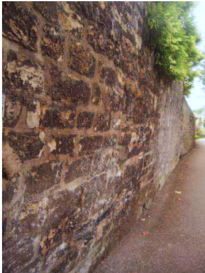
Plate 2: President's Lodgings Wall, Magdalen College: Bulge in north face, looking west
