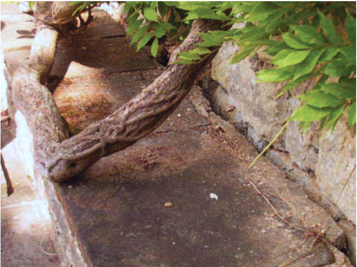
Plate 8: President's Lodgings Wall, Magdalen College: Evidence of movement on south face
