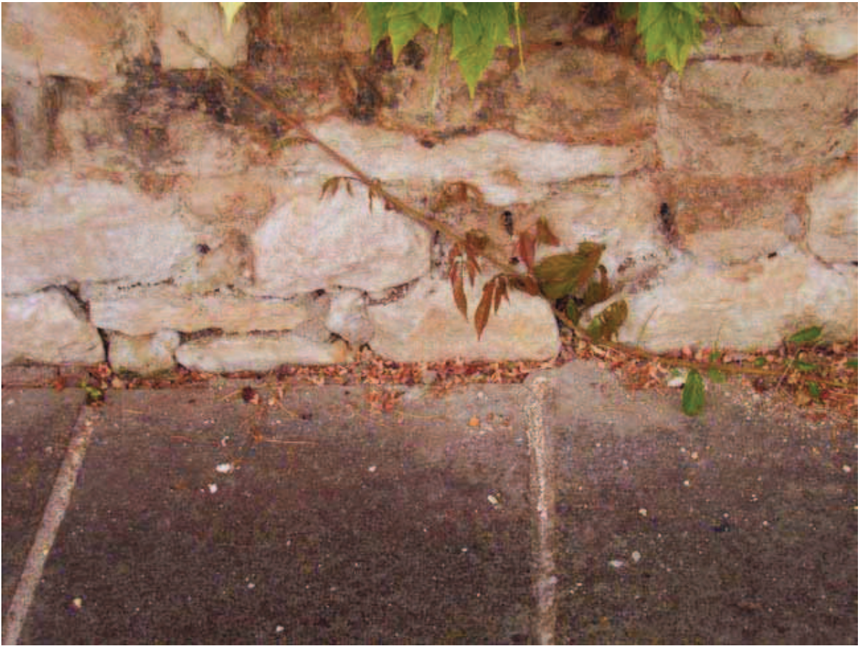
Plate 9: President's Lodgings Wall, Magdalen College: Foot of wall at south side, looking northwards
