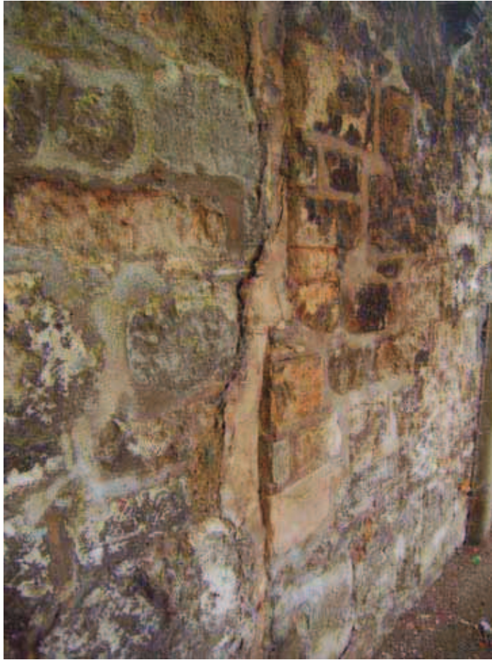
Plate 3: President's Lodgings Wall, Magdalen College: Crack in north face, looking south west
