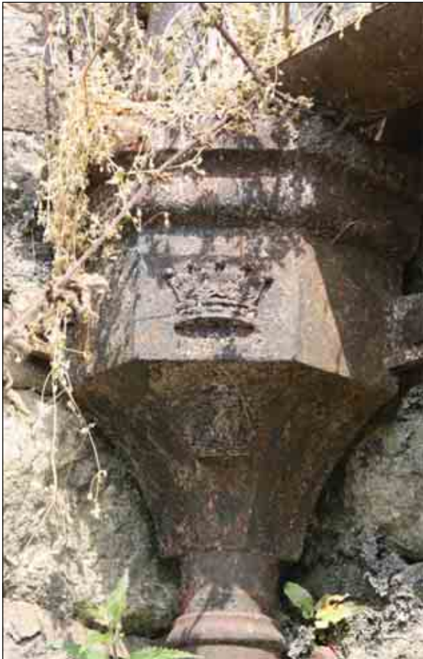
Plate 43: Iron hopper with Fermor-Hesketh crest, Building D
