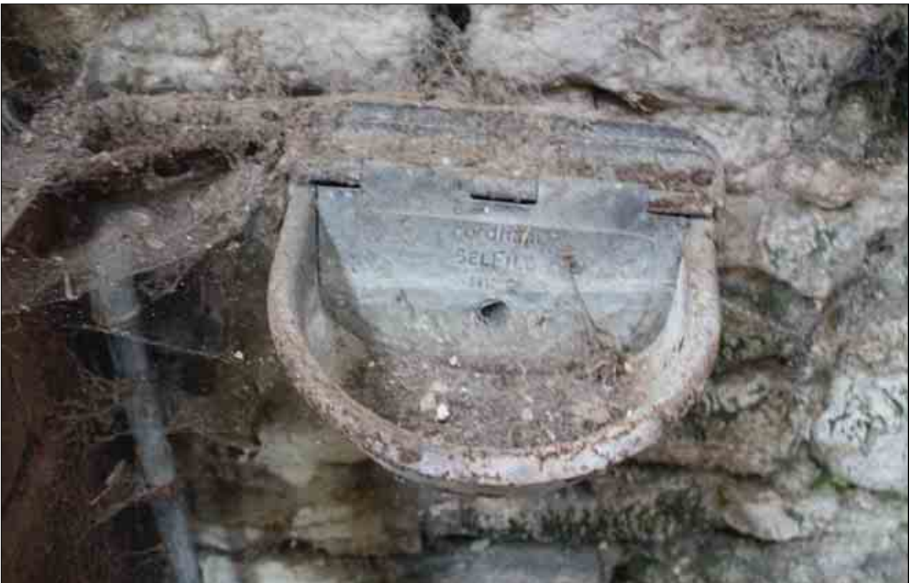
Plate 47: Detail of "Fordham SelfFill", Building D (i)
