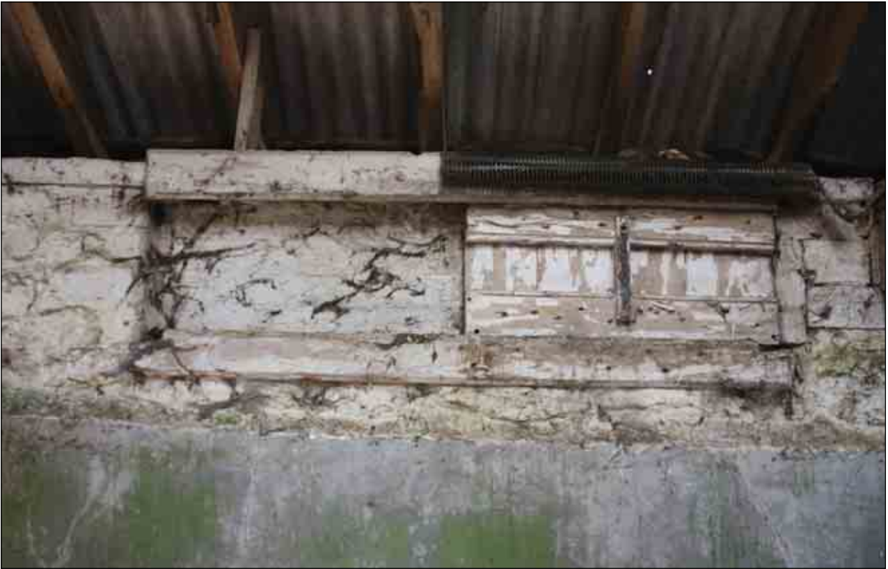
Plate 56: Sliding ventilation, Building D (iii)
