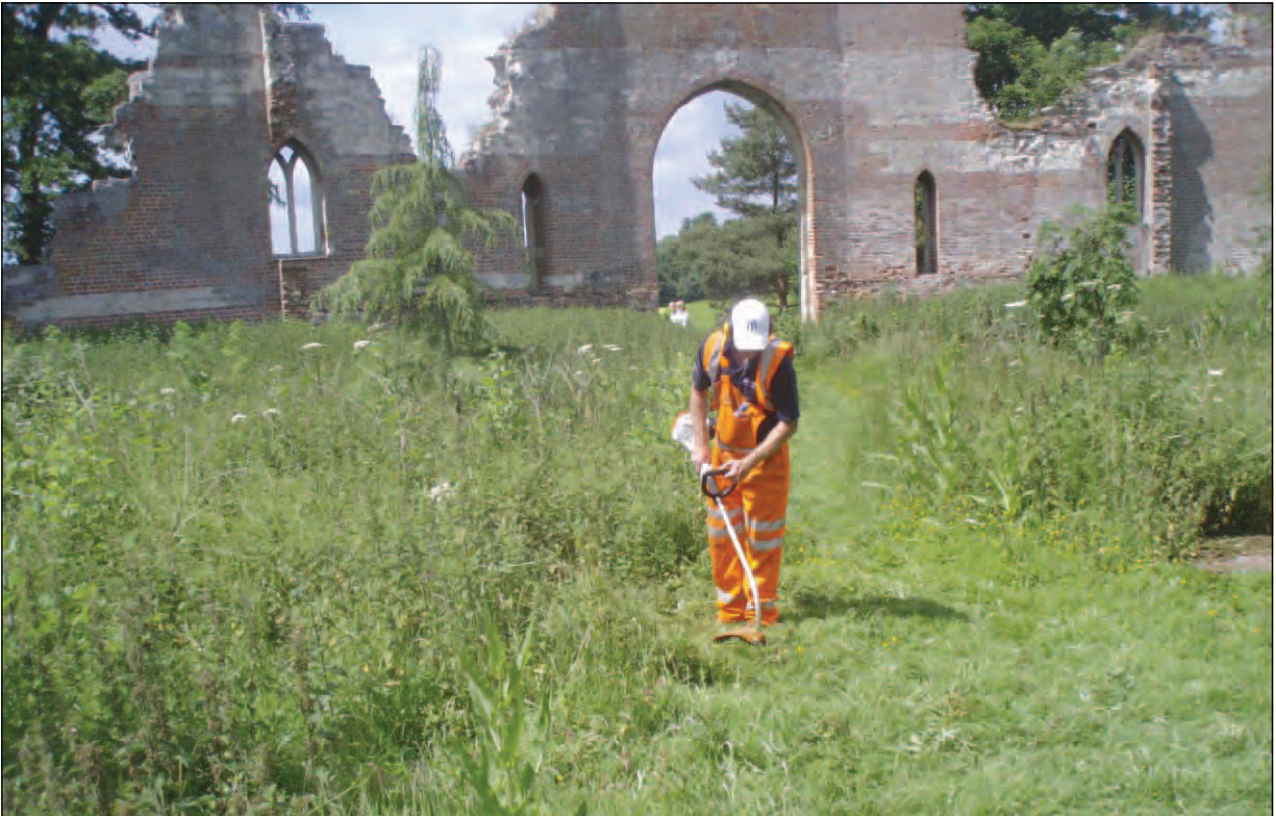
Plate 3: Strimming of vegetation inside the Folly
