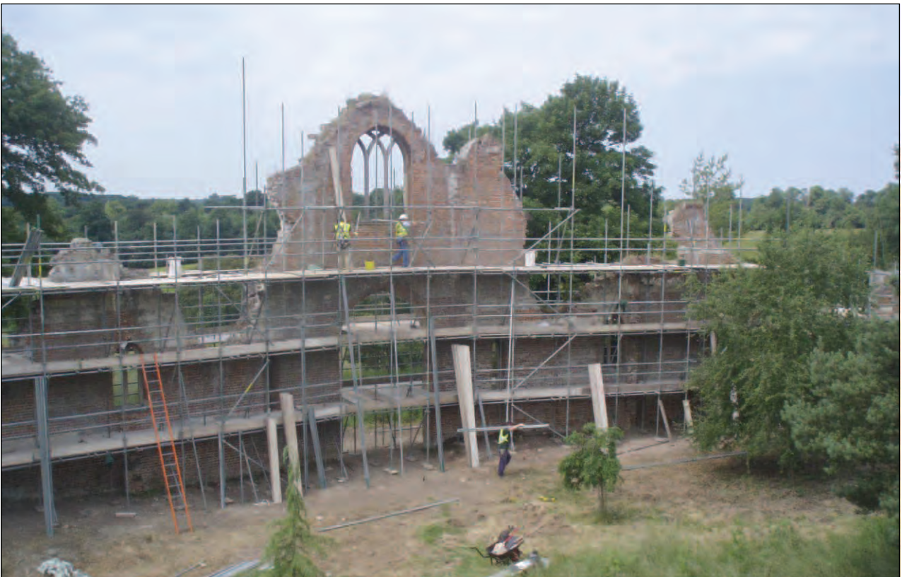
Plate 4: Scaffolding being erected against inside face of south-west wall of the Folly
