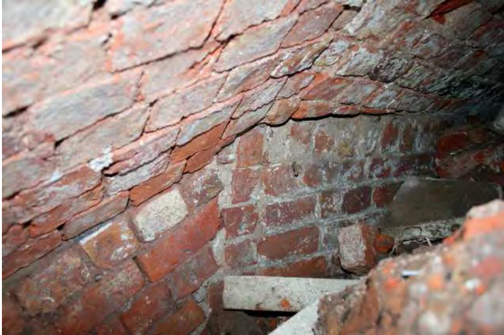
Plate 34: Irregular joint between sloping and level sections of vault side wall
