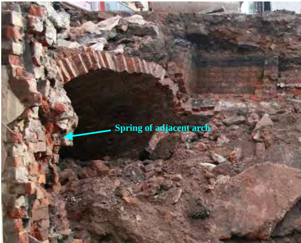
Plate 36: Broken north wall of vaulting, with stub of adjacent vault identified
