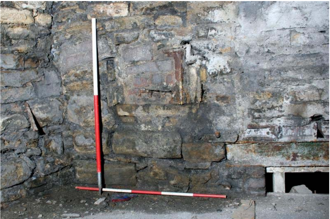
Plate 20: Blocked bearing box in the south wall of the economiser house
