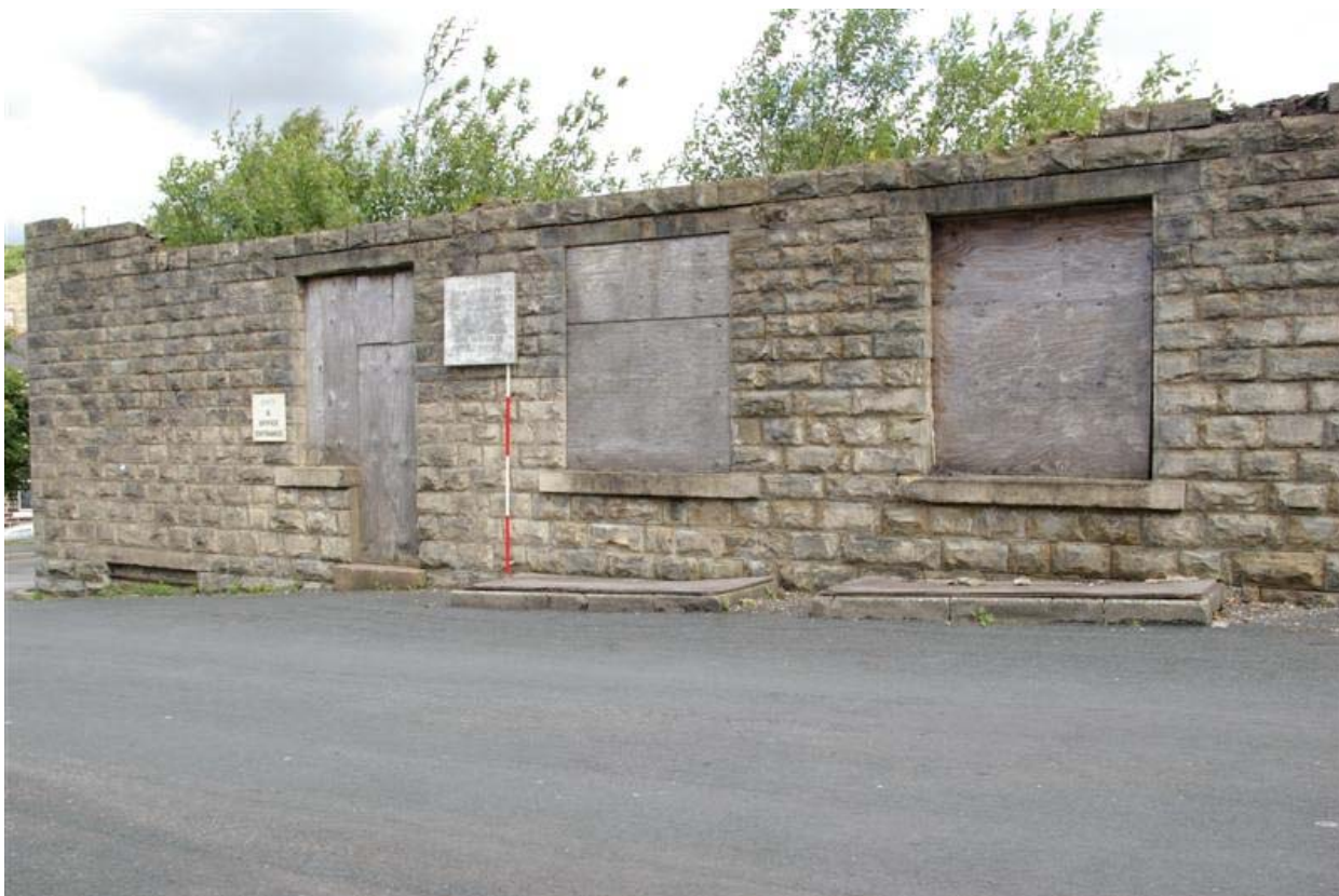
Plate 4: Boarded windows and doorway at the north end of the west wall of the weaving shed
