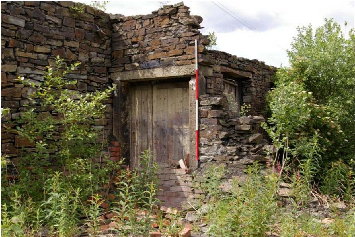
Plate 6: Remains of the south elevation of the spinning block projecting from the west wall of the weaving shed
