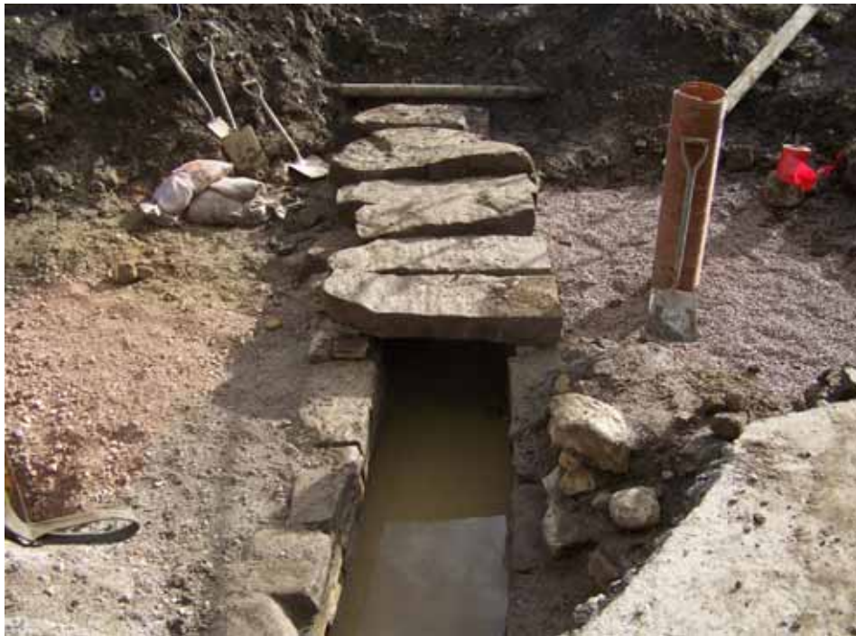
Plate 13: Reinstatement of capping stones 134 over tail-race channel SG 168 following insertion of pipe
