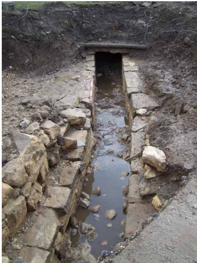
Plate 6: The tail-race for the former corn and saw mill (SG 168), looking south-east, with capping stones removed, showing stone lining 170/171
