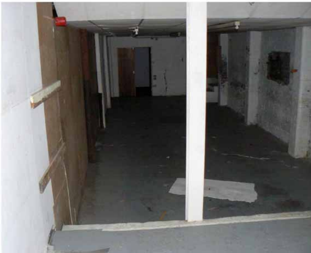
Plate 11: Inside the rear portion of 107 George Leigh Street, showing the reduced floor level
