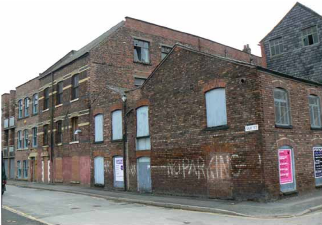
Plate 12: The Silk Street frontage of the study area, showing the rebuilt rear portion of 107 George Leigh Street, the two-storey structure infilling the former yard, and the rear element of 109 George Leigh Street (80 Silk Street)
