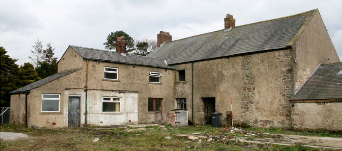
Plate 11: General view of Cross Keys Inn and attached barn, from the south-west
