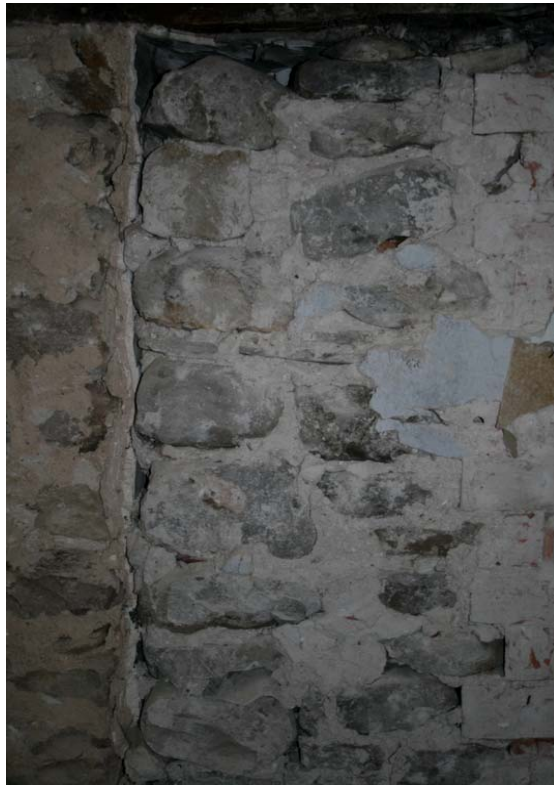
Plate 20: Original wall plaster within window blocking, Room F3
