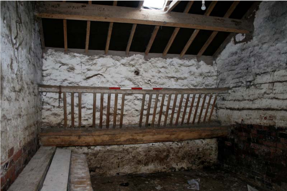
Plate 44: Manger, in central bay of stables
