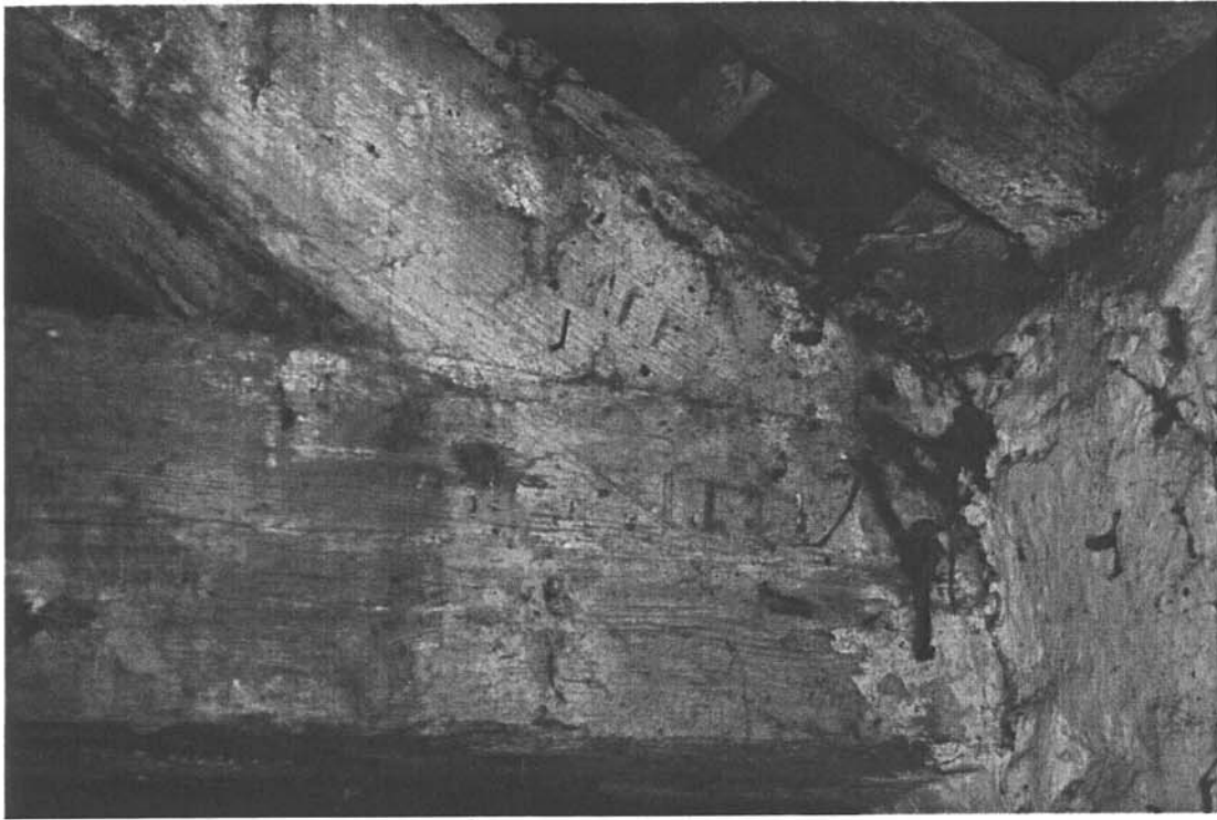
Plate 5: Detail of the carpentry marks on one of the trusses within the West Cow Shed
