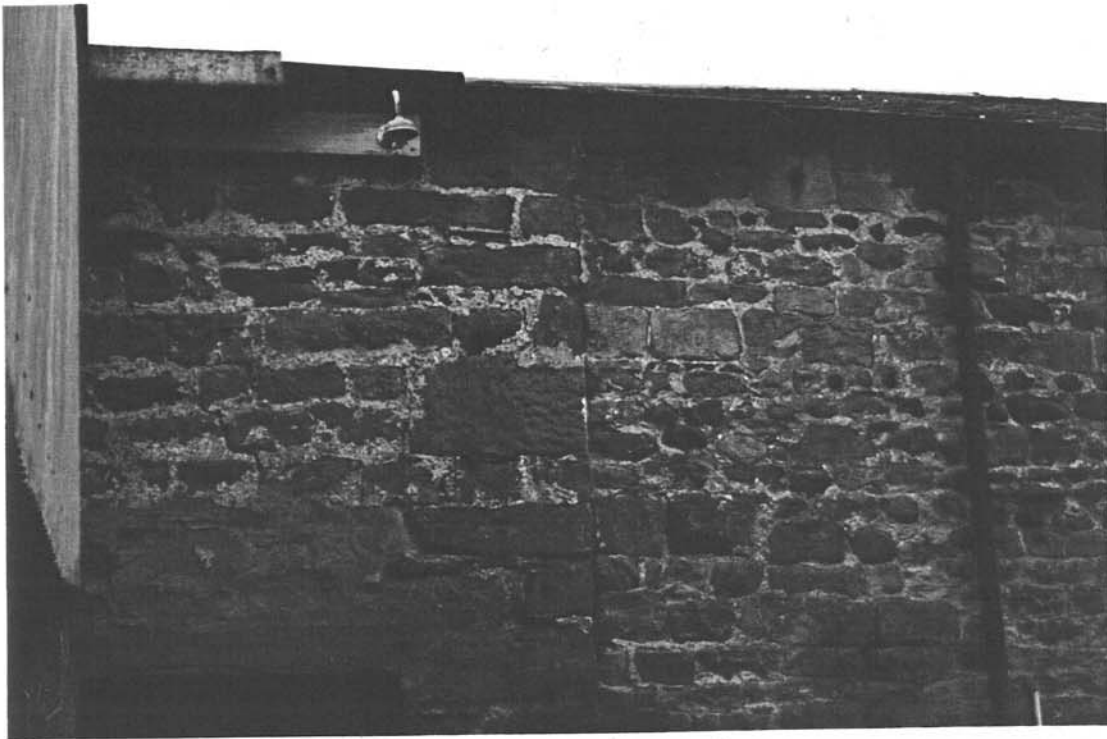
Plate 22: The butt-joint between the original and secondary builds on the east elevation of the East Barn
