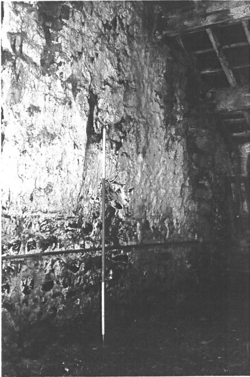
Plate 27: General view of the interior of the single-storey extension at the south end of the East Barn
