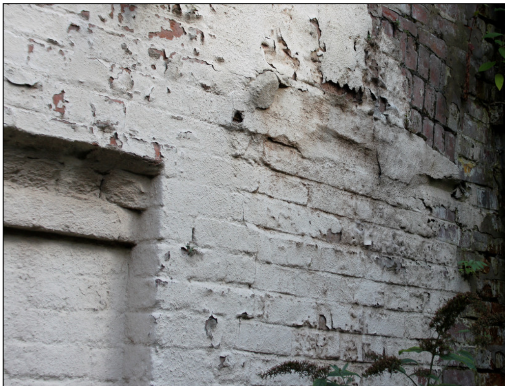
Plate 29: Blocked arched window, ground floor of Building C with adjacent inserted doorway
