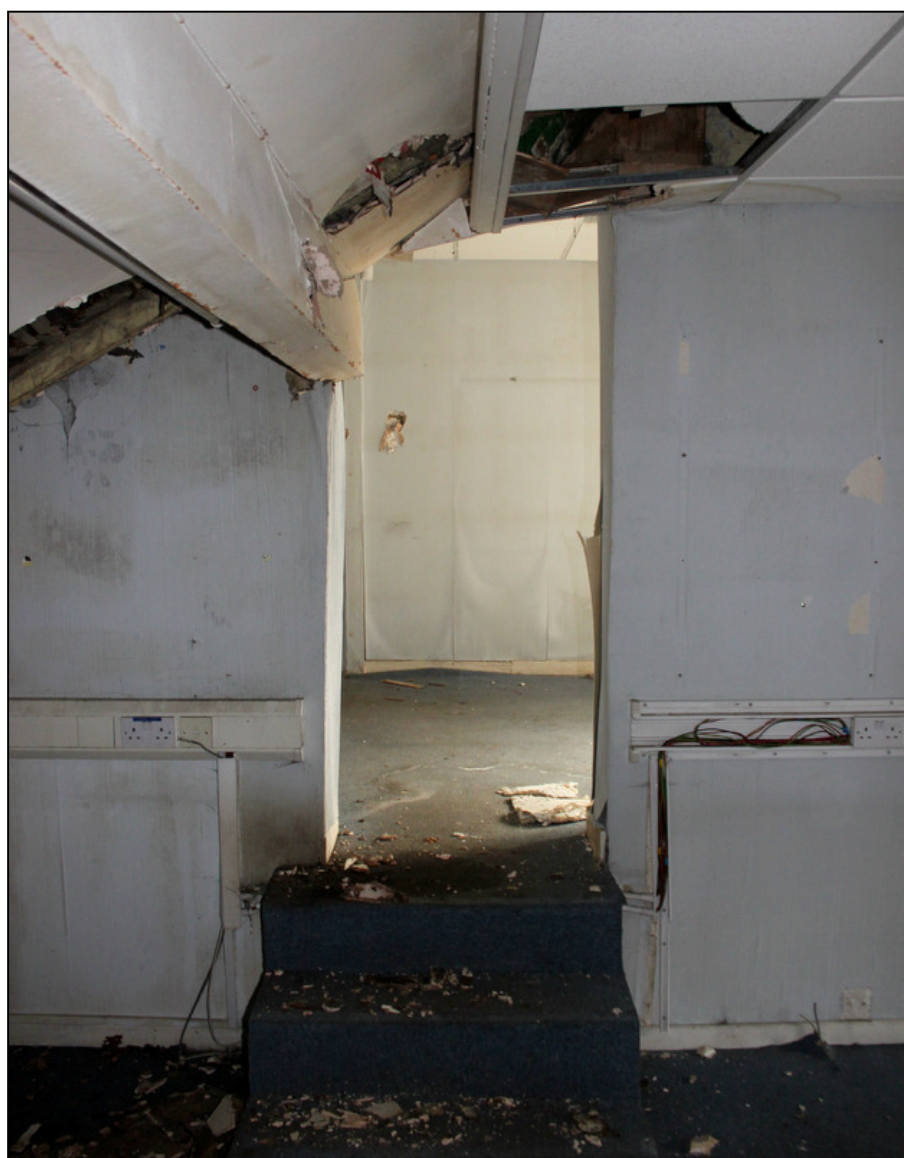
Plate 11: Sloping ceiling of rear first-floor rooms in west range of Building A, and steps up to Building B
