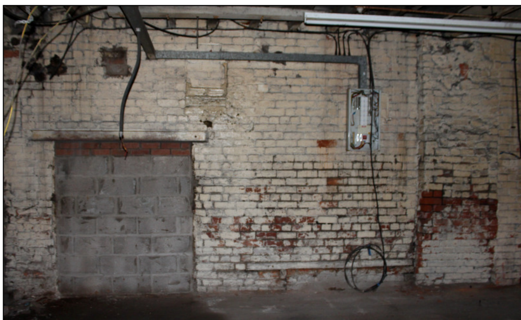
Plate 23: Blocked bearing box in internal wall between Bays 3 and 4, looking west
