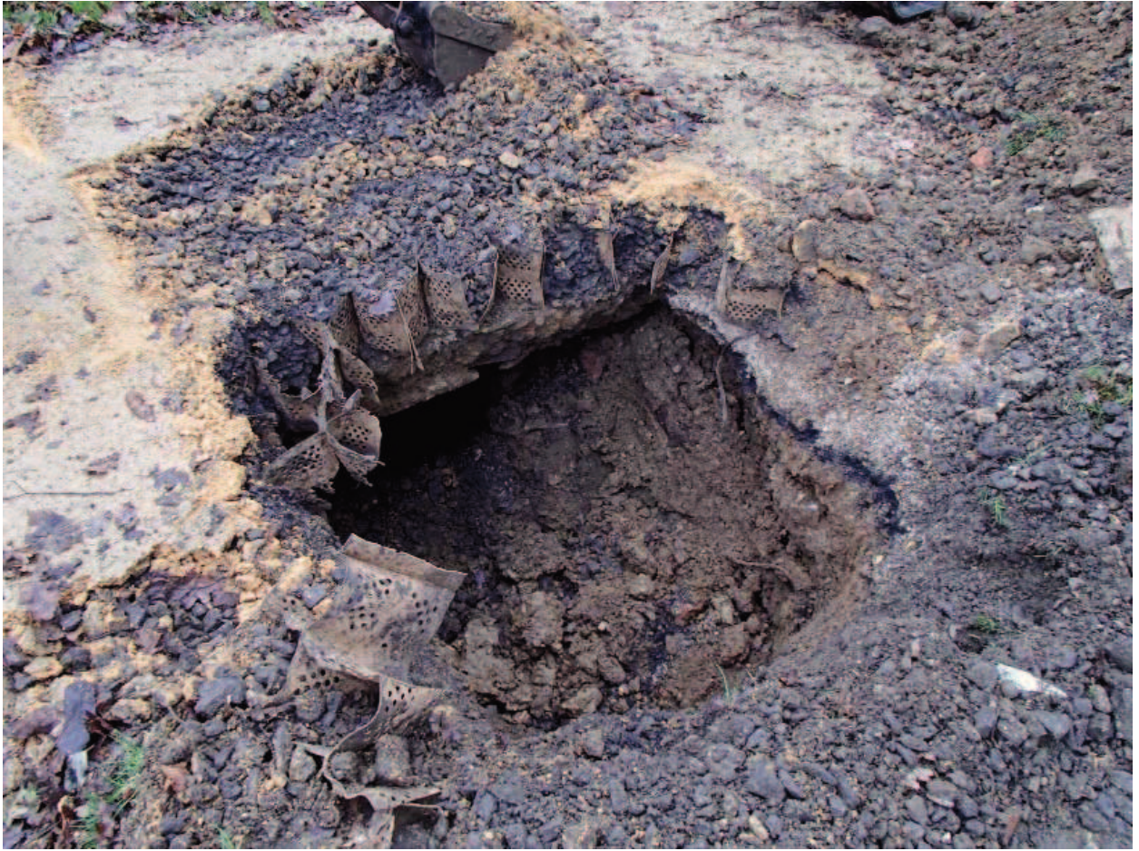
Plate 1: Showing collapse of path
