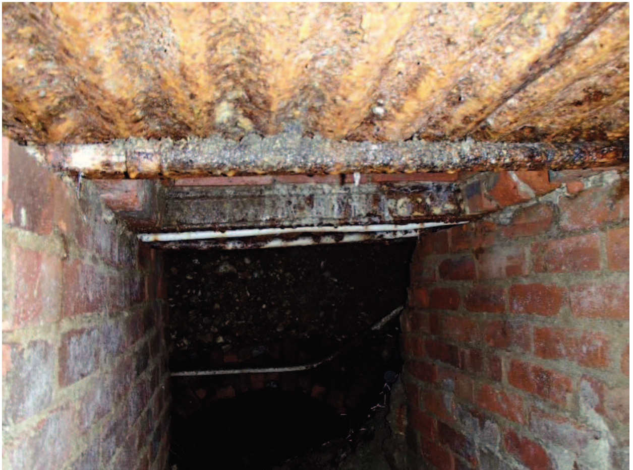
Plate 2: State of corroded concrete slab
