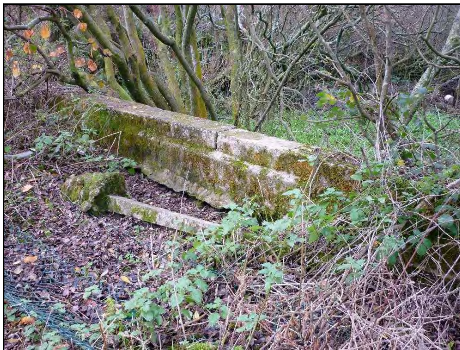
Plate 5: The retaining wall along the southern side of the pond at the north end of the Whangs Beck culvert to be upsized
