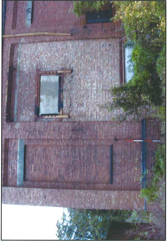
Plate 28: Building 10, blocked winder cable openings, view north-west, scale of 2.0m
