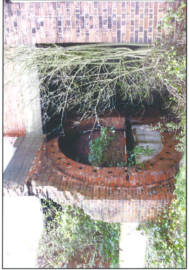
Plate 8: Fan House, circular brick opening at base of tower on north-east side
