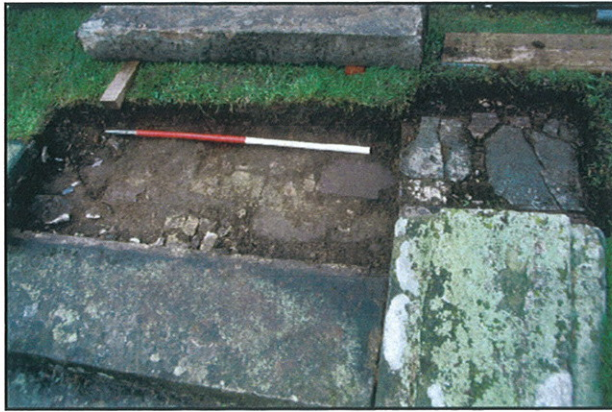
Plate 9 - monitoring works carried out during removal of step stonework, steps S2. Looking north.
