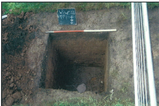
Plate 5 - Trial pit 1, excavated along course of new disabled access path. Looking south.
