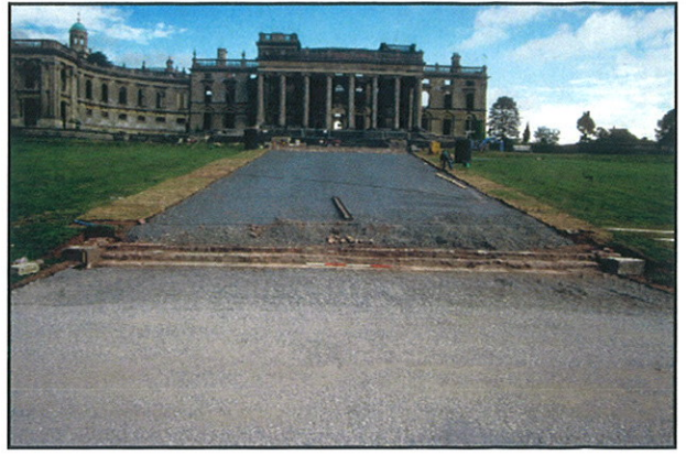
Plate 50 - Preparation of paths for re-surfacing with steps S5 in foreground. Looking north.
