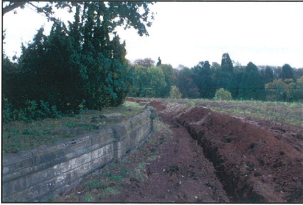
Plate 67 - Service trench excavated along east side of eastern balustrade of gardens for new pumphouse. Looking north.
