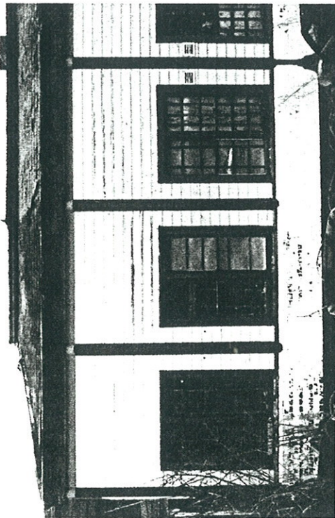
Plate 44 Typical W1 type wall panel as used on the flanking wings. Both the panels and columns originally continued to just above ground level.
