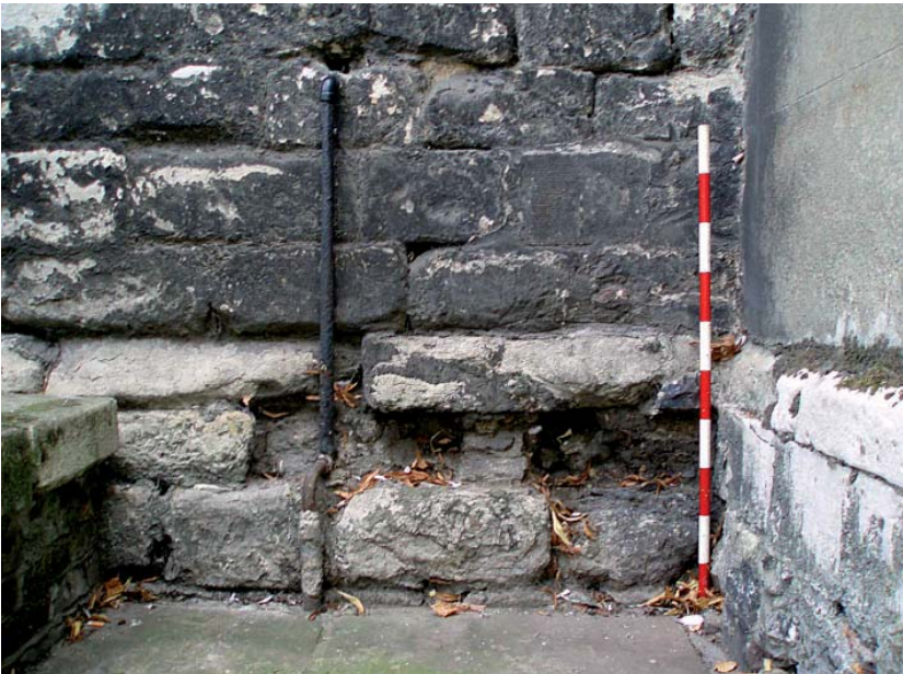
Plate 11: All Saints Vestry, Kingston: North Elevation - replacement stone with tool marks and weathered plinth
