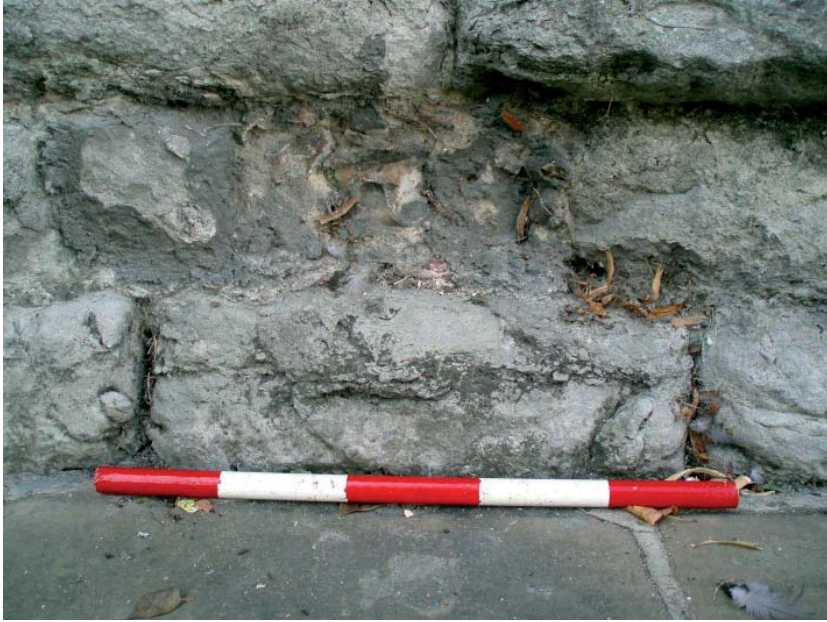
Plate 5: All Saints Vestry, Kingston: East elevation - rubble infill at base of elevation
