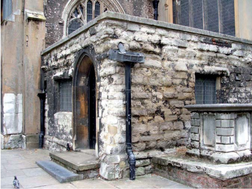
Plate 9: All Saints Vestry, Kingston: North Elevation - repairs to corner and discolouration of stonework caused by damp
