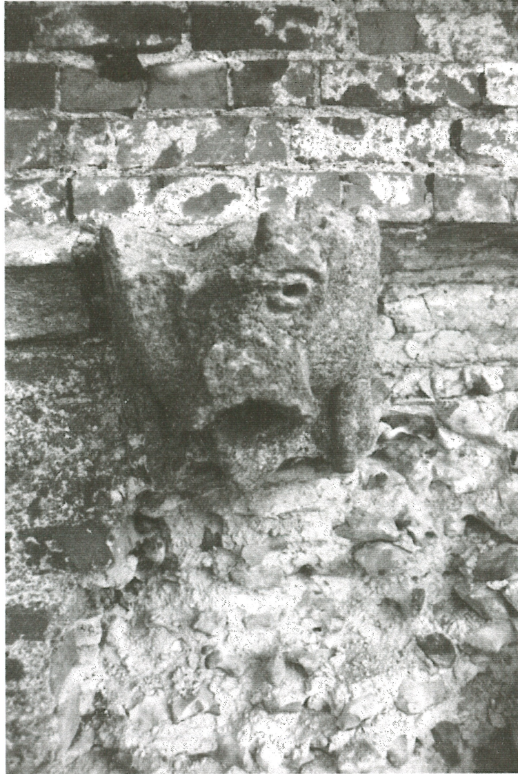
Plate 5 Grotesque on west face of tower parapet
