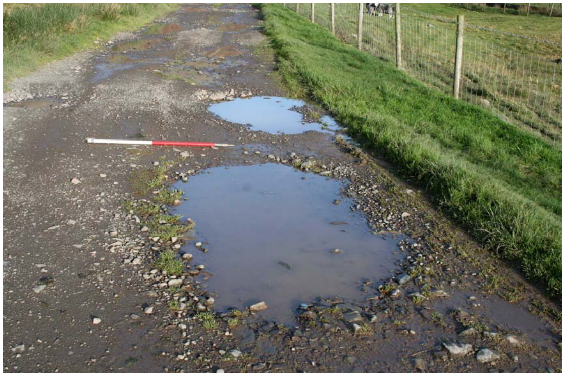
Plate 15: Track pot holes looking north-east (photo position 11)
