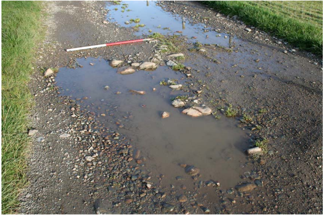
Plate 17: Detail of surface erosion at photo position 13
