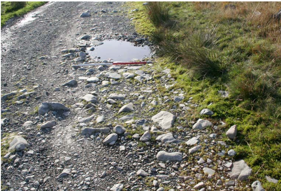
Plate 8: Area of exposed cobbles and pot hole (photo position 4)
