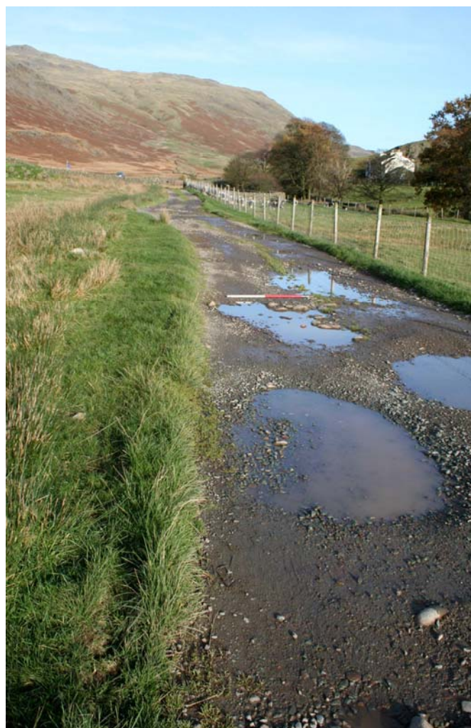
Plate 16: An extensive area of surface erosion at photo position 12, looking north-east
