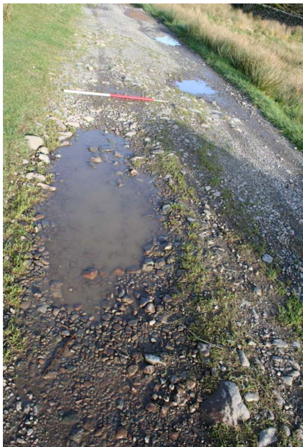
Plate 11: Area of erosion at photo position 7
