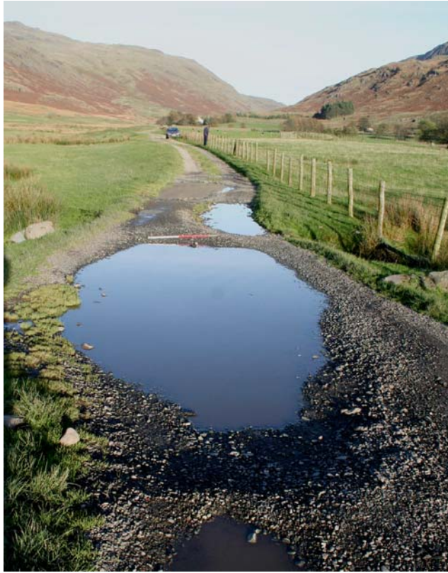
Plate 29: One of the larger areas of erosion (photo position 25)
