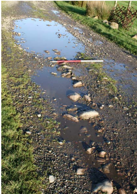
Plate 26: Area of severe erosion at photo position 22
