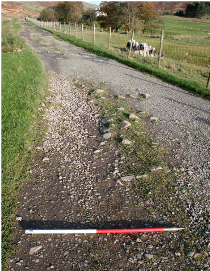
Plate 19: Exposure of foundation cobbles in the middle of the track at photo position 15
