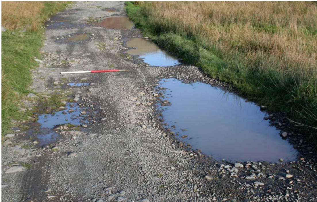
Plate 10: A typical group of potholes along the track (photo position 6)
