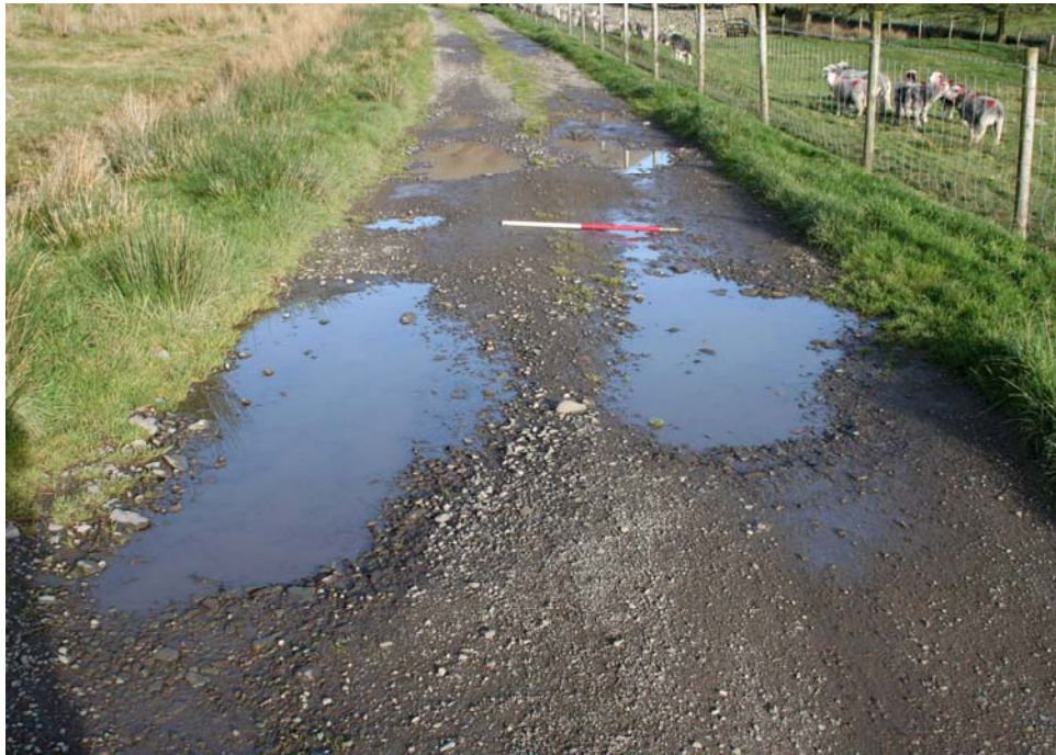
Plate 14: Erosion scars on the eastern part of the track (photo position 10)
