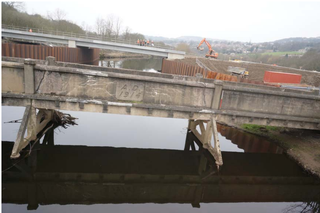
Plate 41: South-east-facing bridge elevation and trestles (4a) and (4b); also showing cut-waters (5) and (5a) (DSC00493)
