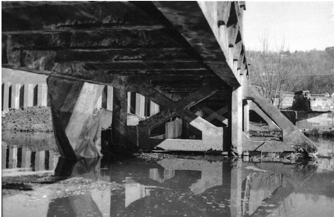
Plate 51: North-facing view showing trestles with diagonal internal bracing ( 4b ) and ( 4a ), and cut-waters ( 5a ) and ( 5 ) (MF SB02_09)
