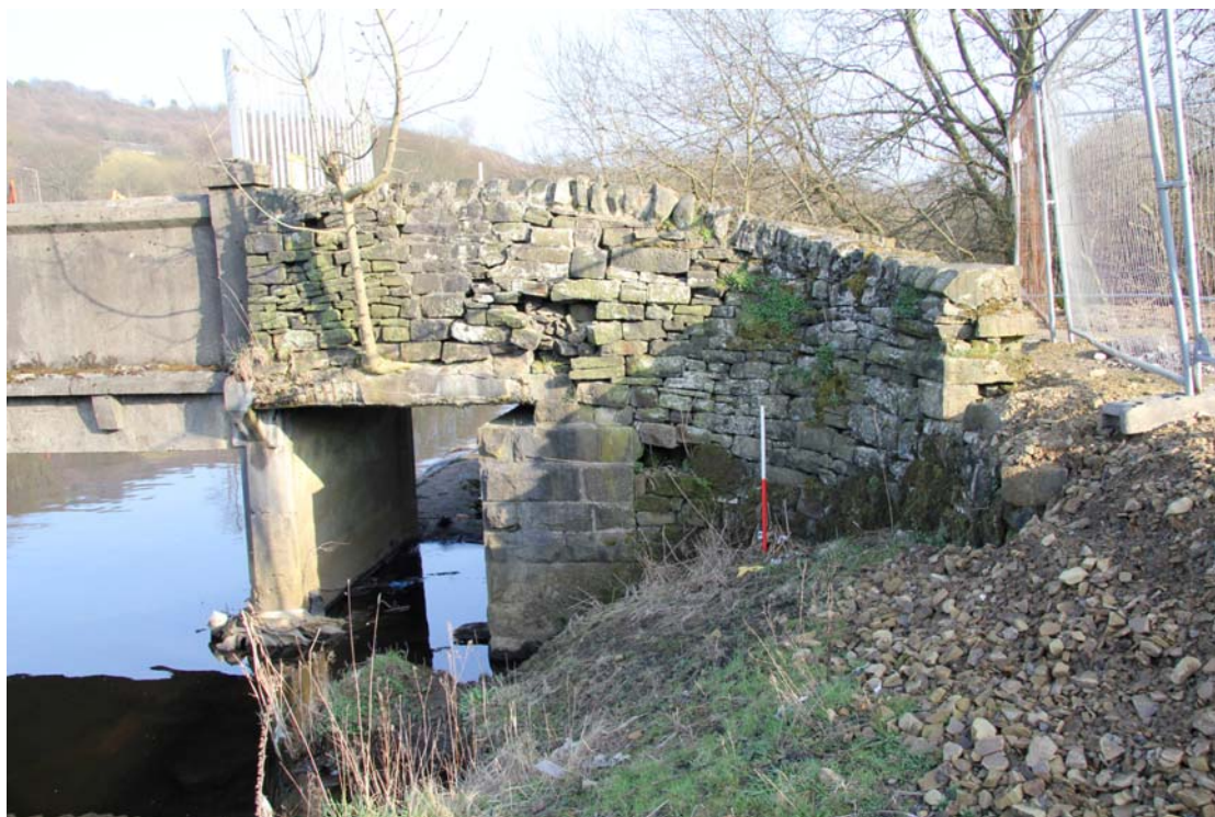
Plate 56: East-facing view showing southern trestle ( 4c ), parapet ( 10 ), and western rubble wing wall ( 11a ) (IMG_2423)
