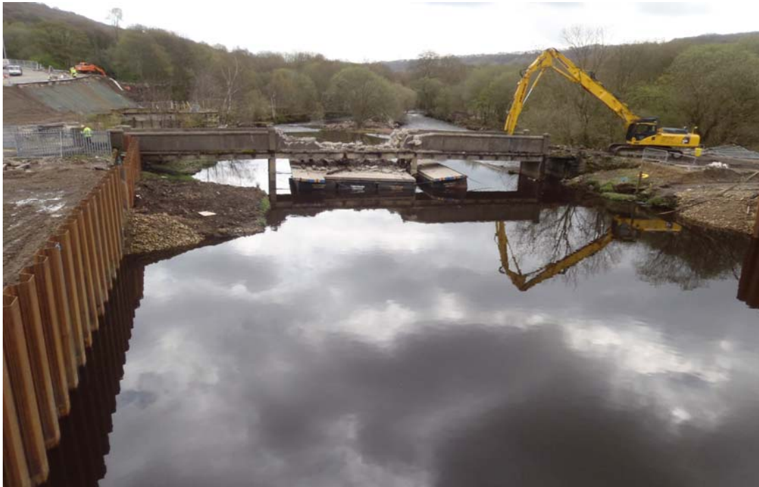
Plate 85: Sterne Bridge during the demolition process, with central section of concrete parapet (10) removed (P3020740.JPG)
