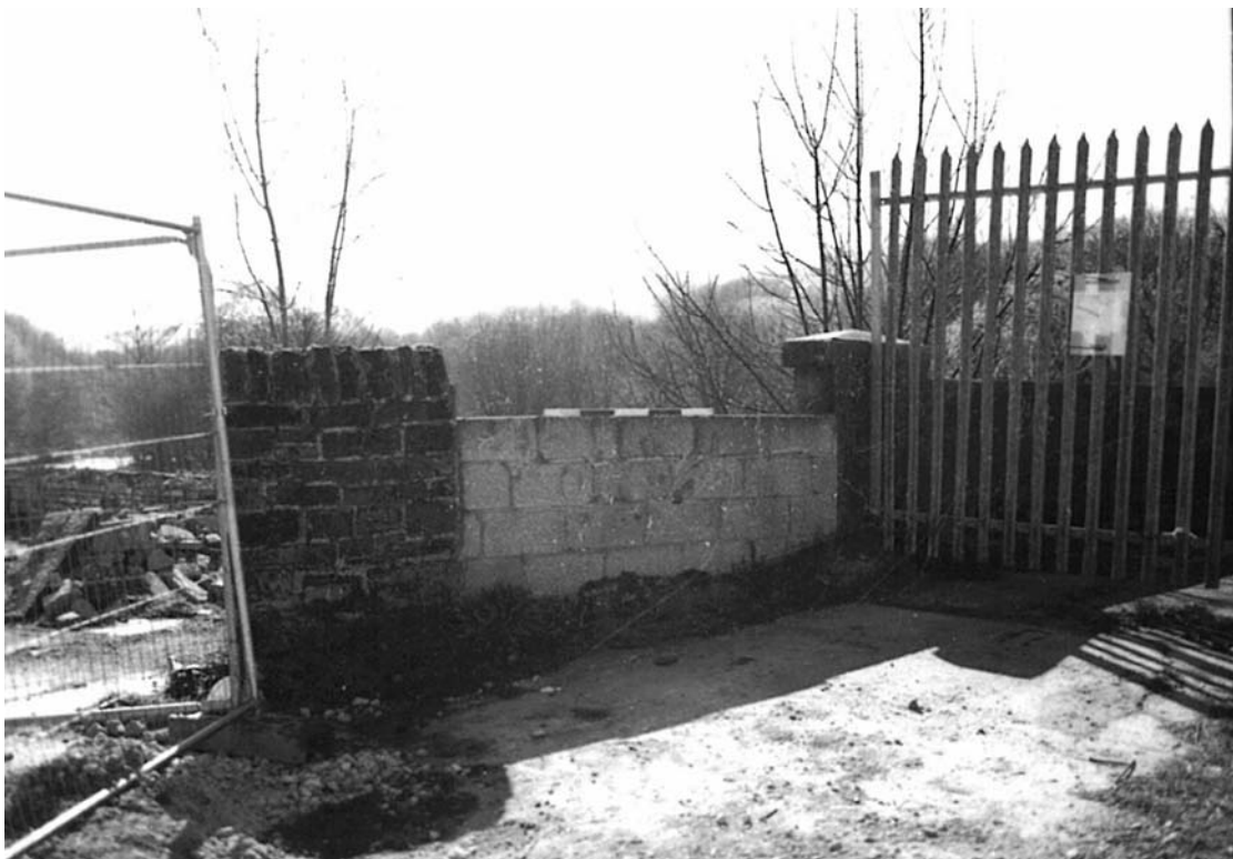
Plate 28: Blocked stepped access (1) and surviving section of eastern wing wall (2) (MF SB05_11)
