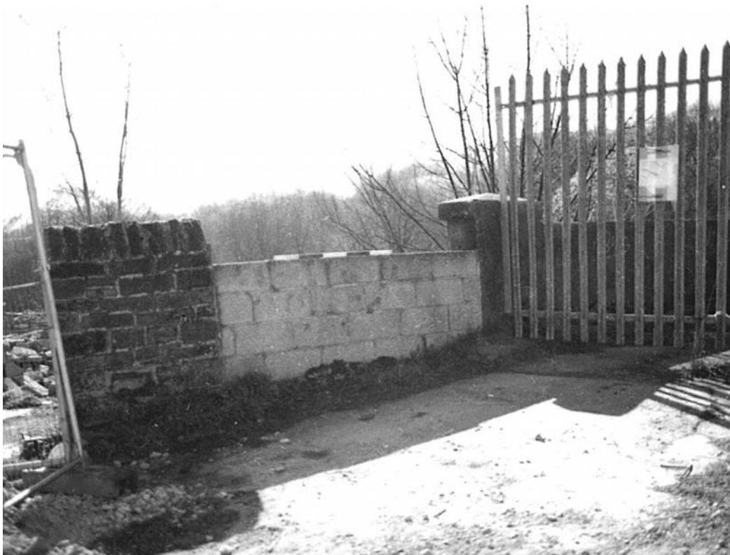
Plate 26: Blocked stepped access (1) and surviving section of eastern wing wall (2) (MF SB05_09)
