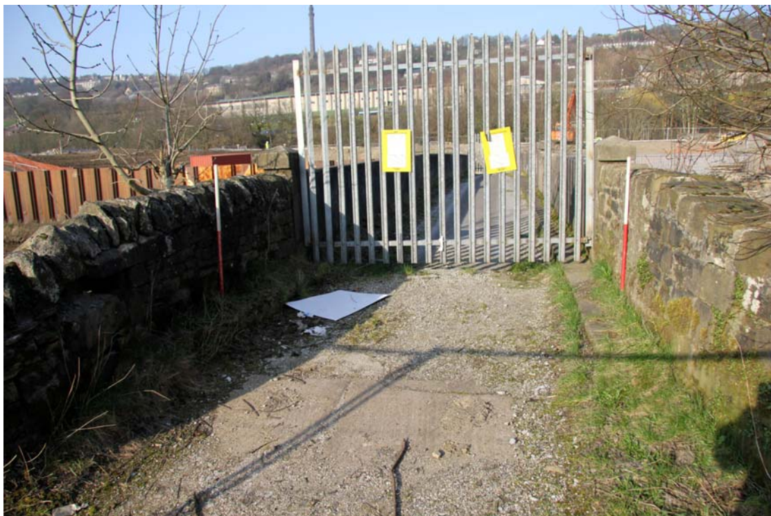
Plate 83: View to north bank showing modern bridge deck (14) flanked by stone parapet wing walls (11) (IMG_2397)
