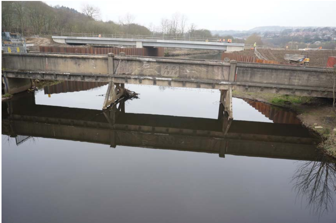
Plate 47: South-east facing bridge elevation showing trestles (4a) (4b) and (4c); also showing cut waters (5) and (5b) (DSC00512)
