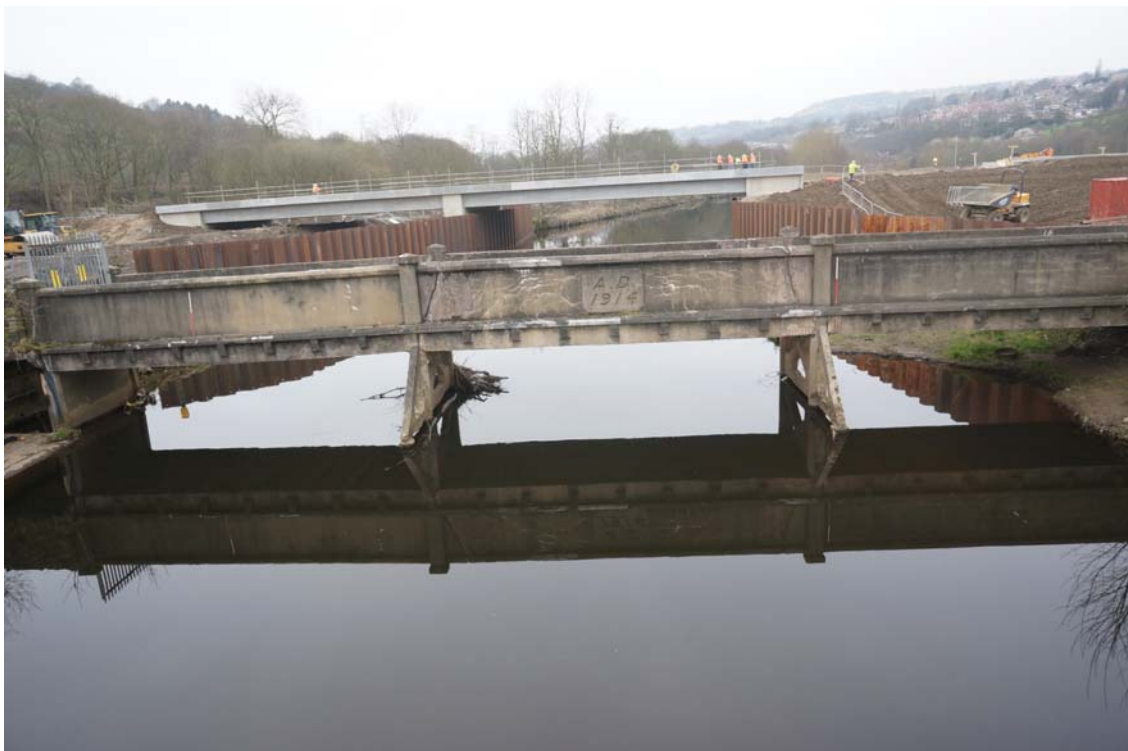
Plate 46: South-east facing bridge elevation showing trestles (4a) (4b) and (4c); also showing cut-waters (5) and (5b) (DSC00510)
