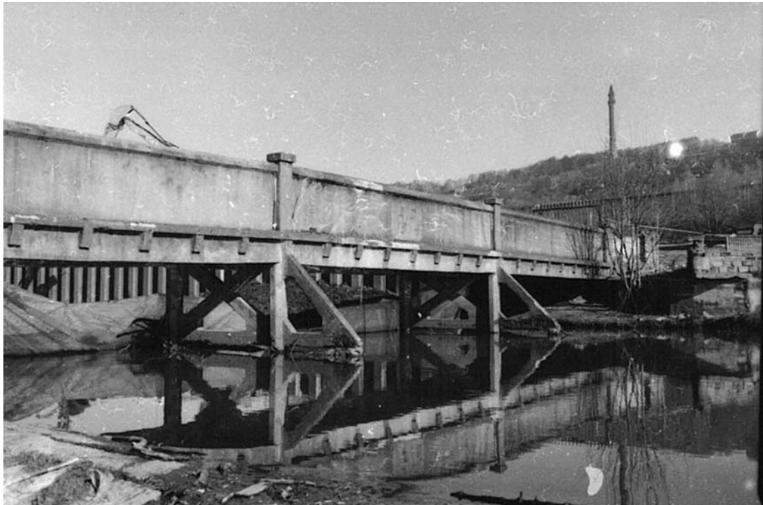
Plate 33: North-facing view showing south-east-facing bridge elevation, trestles (4a) and (4b), and cut-waters (5) and (5a) (MF SB03_04)
