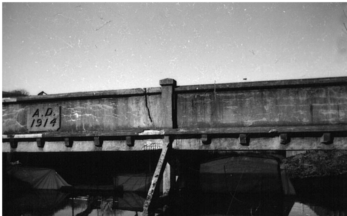
Plate 64: West-facing view showing parapet and parapet sill ( 10 ) over cross beams ( 8 ) with vertical pillar ( 9a ) (MF SB06_11)
