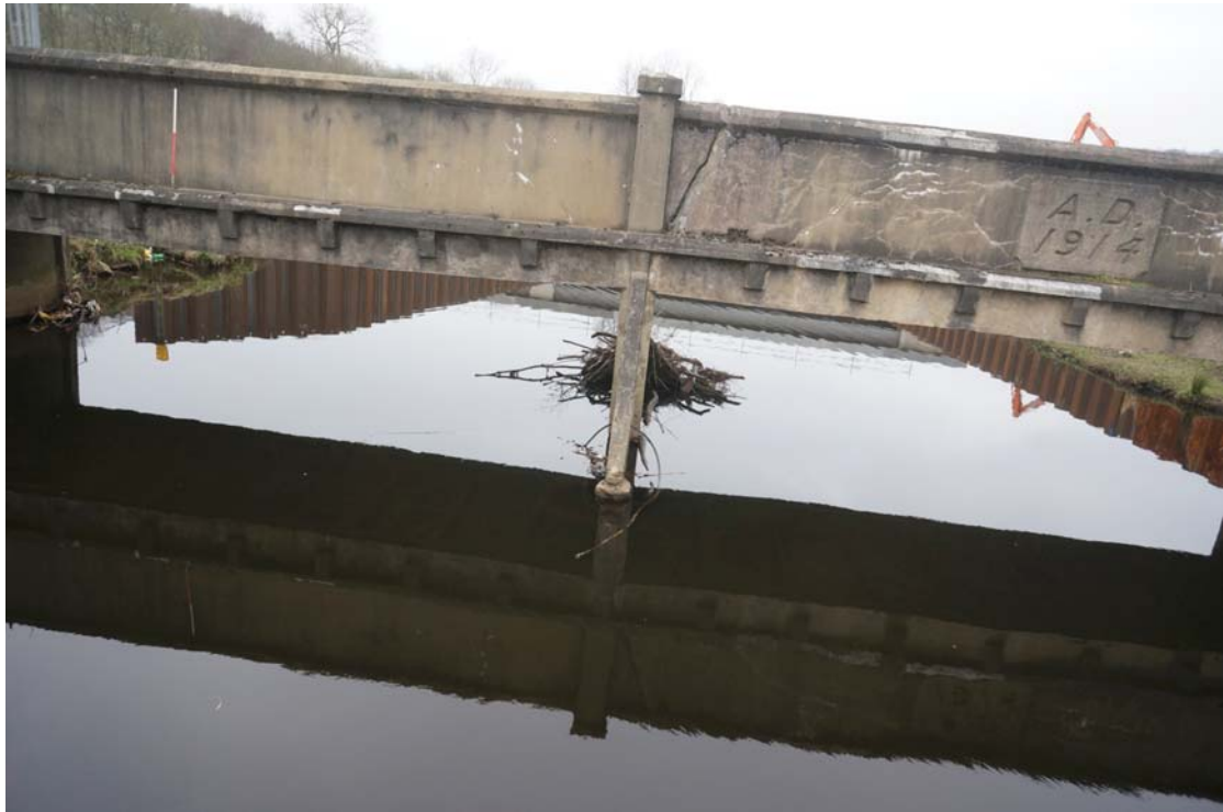
Plate 43: South-east-facing bridge elevation and trestle (4b); also showing elevation view of cut-water (5a) (DSC00499)
