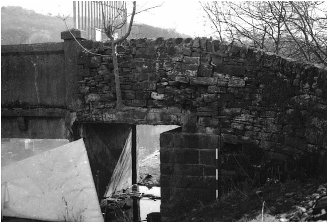
Plate 59: East-facing view showing southern trestle (4c) and western rubble wing wall (11a) (MF SB02_04)
