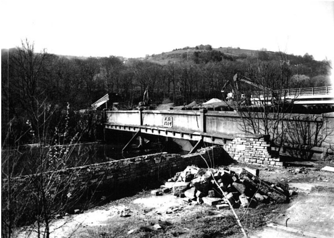
Plate 17: South-facing view across the river Calder, showing the south-east-facing bridge elevation (MF SB04_04)
