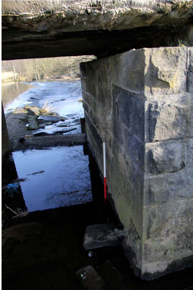
Plate 69: East-facing shot showing a close-up of the ashlar sandstone southern abutment (12) (IMG_2406)
