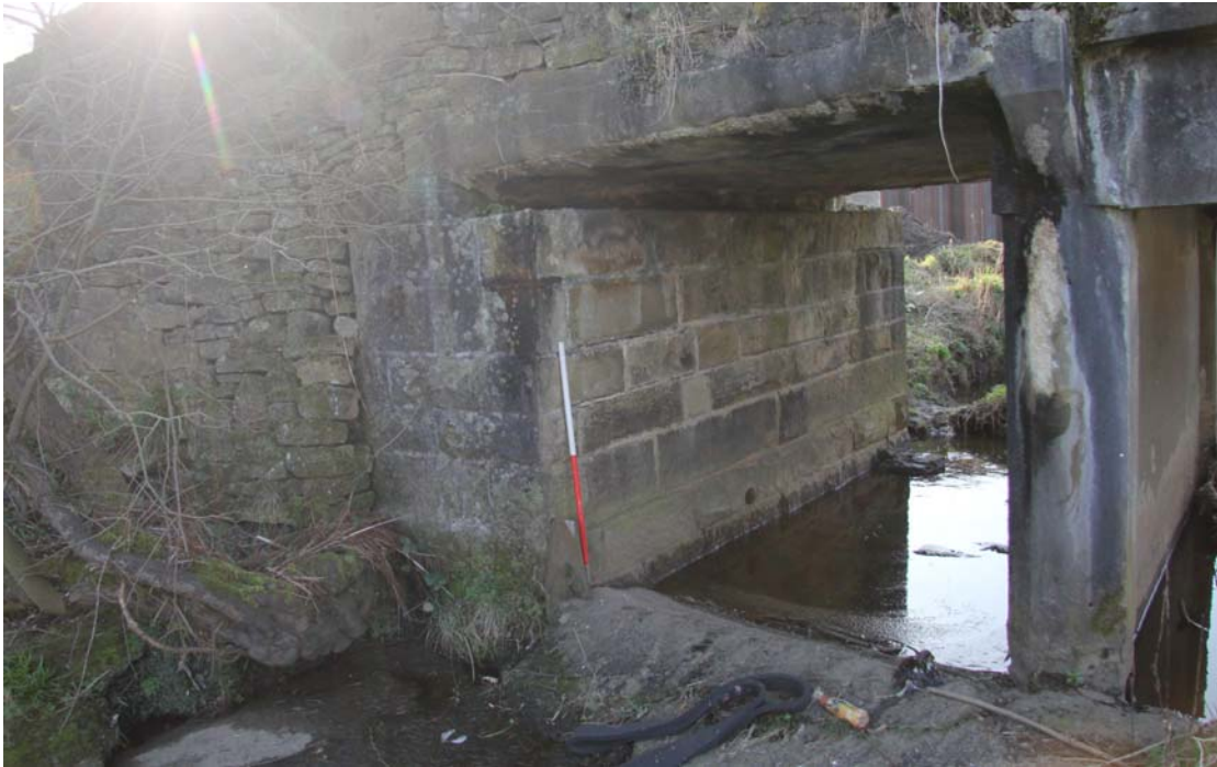
Plate 67: Interface between the south-east wing wall (11), stone abutment (12) and the later concrete parapet wall of bridge with chamfered cross beam (8) (IMG_2408)
