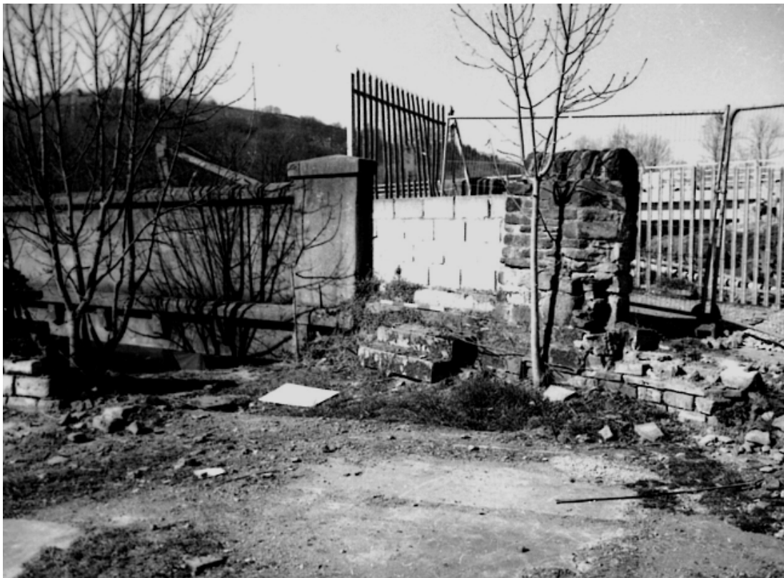
Plate 24: Blocked stepped access (1) and surviving section of eastern wing wall (2) (MF SB05_02)
