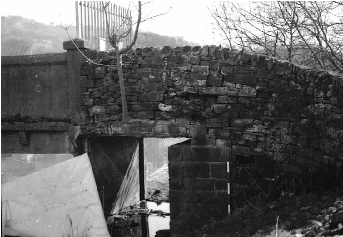
Plate 58: East-facing view showing southern trestle (4c) and western rubble wing wall (11a) (MF SB02_03)
