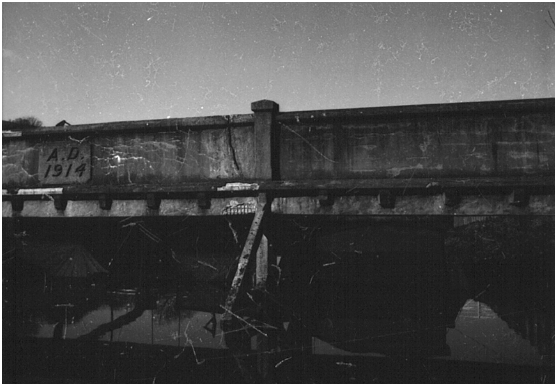
Plate 63: West-facing view showing parapet and parapet sill ( 10 ) over cross beams ( 8 ) with vertical pillar ( 9a ) (MF SB06_10)
