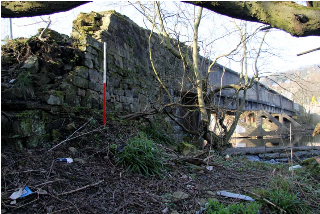
Plate 72: South-eastern wing wall (11) showing truncation and root damage (IMG_2417)
