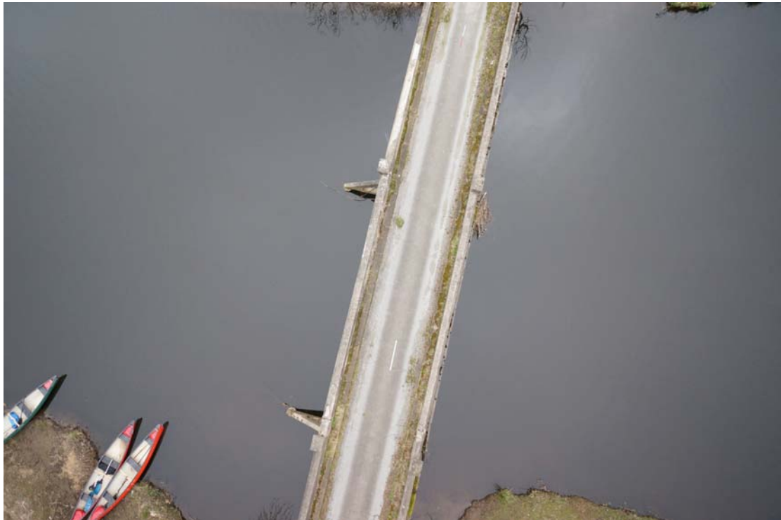
Plate 82: Aerial view showing bridge deck (14) flanked by parapet walls (10) with projecting cut-waters (5) and (5a) on the south-eastern side (DSC00477)
