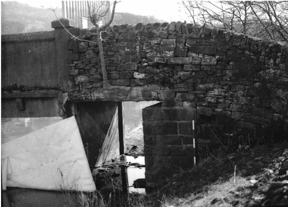
Plate 57: East-facing view showing southern trestle (4c) and western rubble wing wall (11a) (MF SB02_02)
