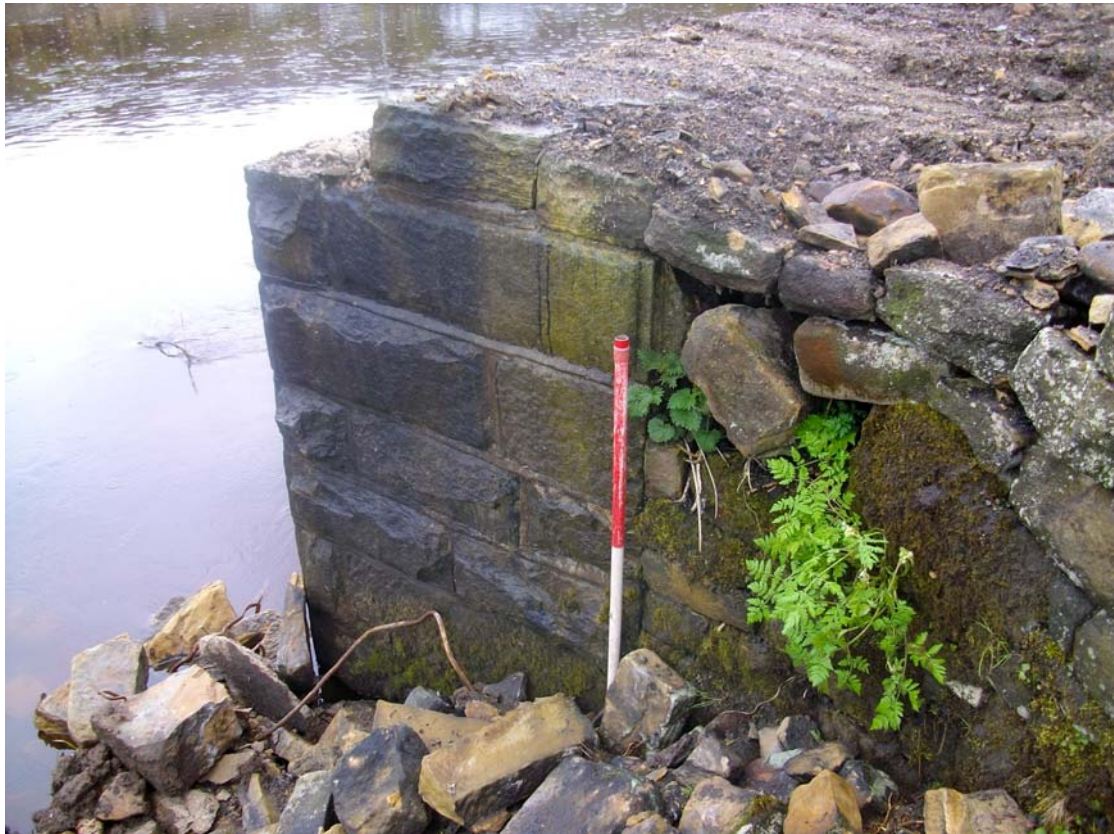
Plate 91: Close-up of interface between southern abutment (12) and remains of rubble wing wall (11) after main phase of demolition (IMG_8754)
