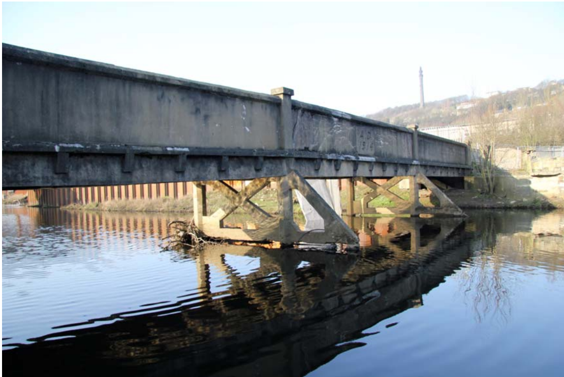
Plate 49: North-facing view showing trestles with diagonal internal bracing ( 4b ) and ( 4a ), and cut-waters ( 5a ) and ( 5 ) (IMG_2420)
