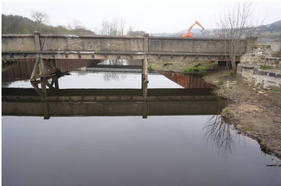
Plate 44: South-east facing bridge elevation showing trestles (4a) and (4b); also showing cut-waters (5) and (5b) (DSC00506)
