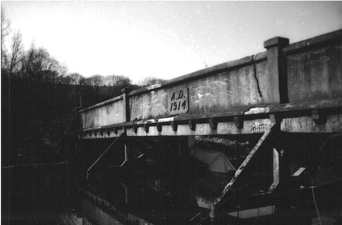
Plate 61: South-facing view showing parapet and parapet sill (10) over cross beams (8) with vertical pillars (9A - 9C) (MF SB06_08)
