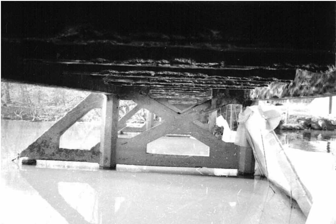
Plate 31: View from the north bank looking south, showing trestles (4a) and (4b) and cut-waters (5) and (5a) (MF SB03_02)
