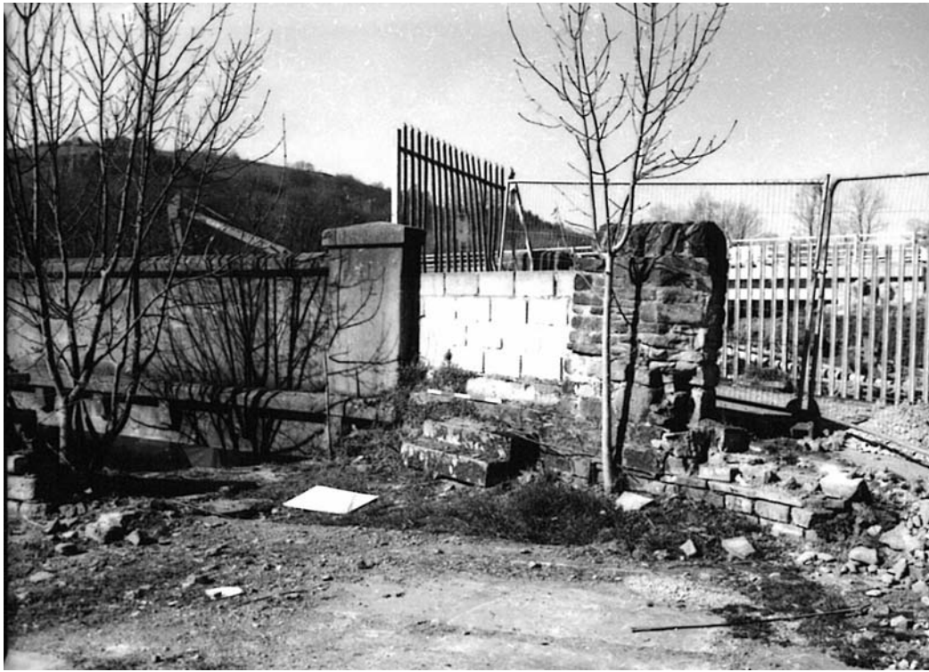
Plate 25: Blocked stepped access (1) and surviving section of eastern wing wall (2) (MF SB05_03)
