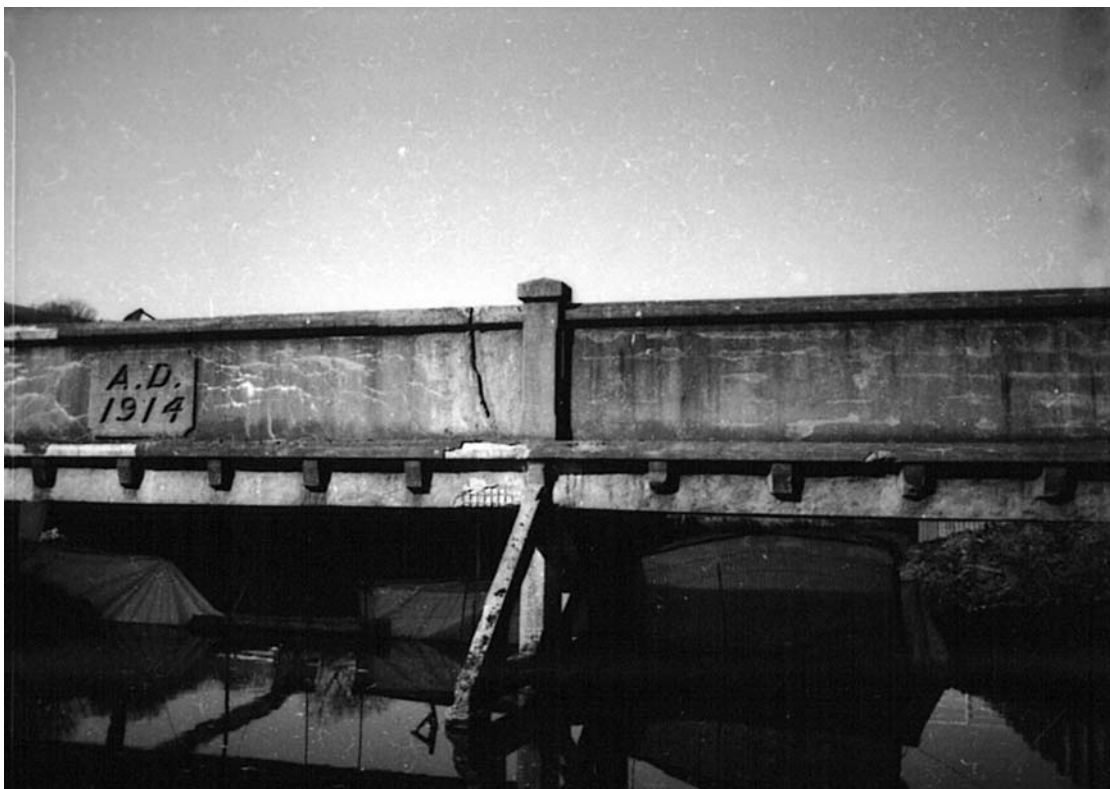
Plate 60: West-facing view showing parapet and parapet sill (10) and over cross beams (8) (MF SB06_04)
