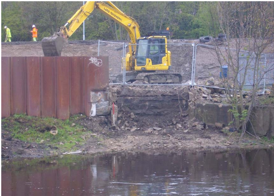
Plate 93: North-facing view showing the remains of the northern abutment (3) following the main phase of demolition (IMG_8751)
