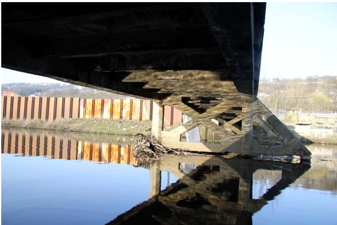
Plate 48: North-facing view beneath bridge showing trestles with diagonal internal bracing (4b) and (4a) and cut waters (5a) and (5) (IMG_2415)
