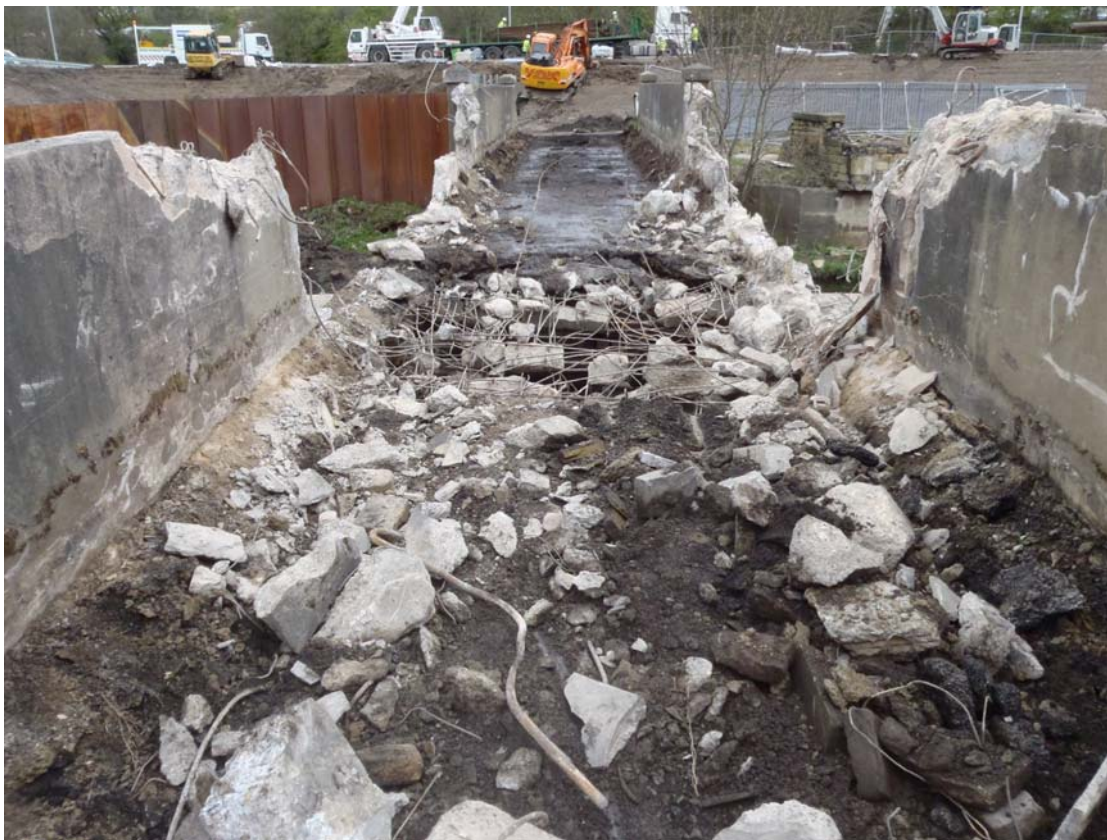
Plate 86: North-east-facing view across the bridge deck ,showing reinforcing in the deck and parapet walls (P3020744.JPG)
