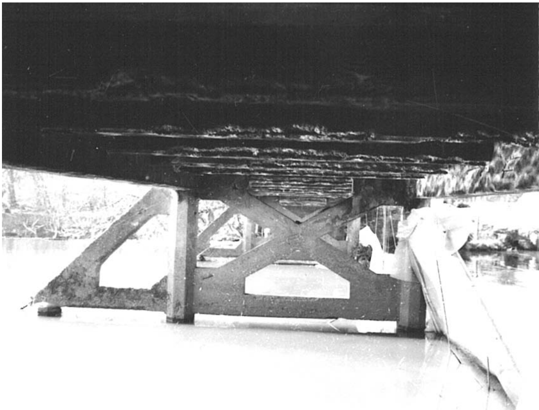
Plate 30: View from the north bank looking south, showing trestles (4a) and (4b) and cut-waters (5) and (5a) (MF SB03_01)
