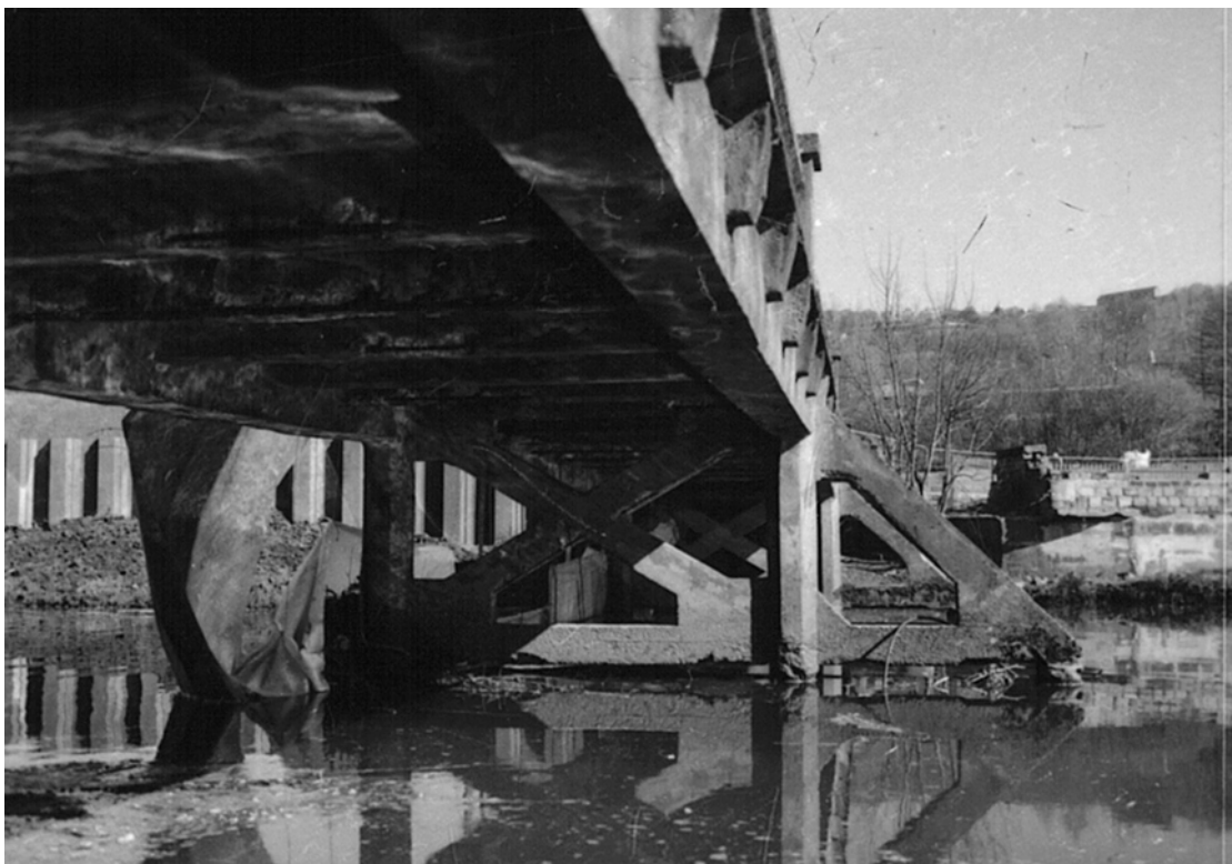
Plate 52: North-facing view showing trestles with diagonal internal bracing ( 4b ) and ( 4a ), and cut-waters ( 5a ) and ( 5 ) (MF SB02_10)
