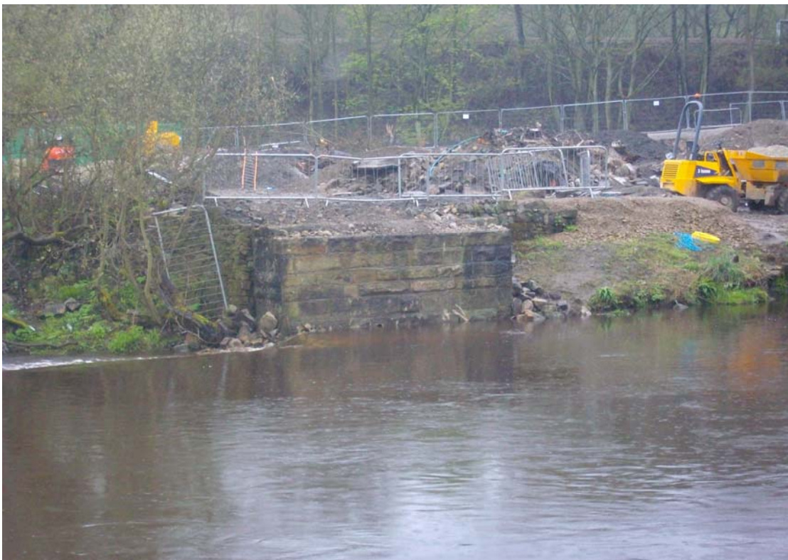
Plate 90: South-facing view across the river Calder showing southern abutment after the completion of the demolition process (IMP_8733)
