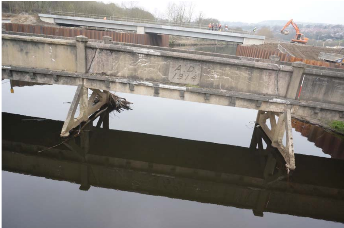
Plate 39: South-east-facing bridge elevation and trestles (4a) and (4b) ; also showing cut-waters (5) and (5a) (DSC00489)
