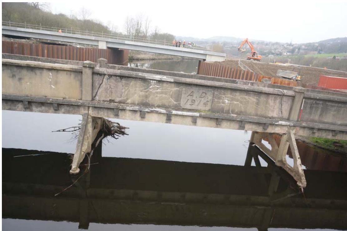
Plate 40: South-east-facing bridge elevation and trestles (4a) and (4b) ; also showing cut-waters (5) and (5a) (DSC00490)
