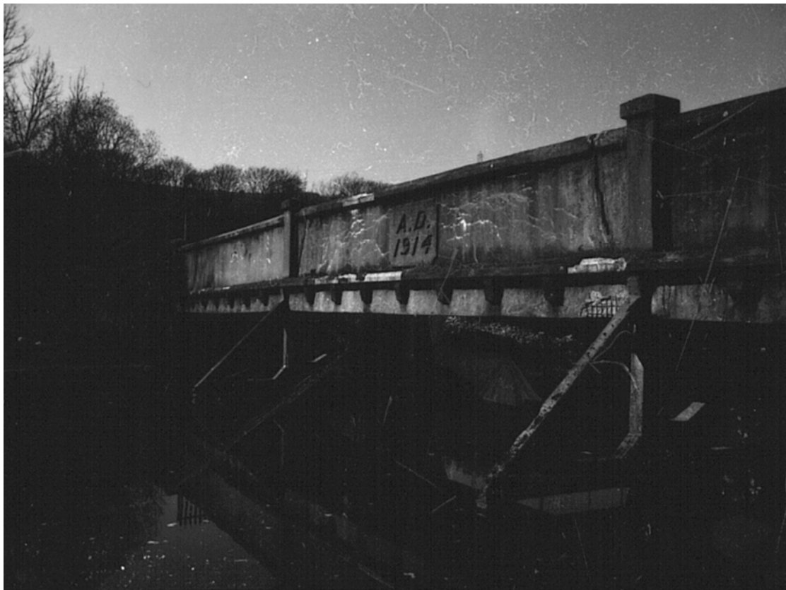
Plate 62: South-facing view showing parapet and parapet sill (10) over cross beams (8) (MF SB06_09)
