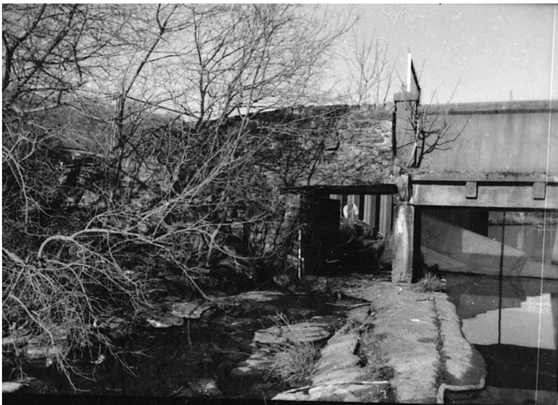
Plate 71: View from the edge of the weir showing wing wall (11), abutment (12) and trestle (4c) (MF SB03_08)
