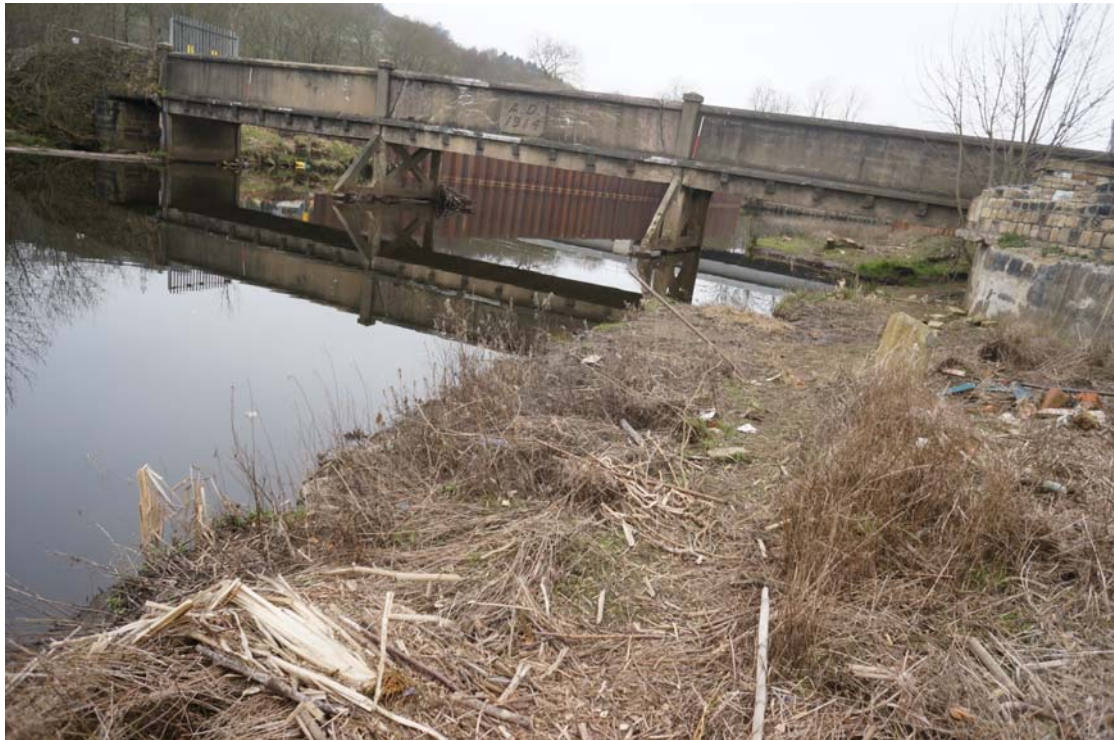
Plate 45: South-east facing bridge elevation showing trestles (4a) (4b) and (4c); also showing cut-waters (5) and (5b) (DSC00507)
