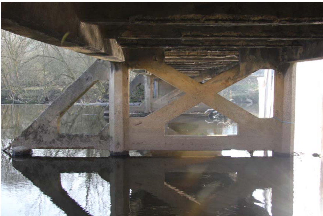
Plate 36: View from the north bank looking south, showing trestles (4a) and (4b) (IMG_2396)
