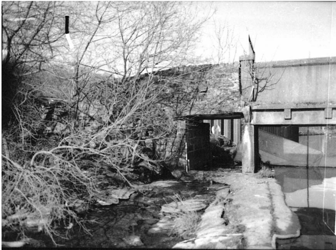
Plate 70: View from the edge of the weir showing wing wall (11), abutment (12) and trestle (4c) (MF SB03_07)
