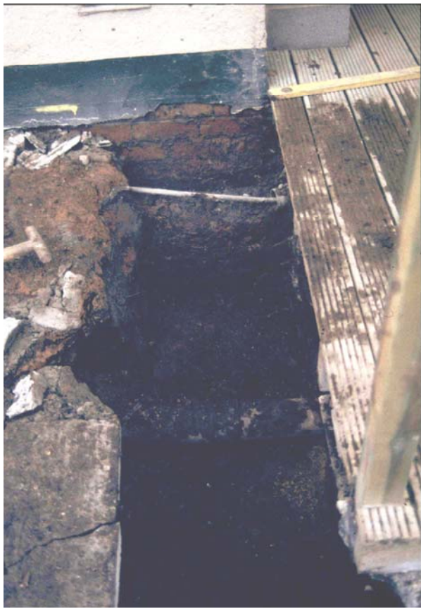
Plate 2: West end of the trench, showing the current foundations of Ladyewell House
