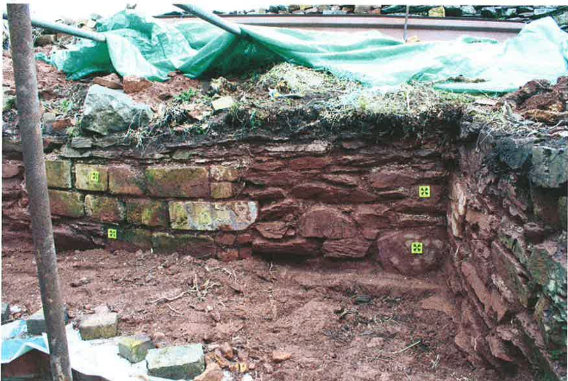
Plate 2: Remodelled section of wall in central part of eastern elevation, also showing the top of the stone slab bridging the corner of the stack
