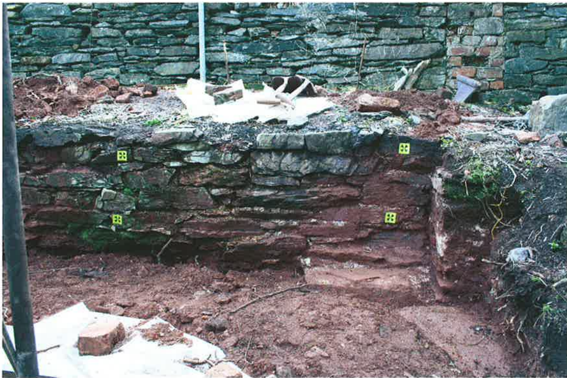
Plate 3: South elevation of the stack, with projecting stone slabs at western end
