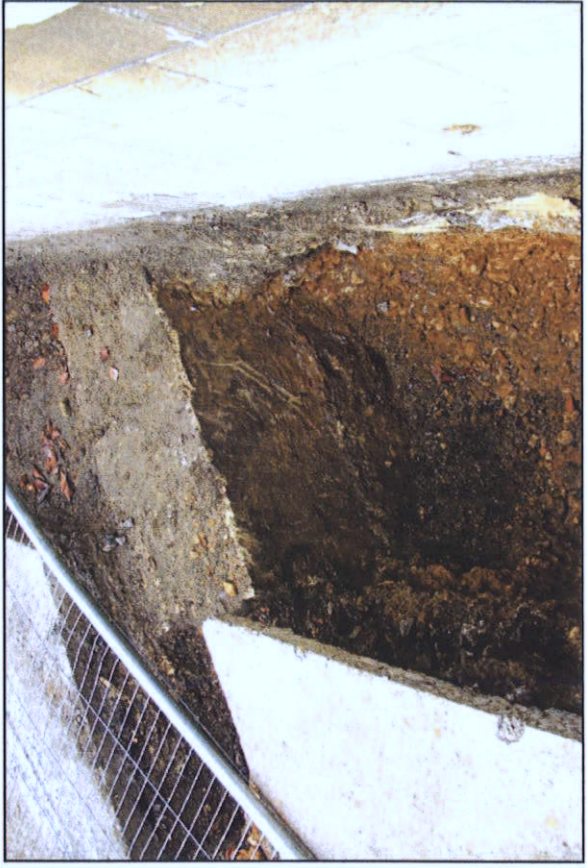
Plate 16: Block 2, foundation of former yard wall below later extension looking south west.
