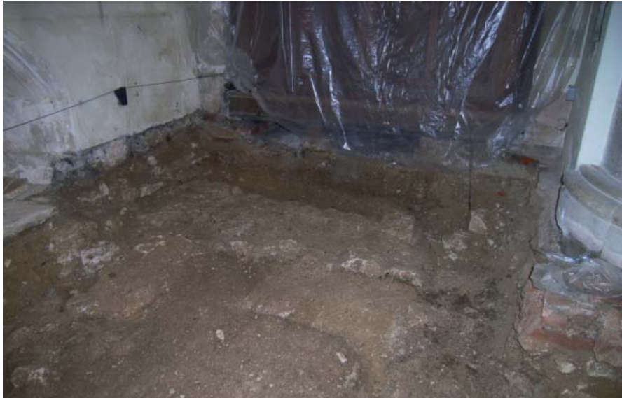
Plate 11: Footings of a wall at the east end of the north aisle (2027)
