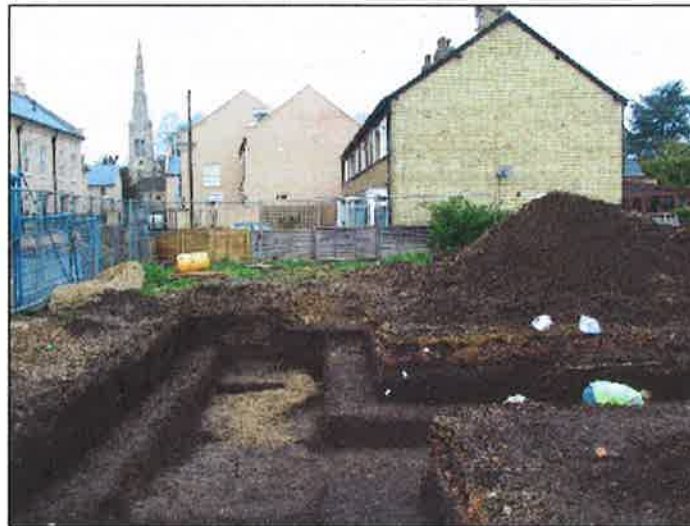
Plate 1: Trenches 1 and 2a under excavation with the former Permanex site and All Saints church in the background (looking west)
