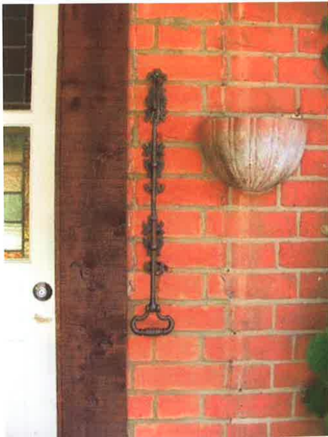
Plate 6: View inside the porch, showing alteration to brickwork and original iron bell pull
