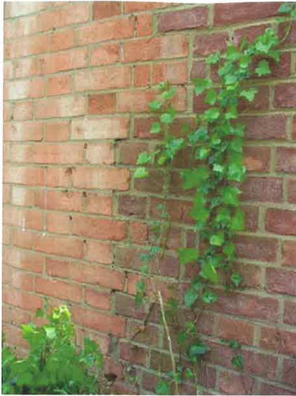
Plate 9: View of the join of the extension brickwork (right) keyed with original brickwork, looking northeast
