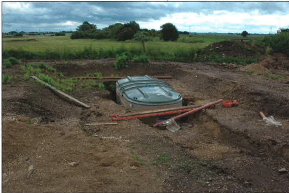
Plate 1: Watching brief trench following insertion of tank (Copyright Ben Robinson, by permission)
