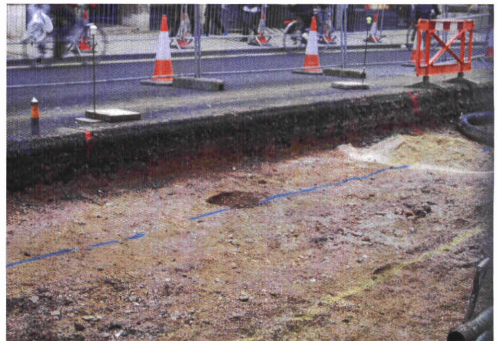
15) Void crossed by water leakage → S
