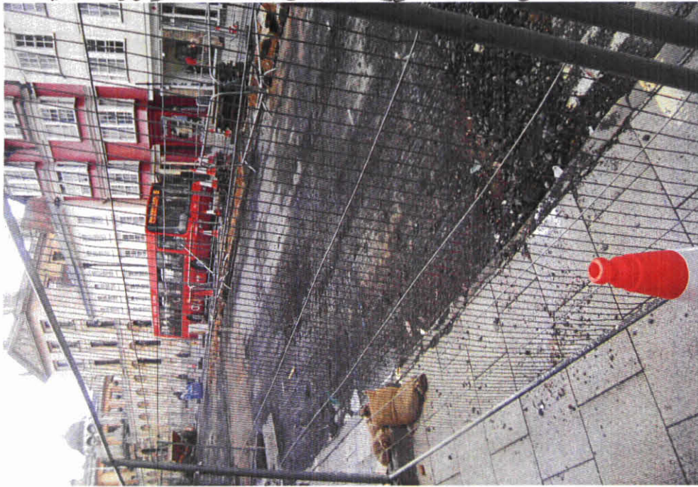
26) Removal of tarmac, south side of High St. Between Queens College + Longwalk St. → N
