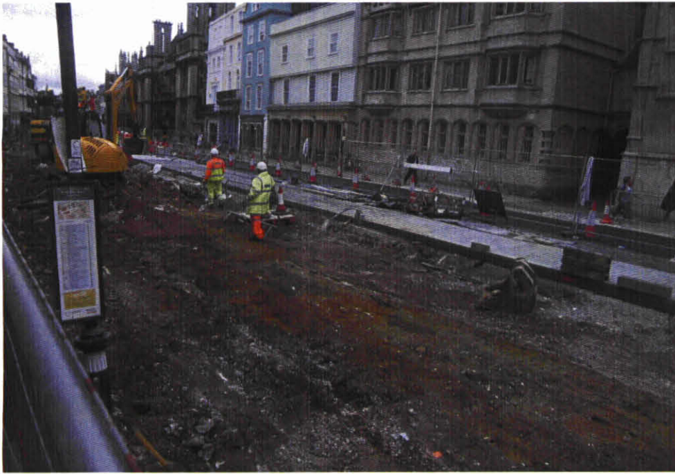
6) West Eastbound carriage way, access collapse → E
