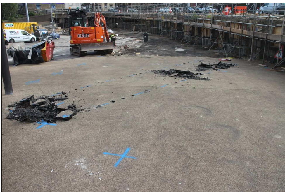
Plate 6: Location of Trench 3 prior to excavation showing the original trench location in the foreground of the image, the 2m gap visible towards the far end of the trench.
