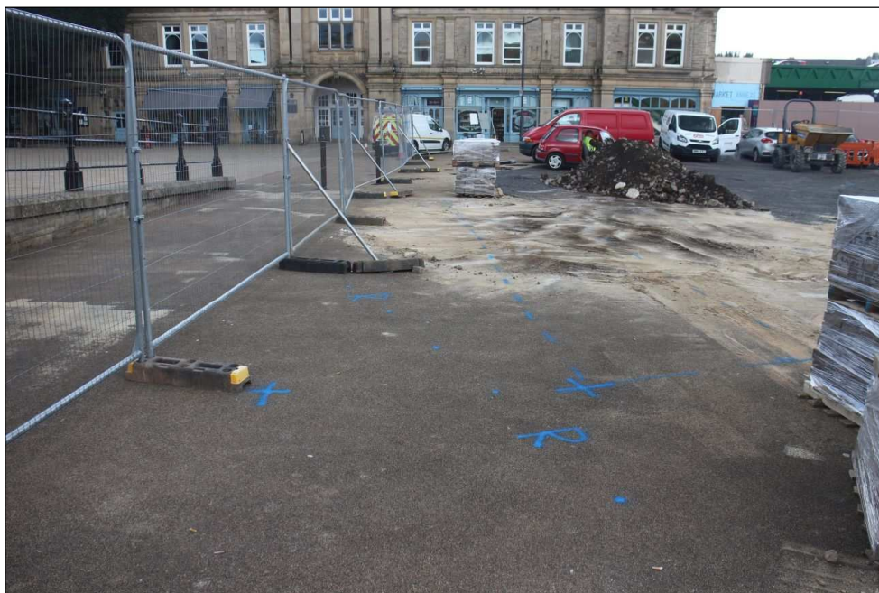
Plate 4: Location of Trench 2 prior to excavation showing original trench location to the left of the image with the dotted line showing the presence of an electric cable detected in Radio mode on the CAT, drainage visible at the northern end of the trench.
