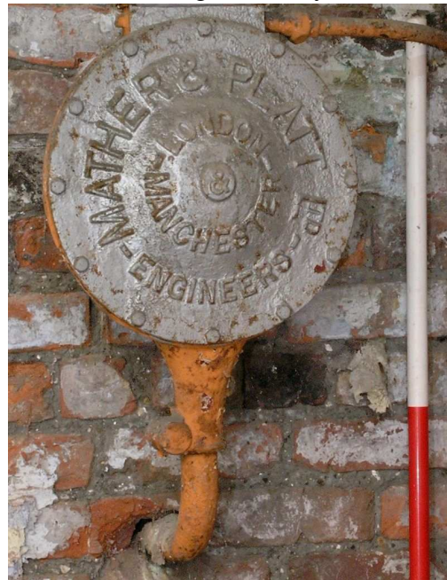
Plate 16: Sprinkler system diaphragm
