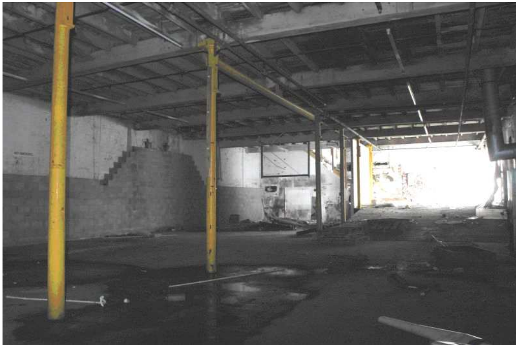
Plate 9: View looking north-east across the ground floor, with the cinder block wall to the left
