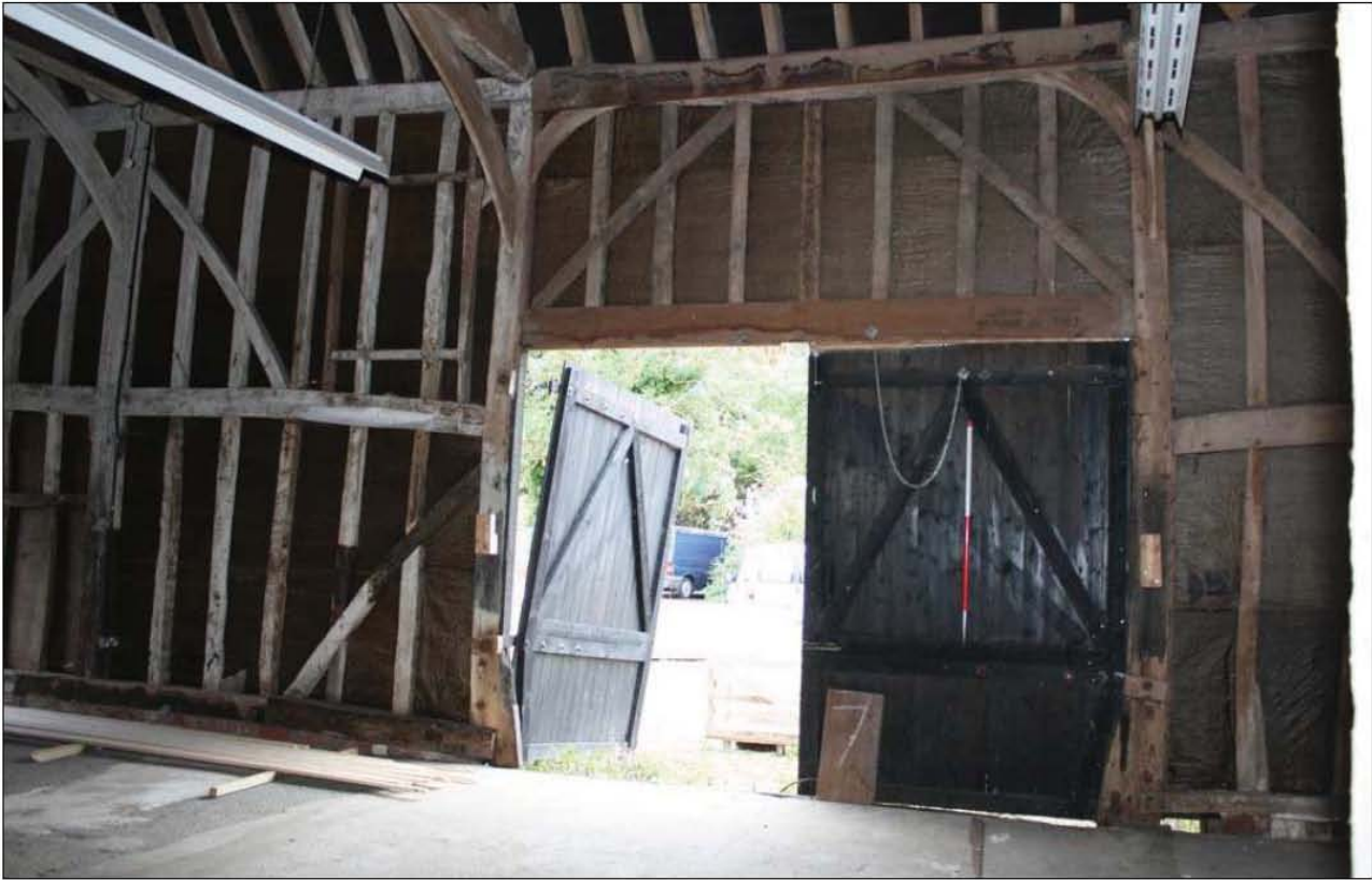
Plate 75: Evidence of blocked ventilation hole above left of doors, phase 1 barn
