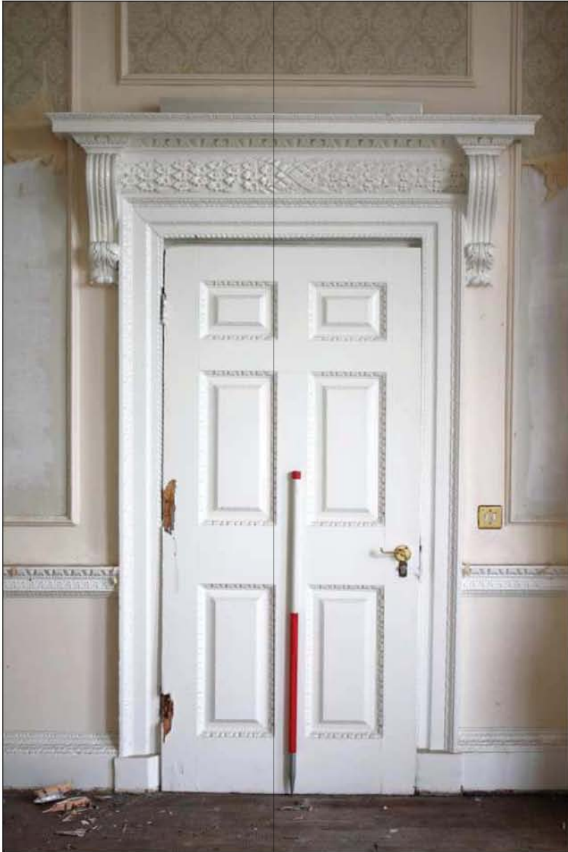
Plate 22: Detail of door, G13
