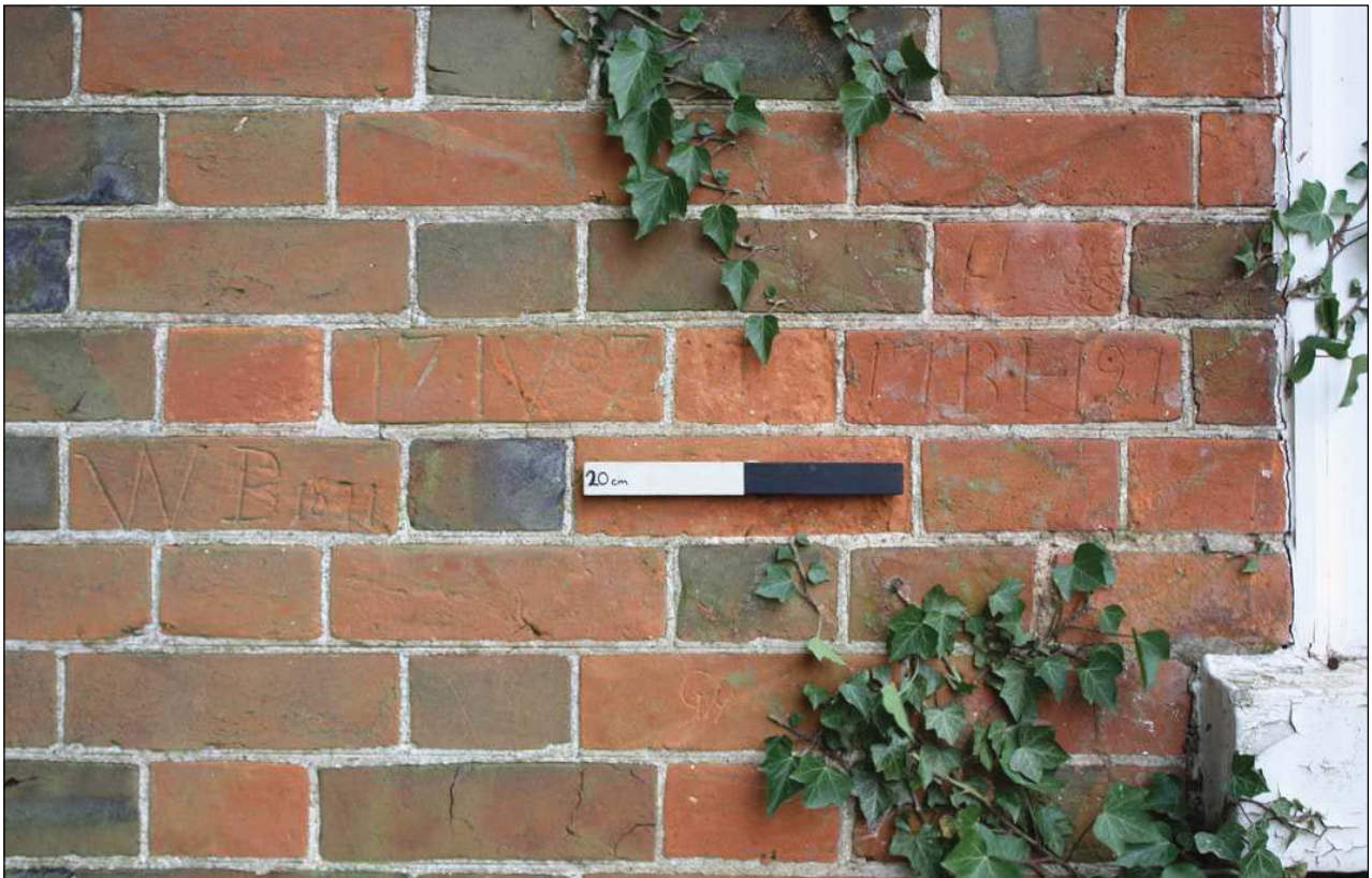
Plate 3: Dated graffiti on exterior wall of G2
