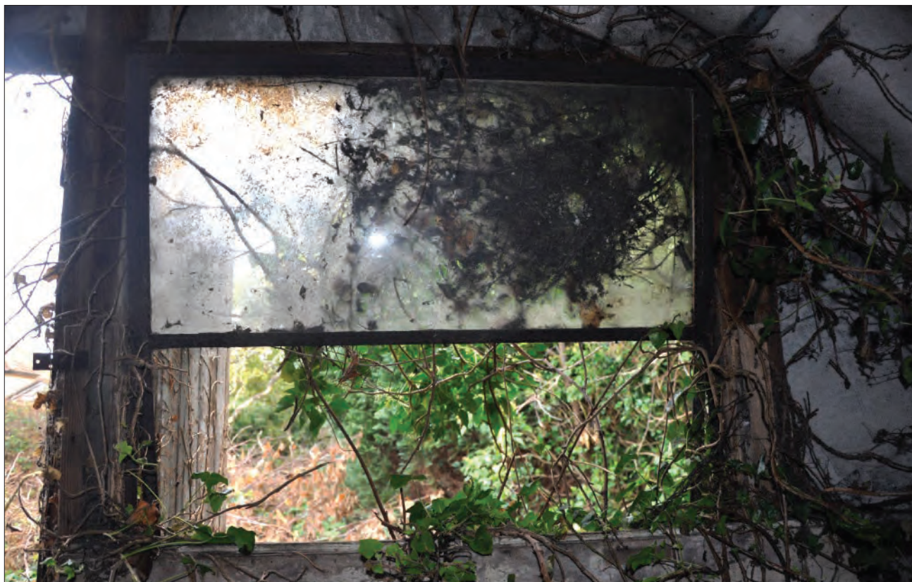
Plate 12: Lefthand window on northeast facing elevation, viewed from the interior, showing surviving glazing
