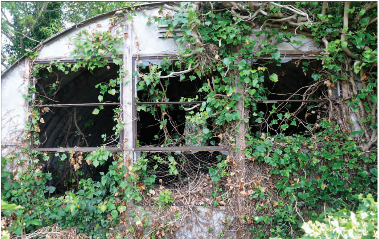
Plate 17: Detail of southwest facing elevation showing chicken wire
