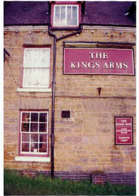
Plate 2: Detail of front of pub showing blocked window
