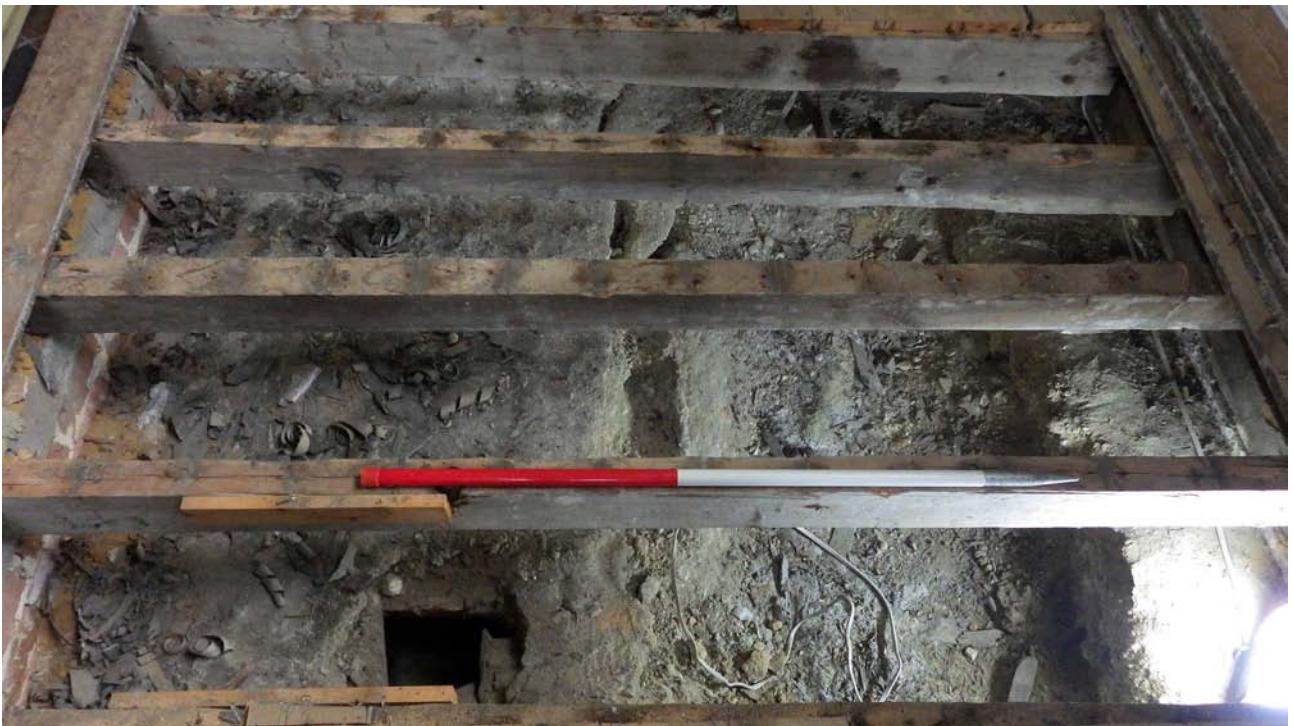
Plate 4: Areas of subsidence visible beneath timber platform of test pit 6
