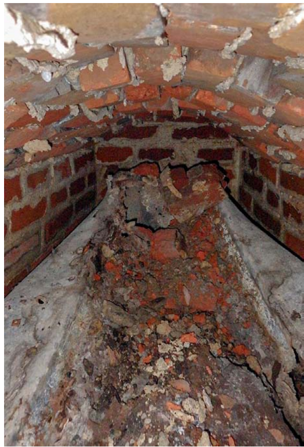
Plate 5: View to east inside the partially collapsed brick vault of test pit 6
