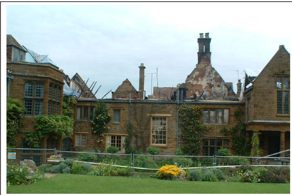
Plate 3: View north east - fire damage to roof on south west wing.
