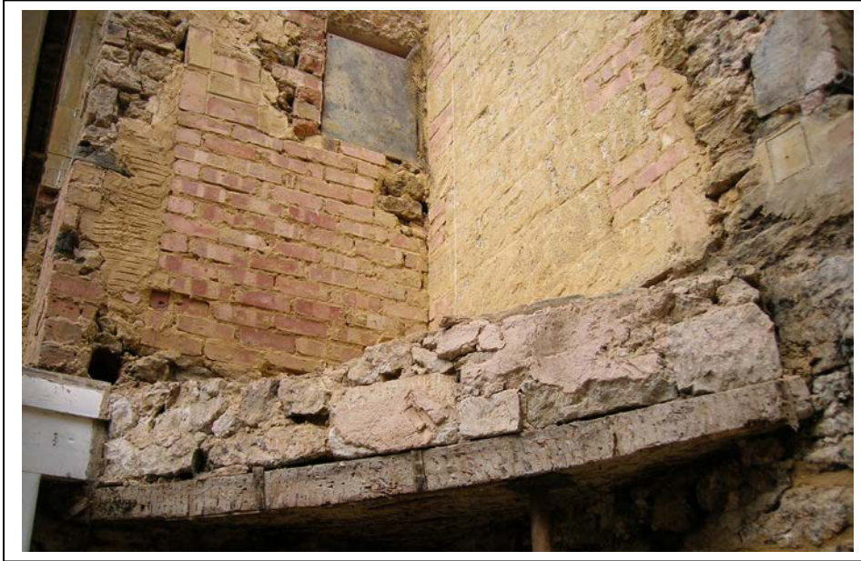
Plate 9: View west - chimney base with brick repairs to first floor walls.
