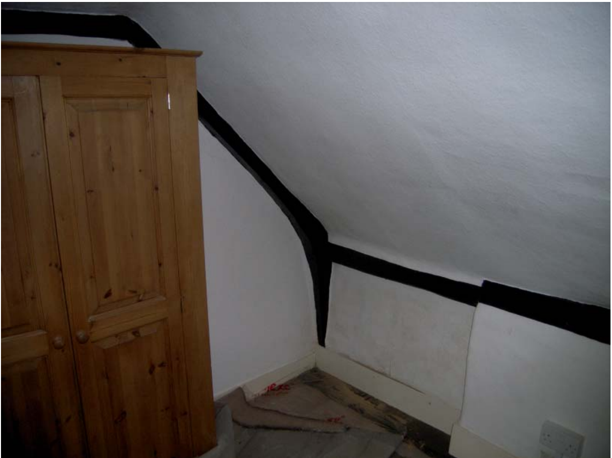
Plate 34: 1st floor room looking SW showing crack
