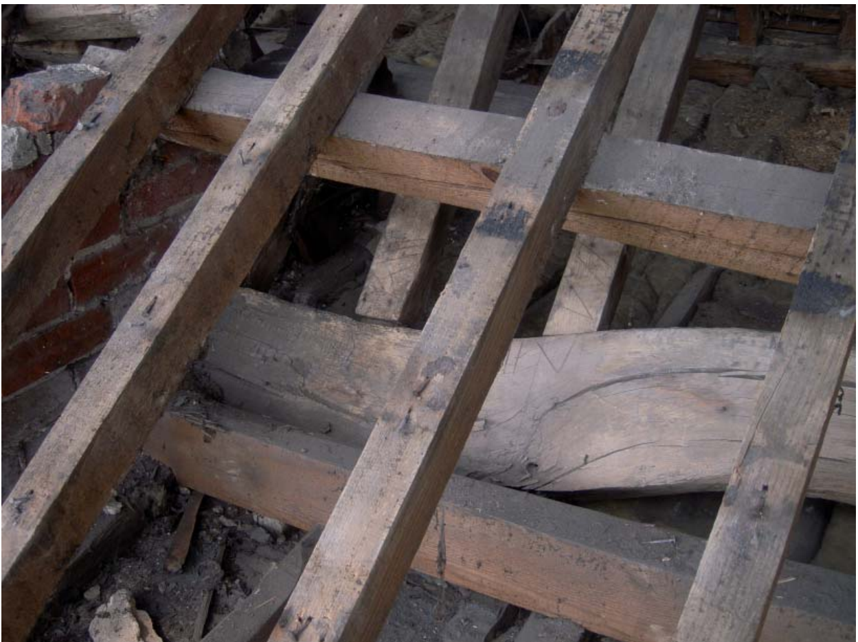
Plate 22: Primary purlin in east slope (Bay 3) below secondary rafters from higher roof line
