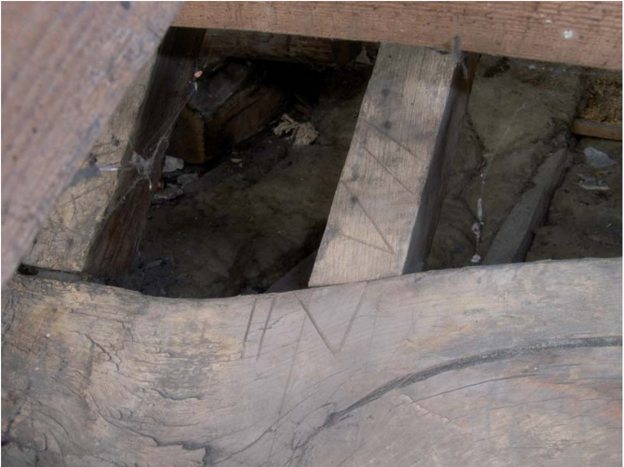
Plate 23: Carpenters marks in primary purlin and rafter below secondary higher roof line
