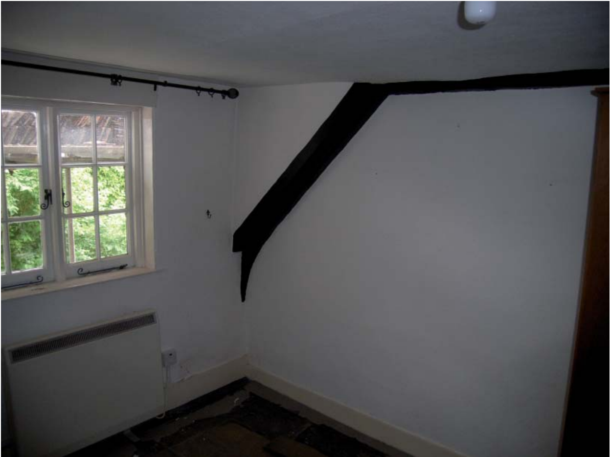
Plate 33: 1st floor room looking SE showing crack
