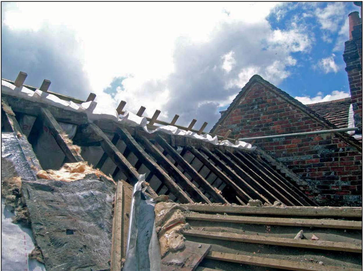
Plate 14: View of timbers forming rear pitch of main roof (looking west to No.50)
