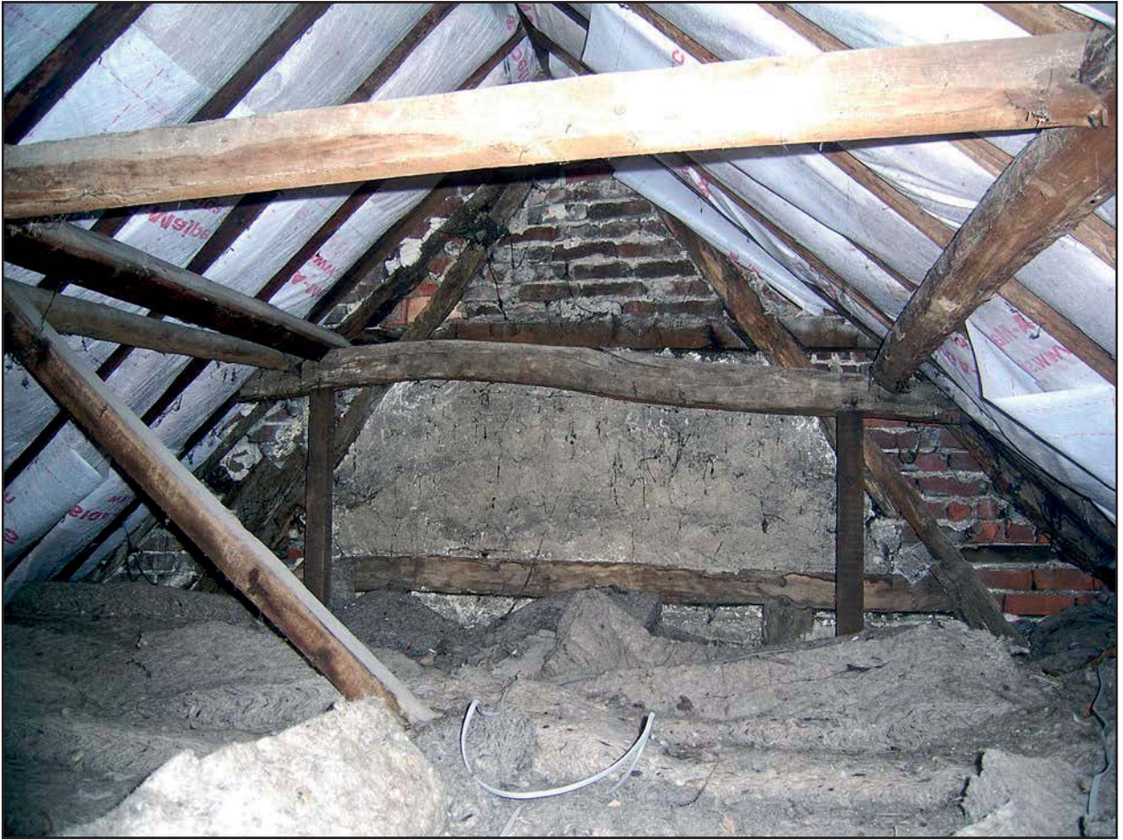
Plate 17: View of gable wall to west of roof (Looking west in No.49 towards wall of No.50)
