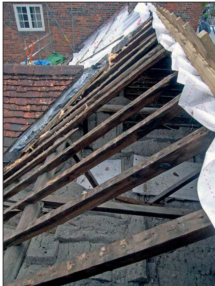
Plate 12: View of timbers forming rear pitch of main roof (No.49 looking east)
