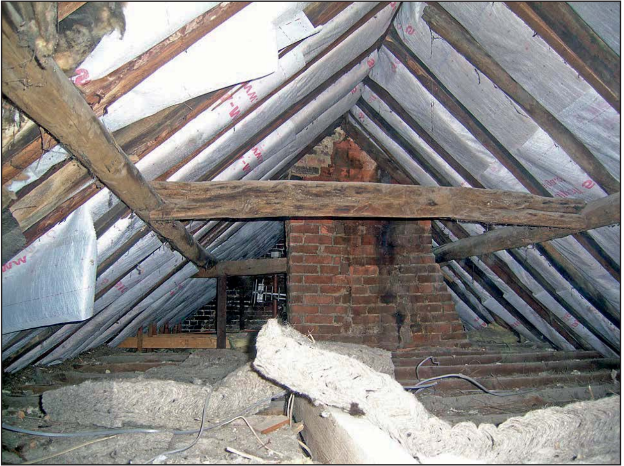
Plate 15: Internal view of roof timbers facing east (No 49 looking east towards No.48)
