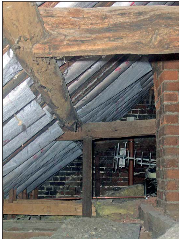
Plate 16: Detail of truss and purlin in eastern part of roof (Clasped purlin in 48 looking E)
