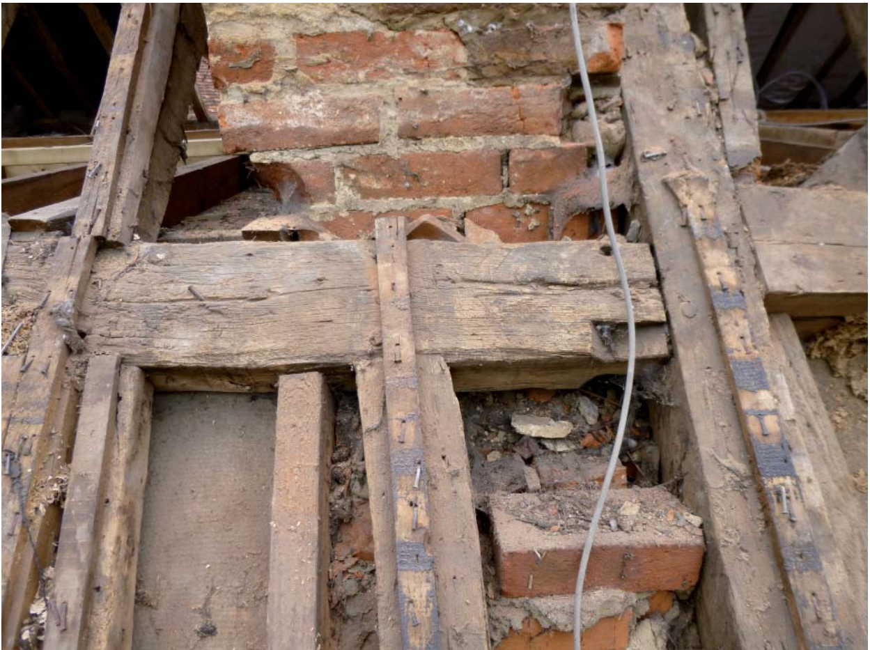
Plate 20: Degraded Carpenter's Marks on south slope
