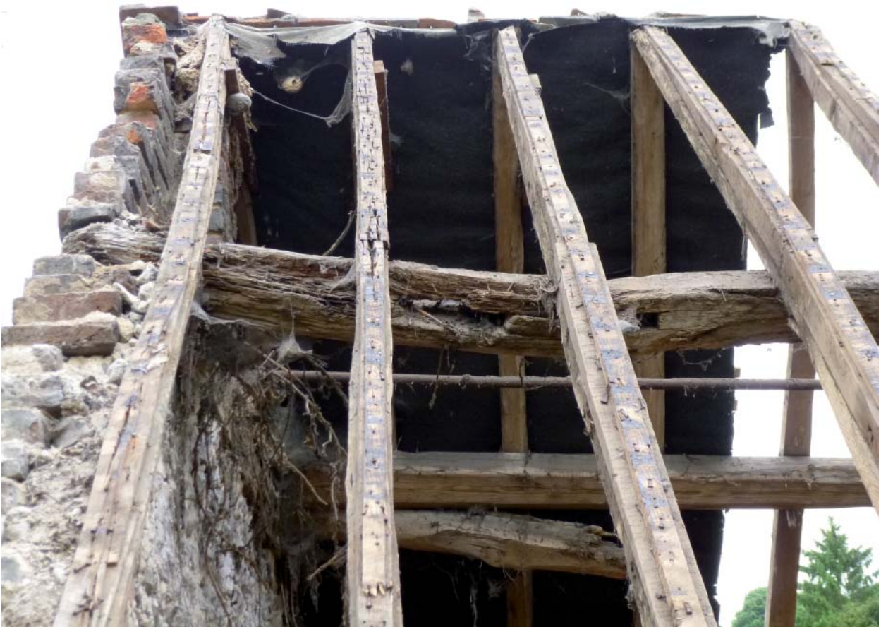
Plate 14: Rotted length of north slope upper purlin
