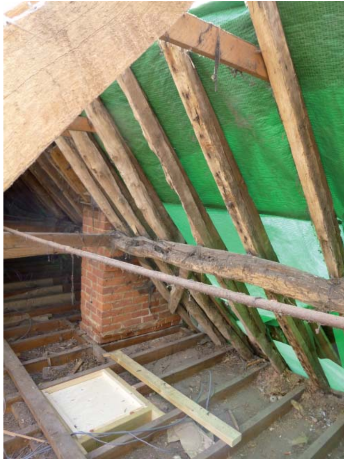
Plate 11: Reinforcing bar visible in the roof space
