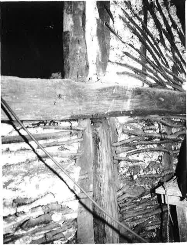
DETAIL OF WATTLE AND DAUB INFILLING TO END TRUSS OF MAIN BLOCK NO. 11 R228 N24
