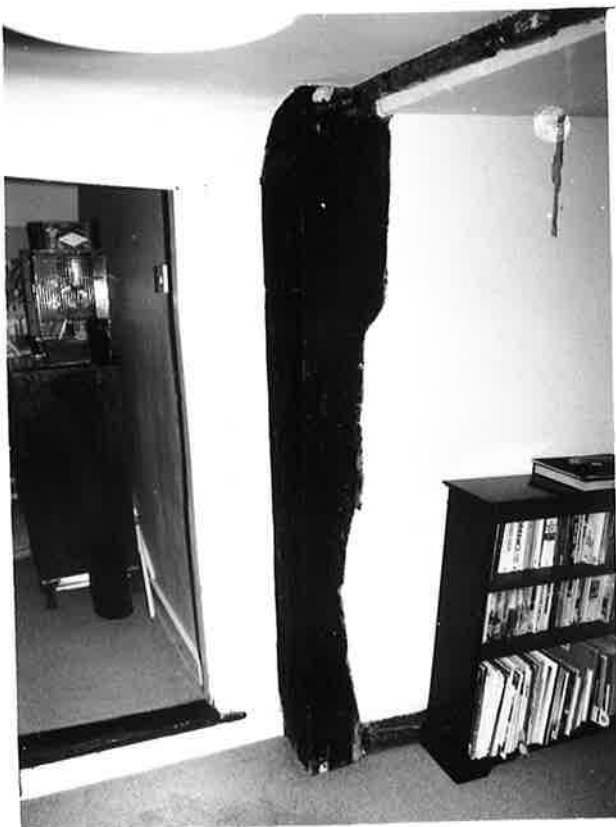
CORNER POST OF 'BUTCHERS RANGE' VIEWED FROM LANDING ROOM K, NO. 11. R 228 N 17.
