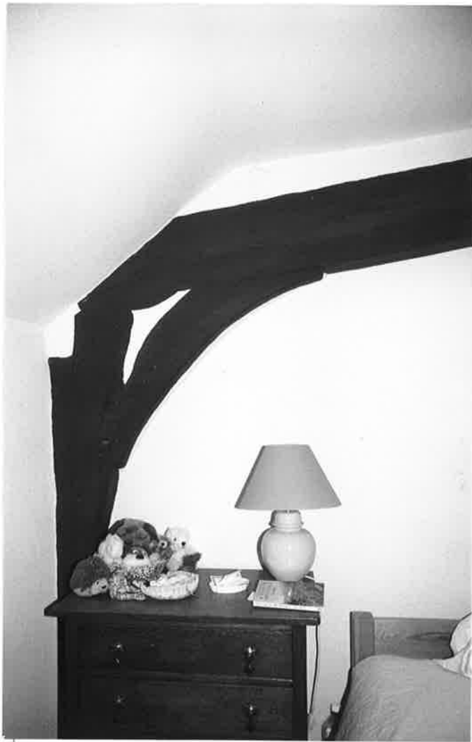
DETAIL OF MAIN POST AND TIE-BEAM TO SOUTH - WEST, ROOM E, NO. 12. R 179 N2.
