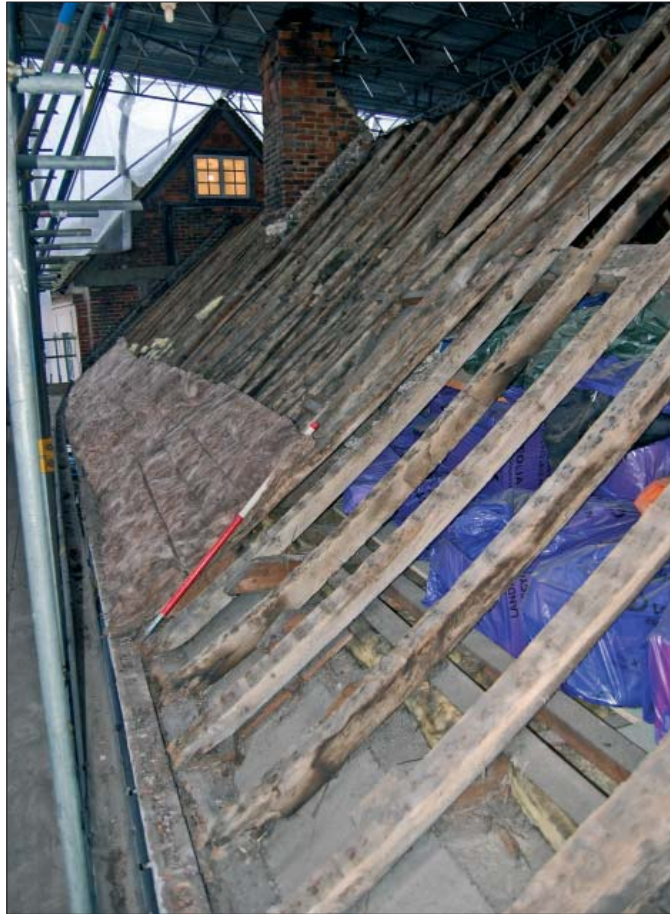
Plate 1: View of no. 11 and 12 roof High Street frontage following removal of tiles
