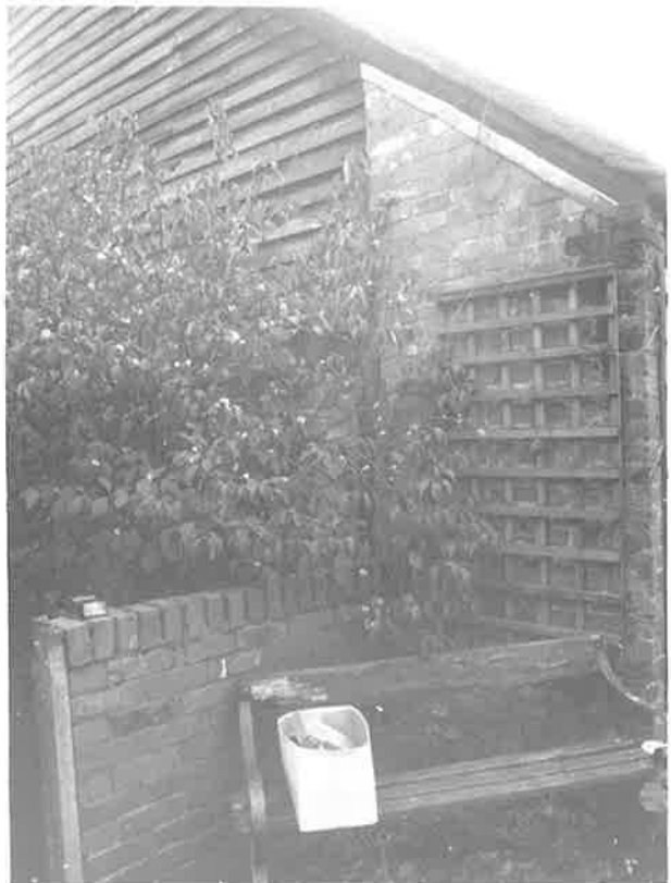
NORTH GABLE OF BUILDING NO. 2, NO. 14 ; ORIGINAL END WALL OF NO. 13 R228 N3
