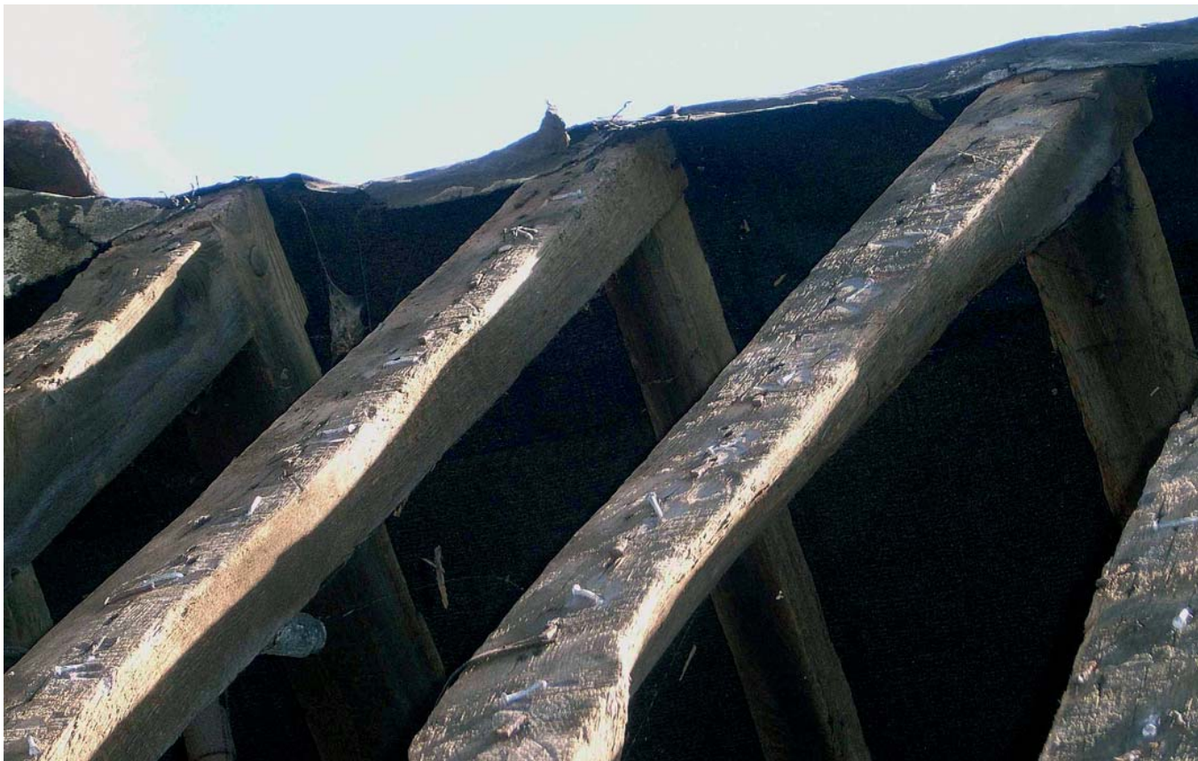
Plate 9: Example of rafter joints at the apex, west slope of west wing
