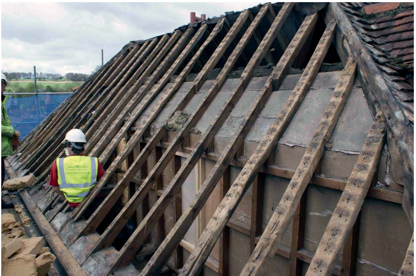
Plate 18: Replacement lengths of rafters to former dormer in the south slope, east end of the south range (courtesy of Gary Marshall)
