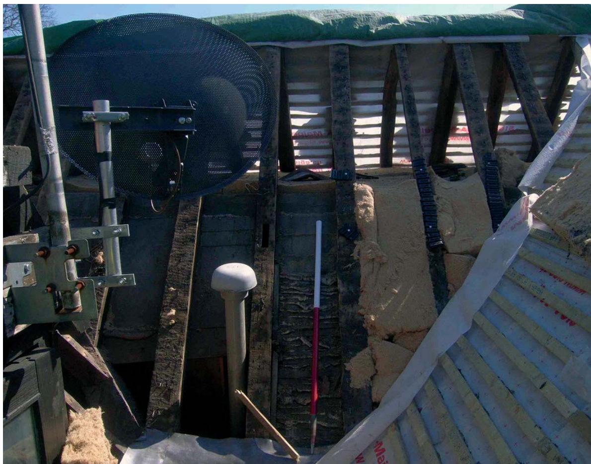
Plate 12: Empty mortice in the principal rafter in the north slope of the south range
