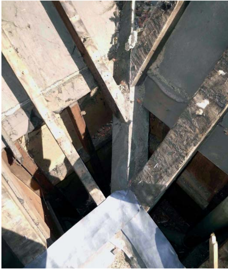
Plate 7: Leadwork in the valley obscuring the rafter ends
