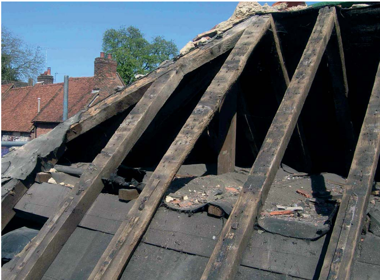
Plate 11: Example of the pegs attaching the rafters to the purlin, west slope of the east wing
