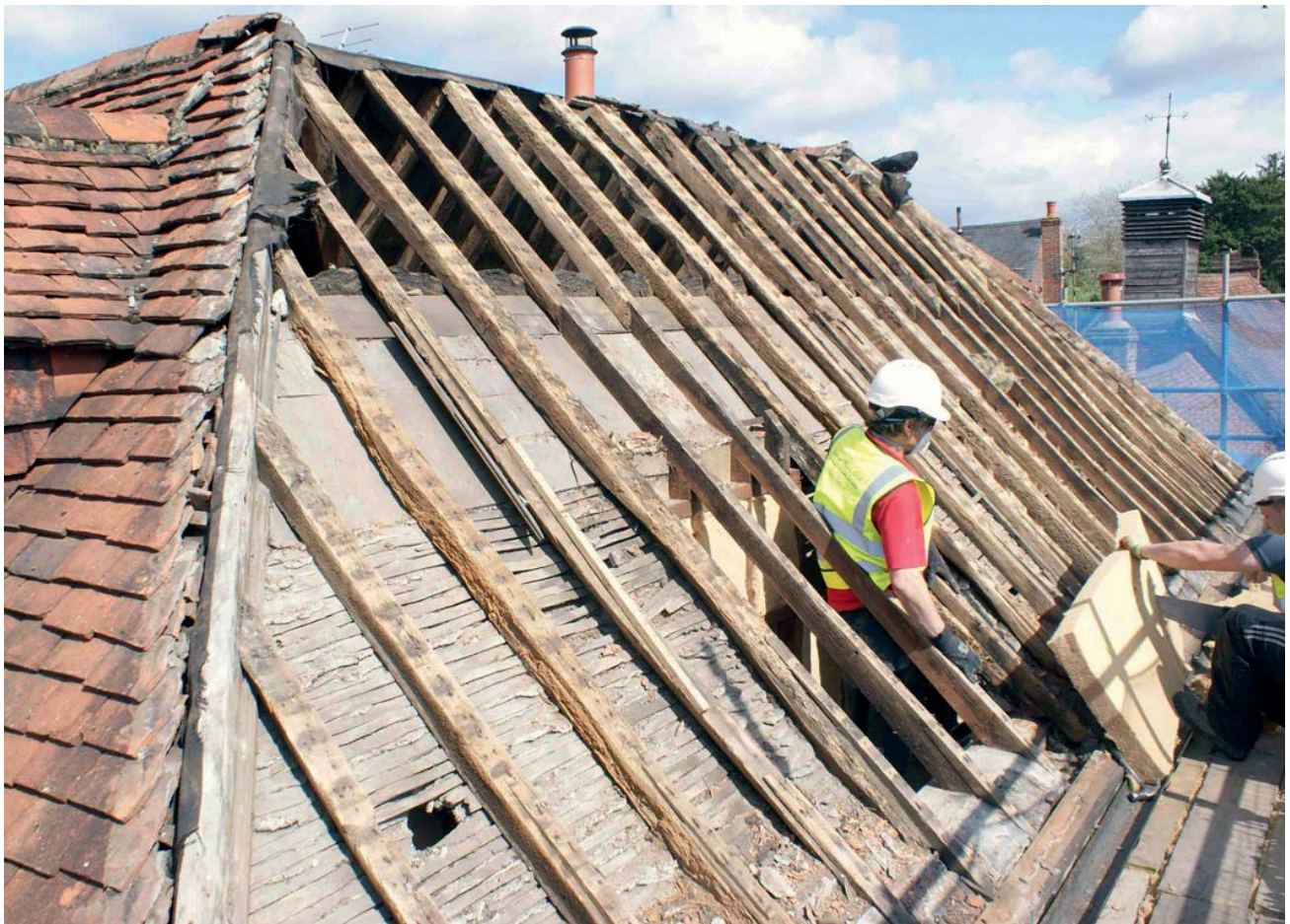
Plate 17: Replacement lengths of rafters to former dormer in the south slope, west end of the south range (courtesy of Gary Marshall)
