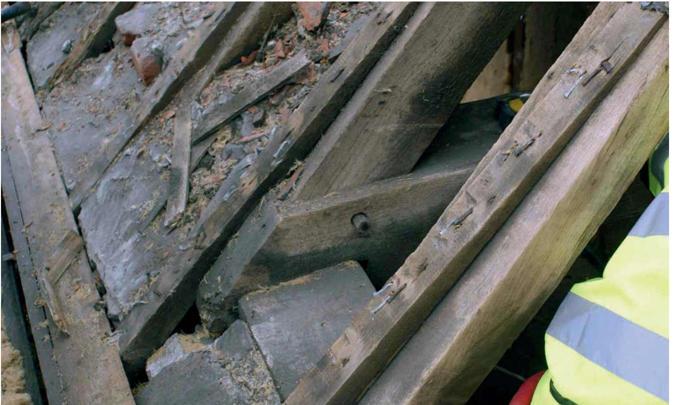
Plate 6: End of the tie beam in the south slope of the south range (courtesy of Gary Marshall)
