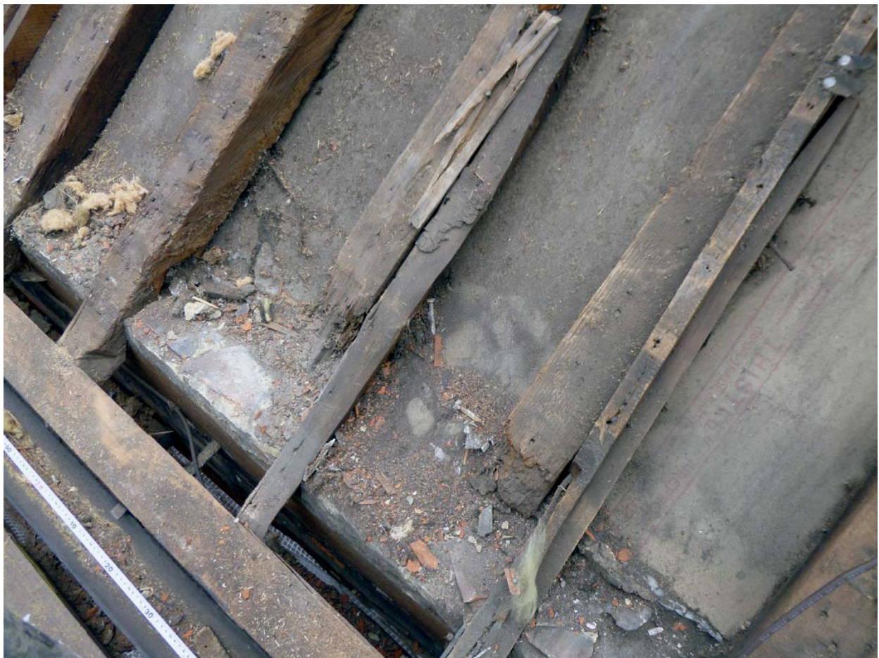
Plate 14: Rot, reinforcement and sprockets, west slope of the west wing
