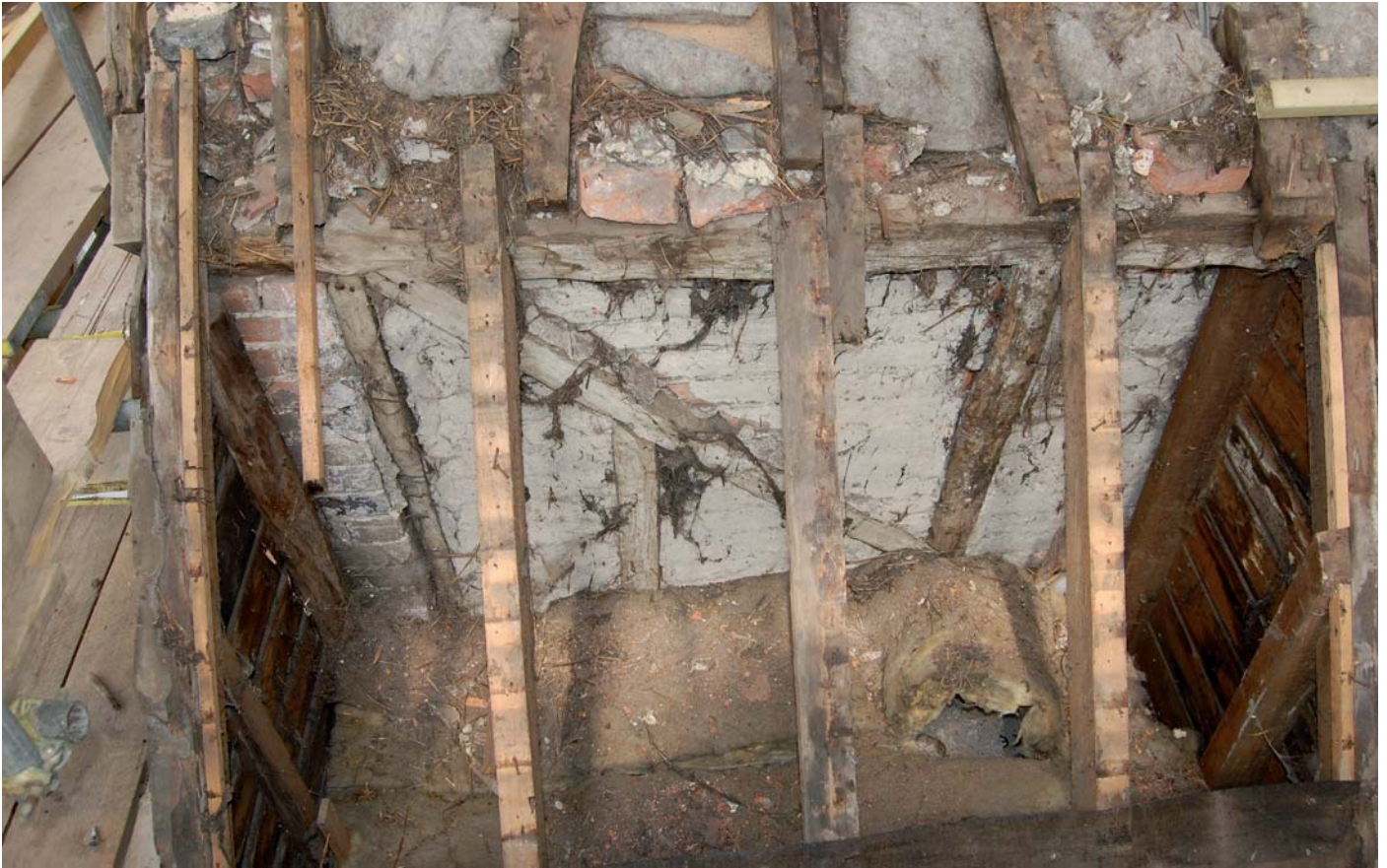
Plate 31: Exposed section of timber framing at west end of south wall (No 30) within outshut
