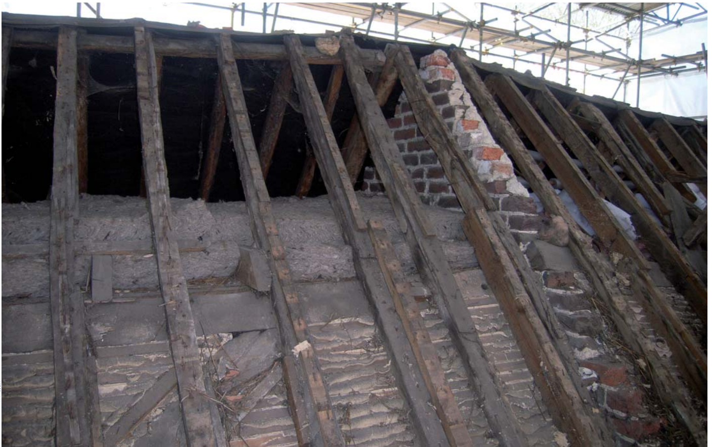
Plate 7: North slope of No 30 showing wind-brace and formerly external face of gable
