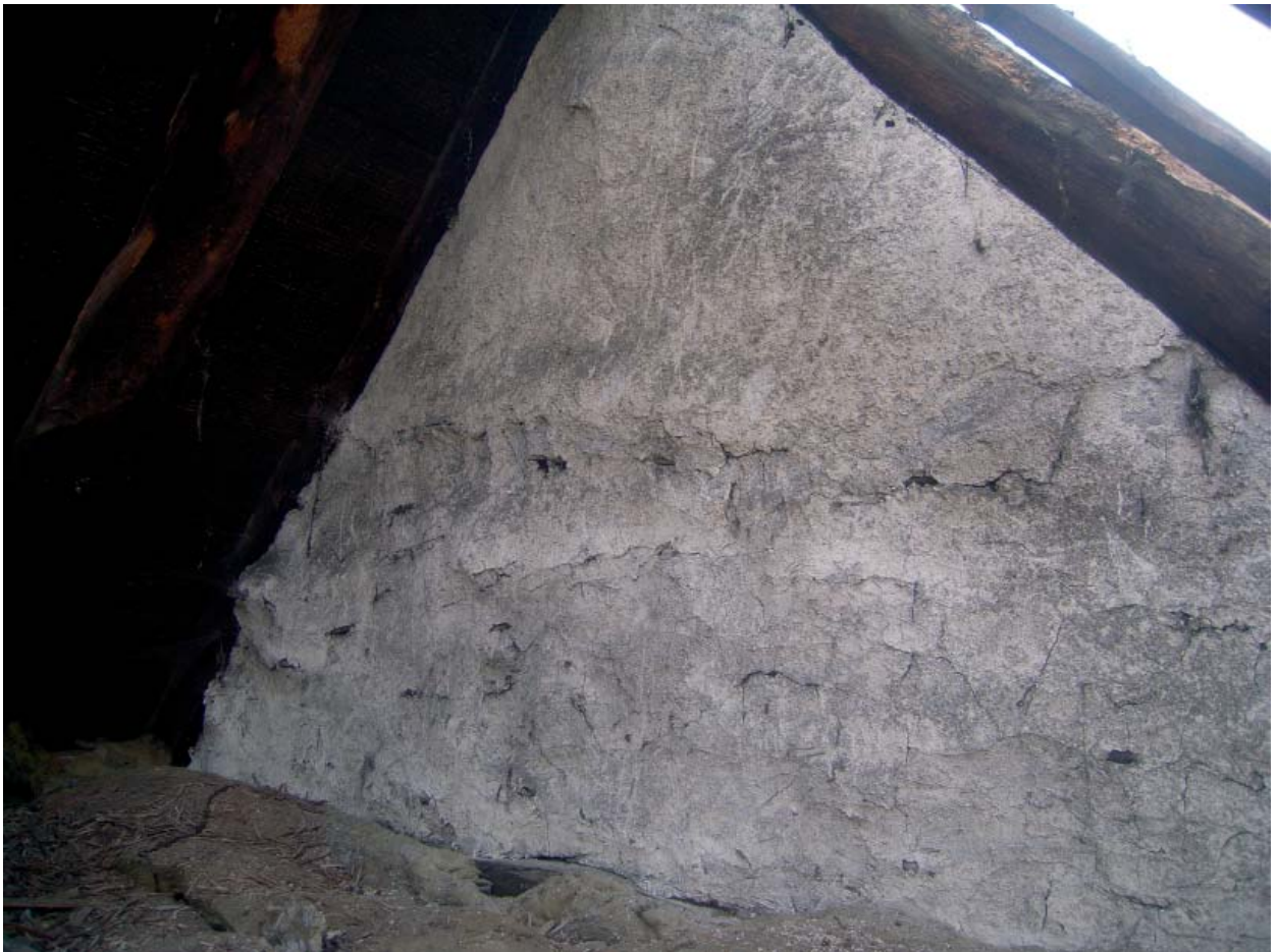
Plate 62: Old plaster, looking west in roof space of No.4 (central truss of Block R)
