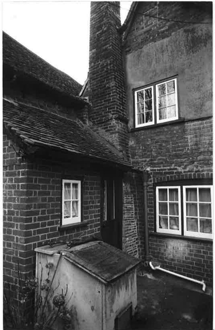
No 5 LEAN-TO M AND REAR WING K, VIEWED FROM SOUTH-EAST. R. 176 N 1A.
