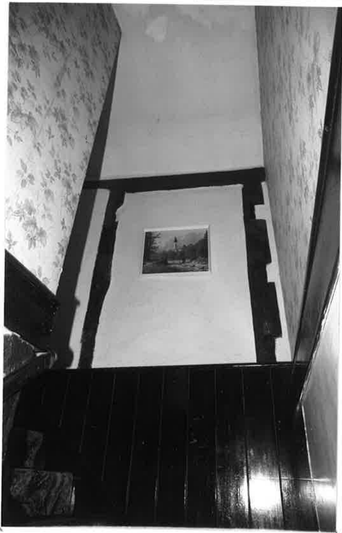
PLANK PANELLING TO SOUTH STAIR WALL, STUDS ABOVE ARE RE-USED TIMBERS. R 176 N12A
