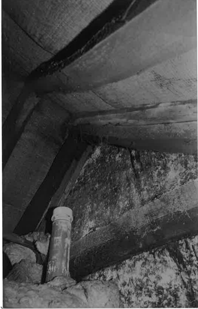
Nº4 HIGH STREET. TRUSS AGAINST GABLE OF BLOCK R, LOOKING WEST. R178 N1A.
