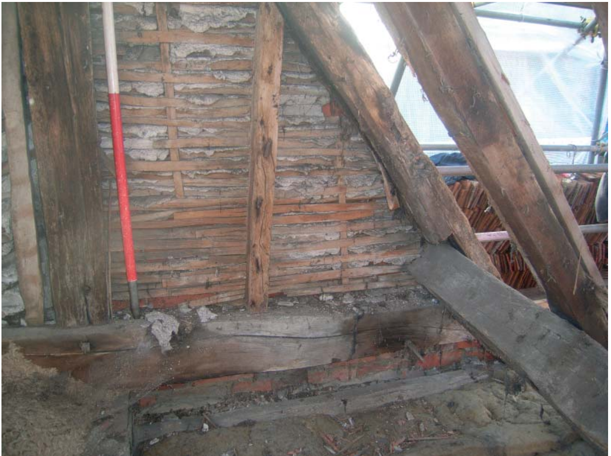
Plate 18: Lath and plaster at south end of No. 4
