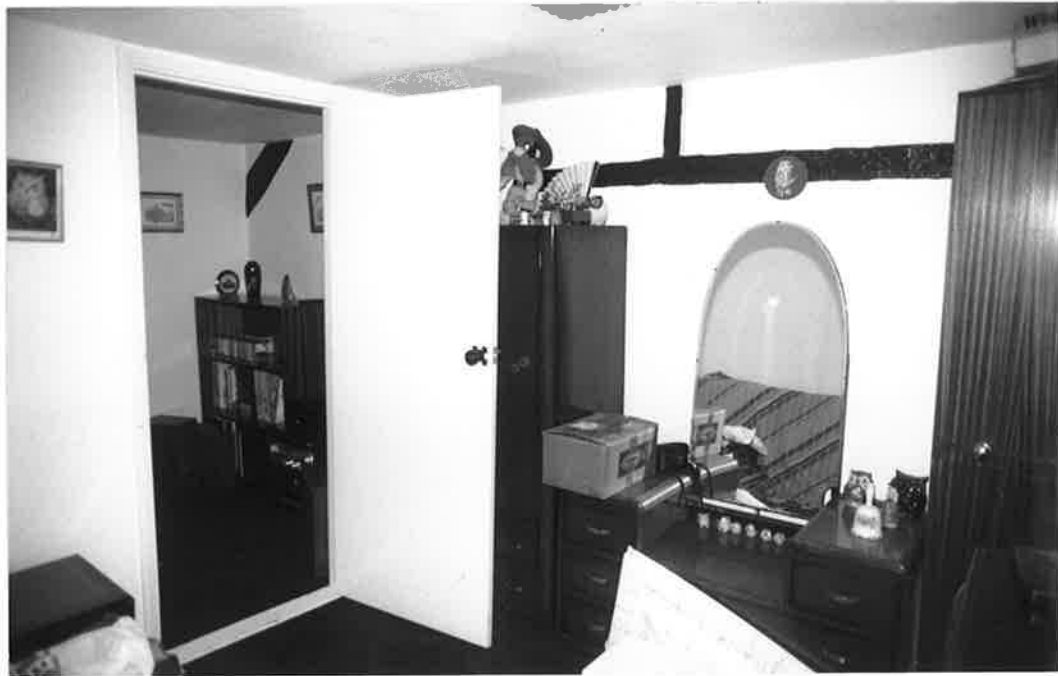
TIMBER FRAMING TO EASTERN END WALL, VIEWED FROM ROOM B. R173 N36A.
