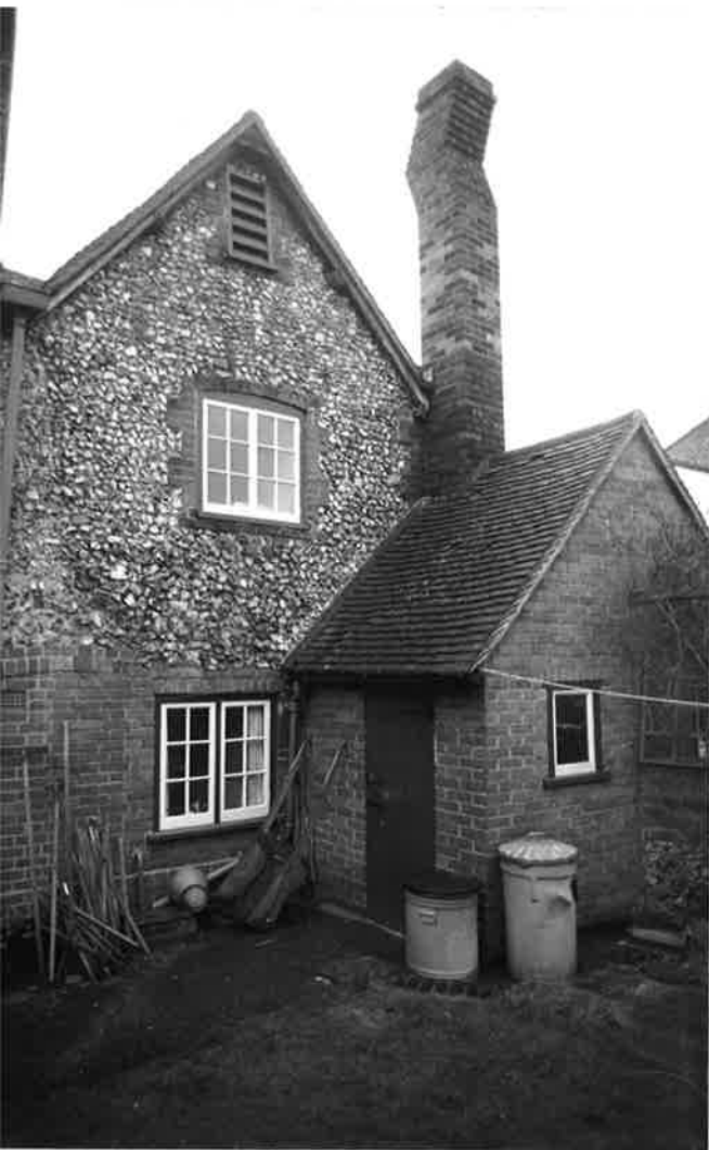
REAR WING I AND SHED G, NO 7 VIEWED FROM SOUTH-WEST R 175 N 16
