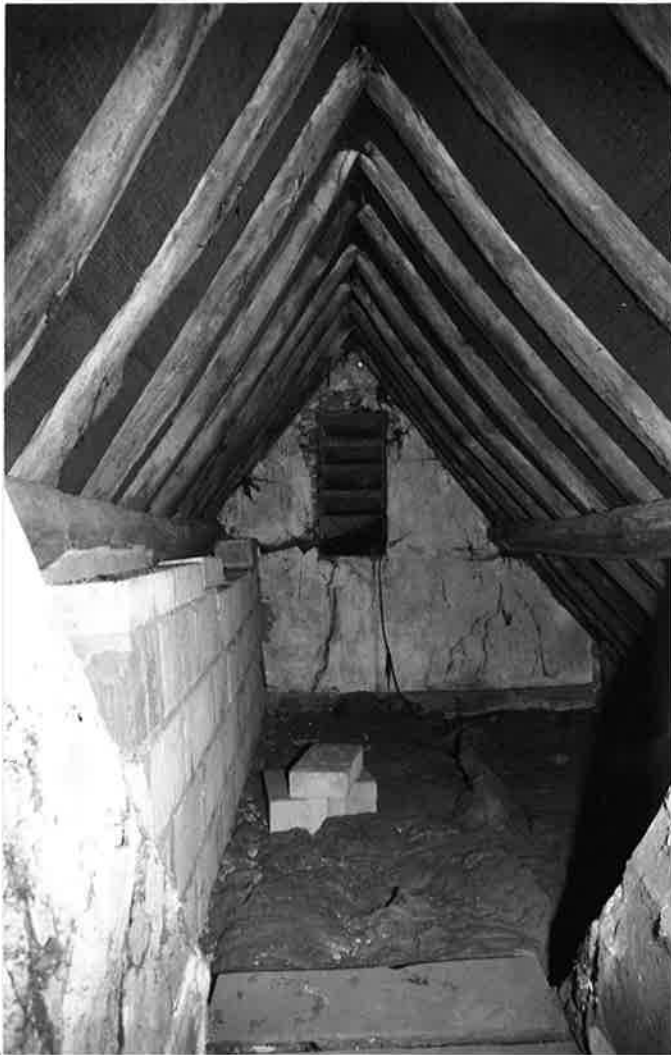
Nº7 HIGH STREET - INTERNAL ROOF STRUCTURE, SOUTH- EASTERN WING, LOOKING SOUTH. R175 N2.
