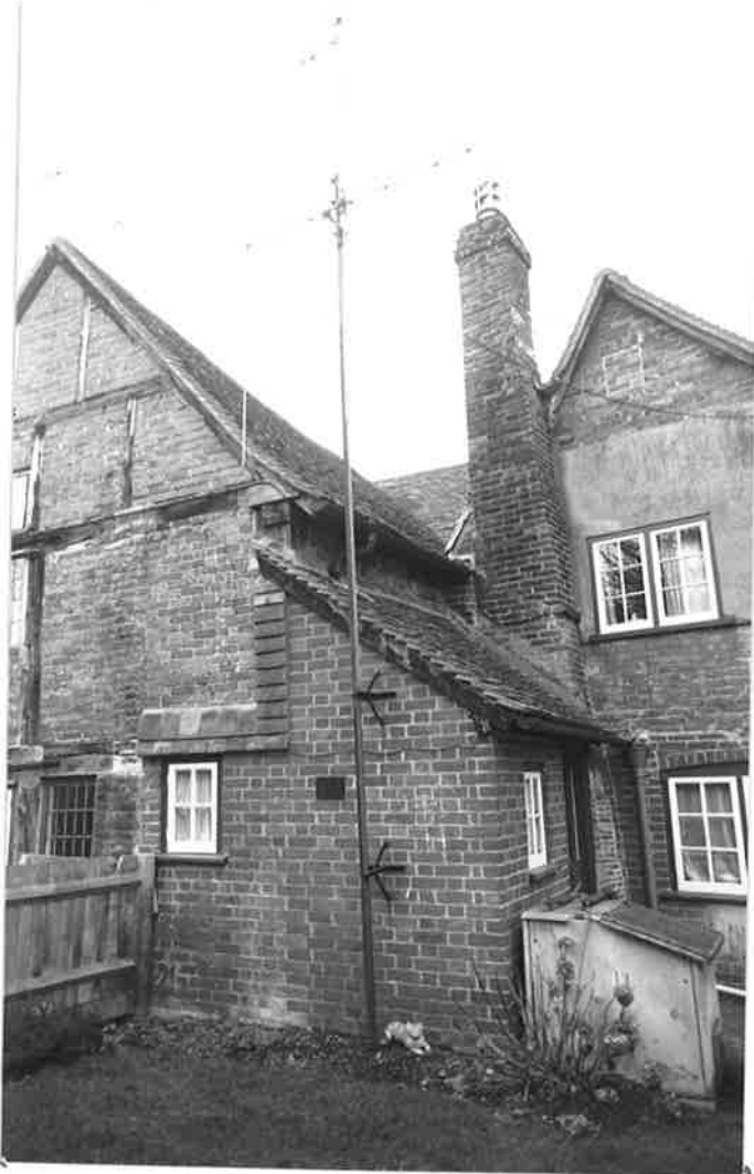
NOs 4 AND 5, WINGS K, AND N AND OUTSHUT M, VIEWED FROM SOUTH. R. 177 N 36.
