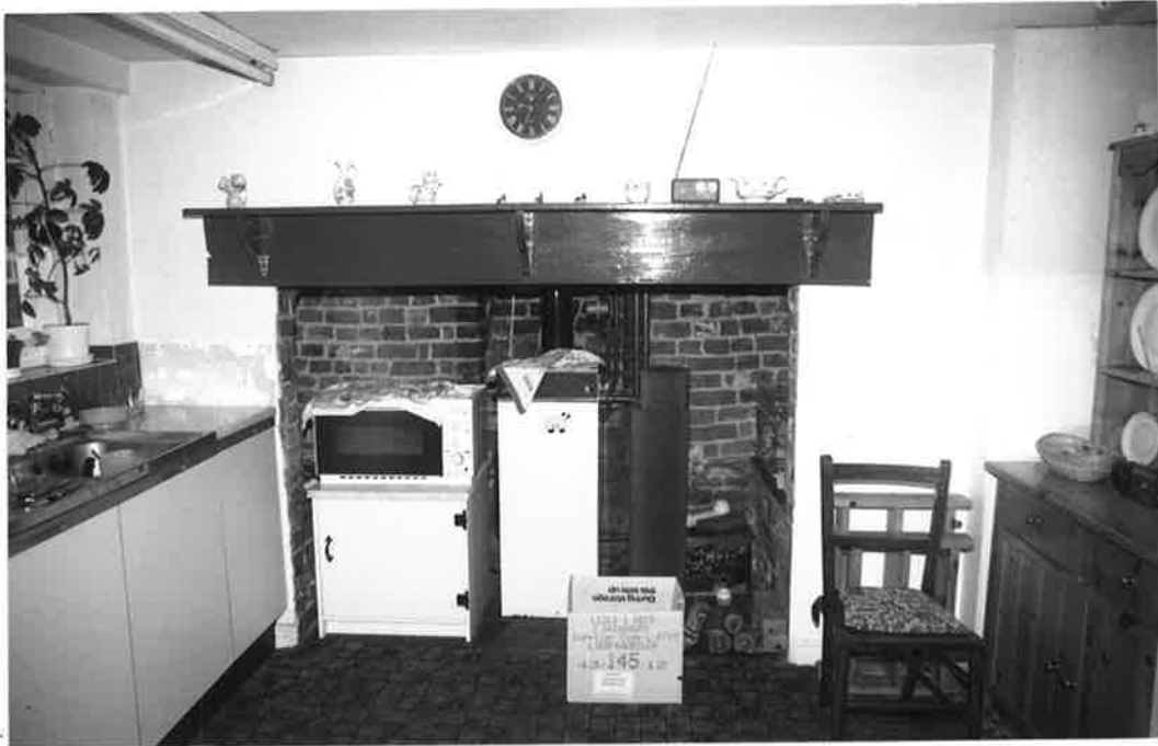
KITCHEN FIRE OPENING, ROOM A. R173 N31A.
