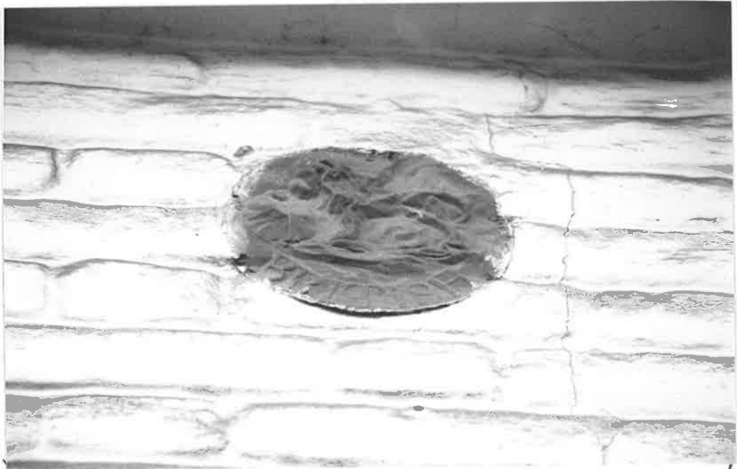
BRITISH FIRE OFFICE ASSURANCE PLATE, FRONT ELEVATION BLOCK L, Nº 7 R.175 N14.
