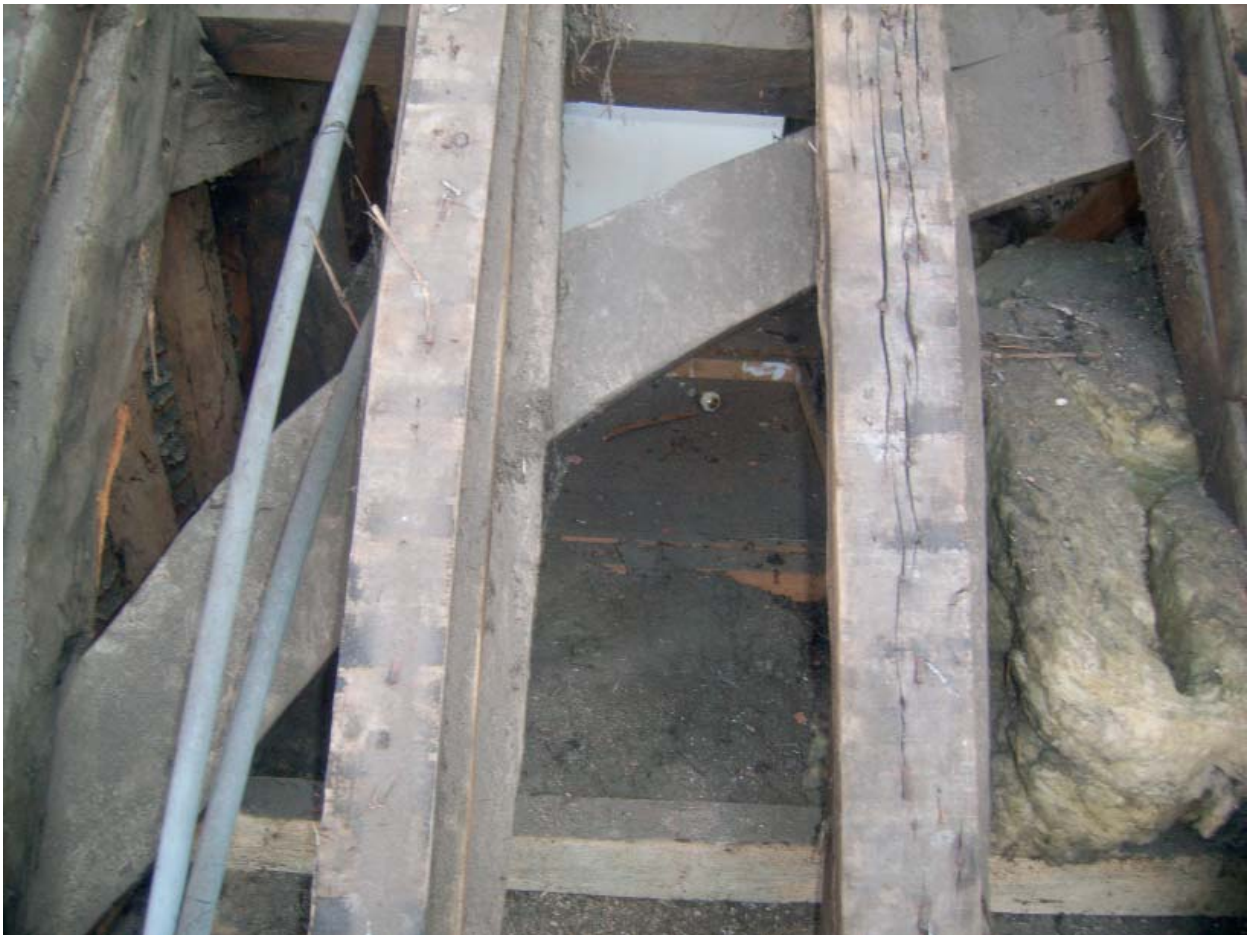
Plate 26: Curved windbrace in No.4 (Block R)
