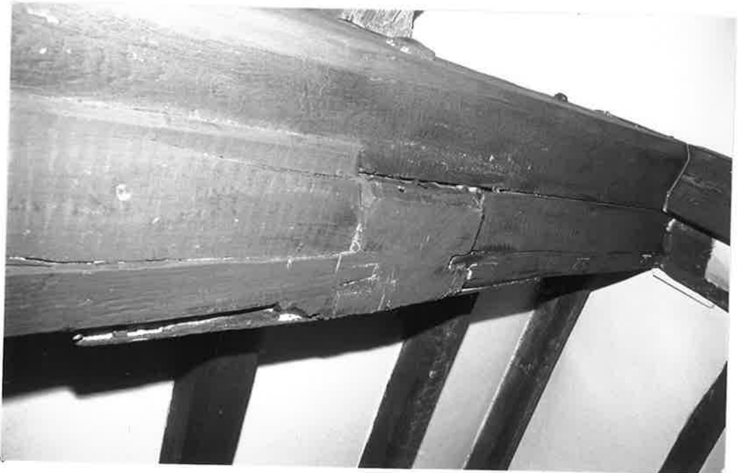
SOFFIT FACE OF BEAM DI, SHOWING ORIGINAL MAIN POST CUT THROUGH. R180 N31.
